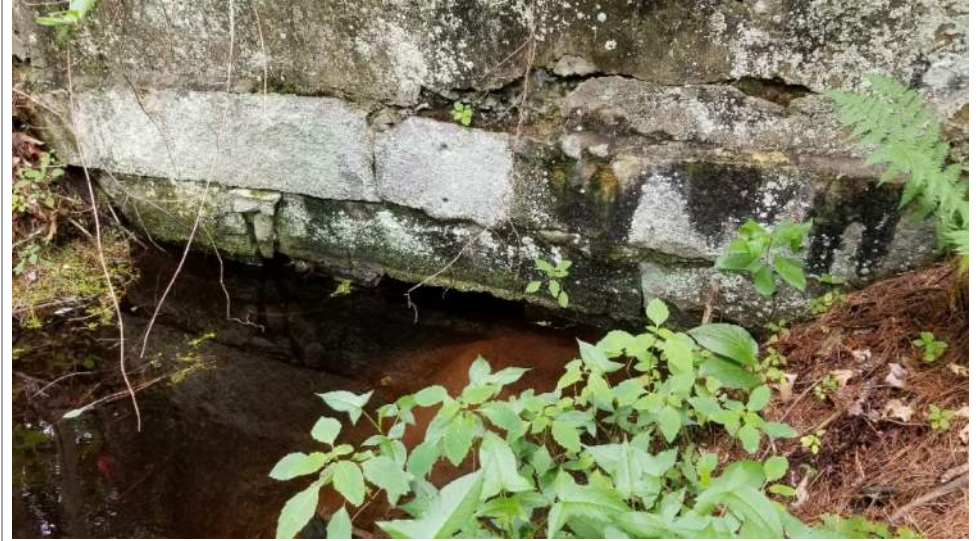
View of northern end of Structure 127G; most of culvert was submerged at time of the inspection
