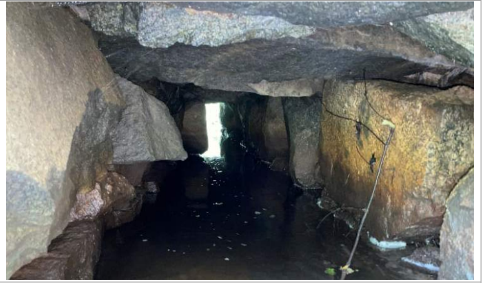
Looking through stone culvert from the north side to the south side
