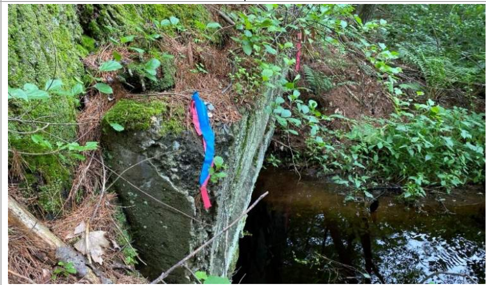
Headwall at northern end has shifted outward.
