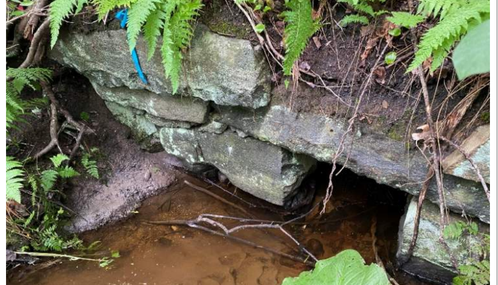
Bulging and missing stones at north headwall due to vegetation growth
