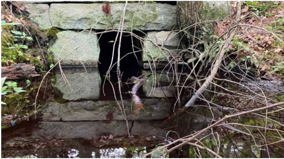
View of southern end of Structure 127G. Small window of daylight visible at northern end.
