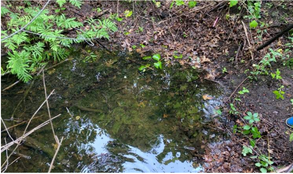
View near south end of culvert. Unable to locate inlet or outlet.
