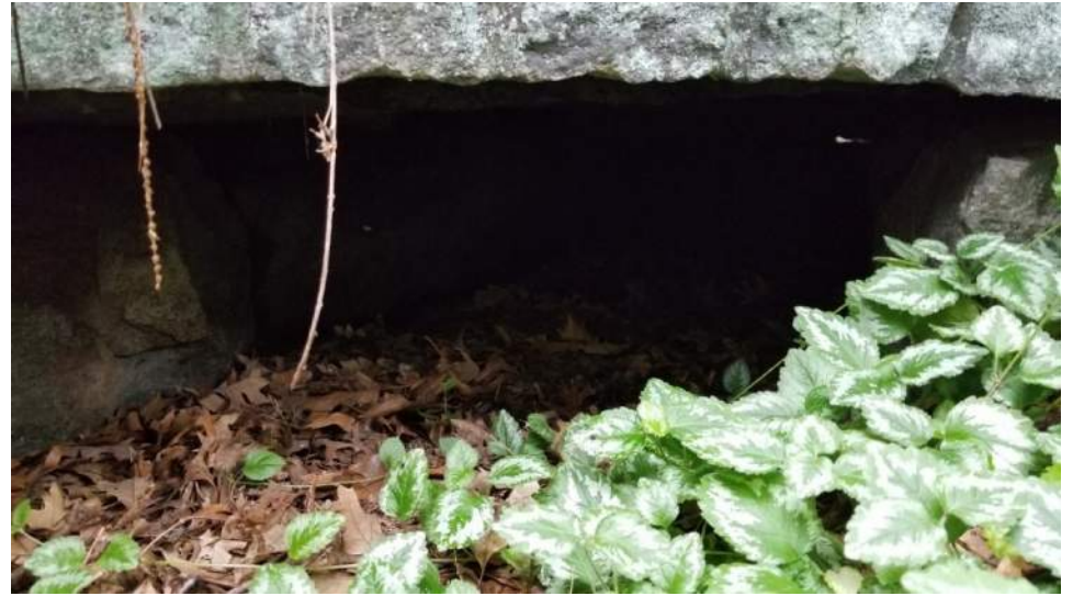
View through southern end of Structure 127H; light through the northern end is visible
