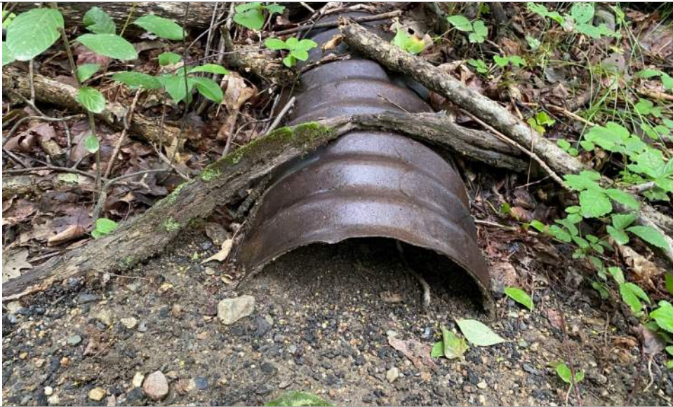
South end of culvert, partially filled with sediment. Sediment will be removed.
