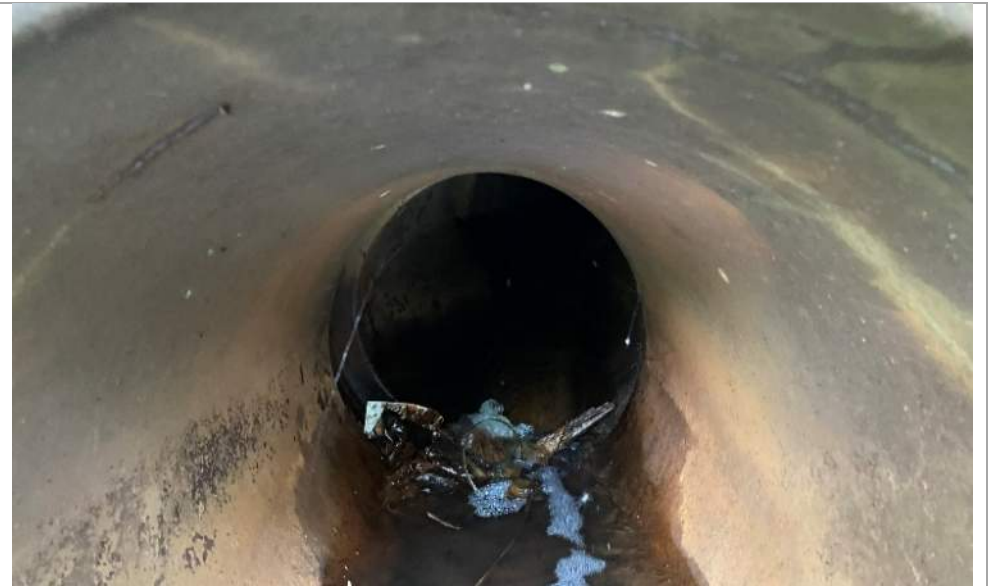
Looking through the pipe from the north side to the south side
