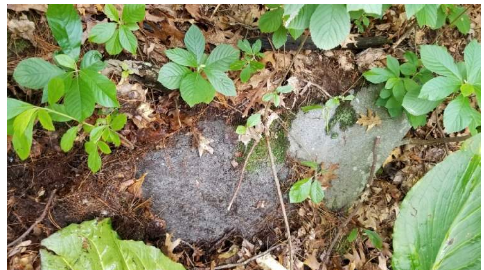
Possible portion of buried pipe and headwall of northern end of Structure 127J
