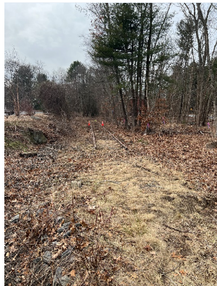
Photo 4: Near Sta. 175+00 looking south. Tree removal and low vegetation clearing was actively occurring in this area during the visit.
