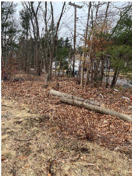
Photo 3: Near Sta. 175+00. Tree cutting and removal has begun to make space for the storage of future removed rail.
