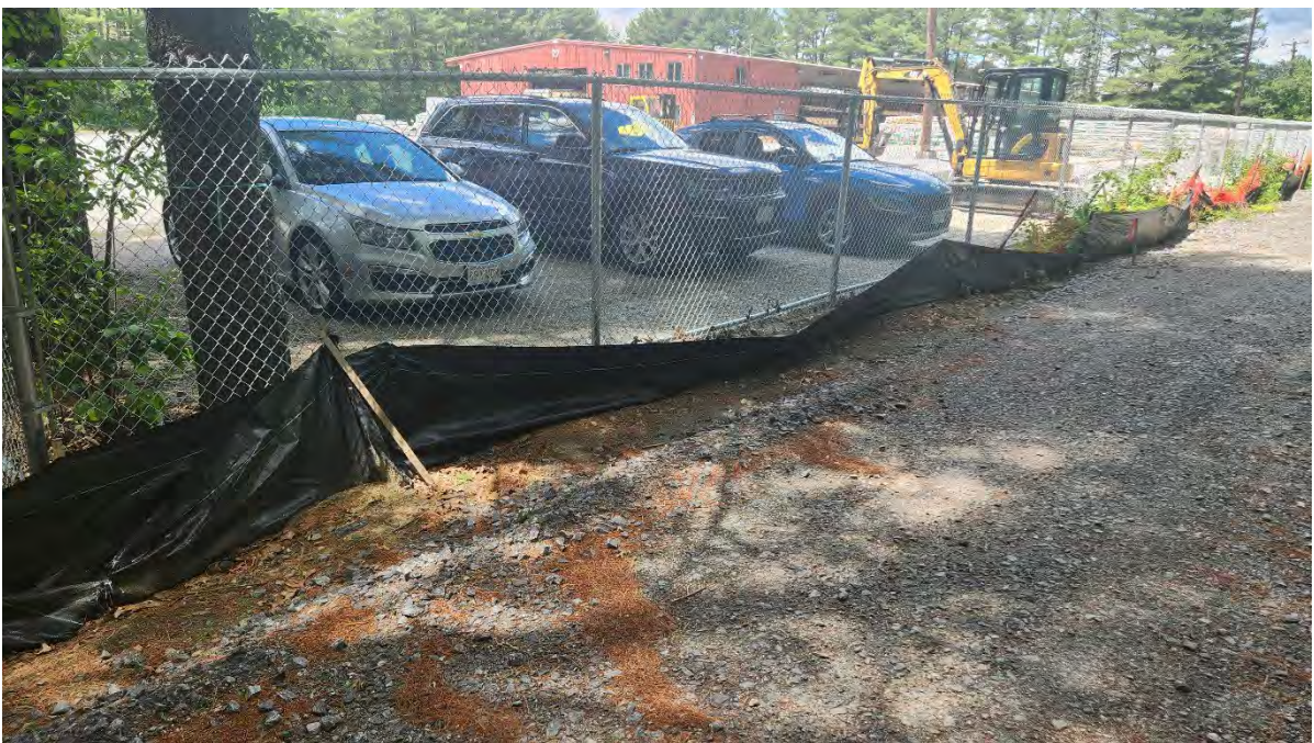
Photo 3: Broken stakes in silt fence along segment 11. Photo taken on 7/1/24
