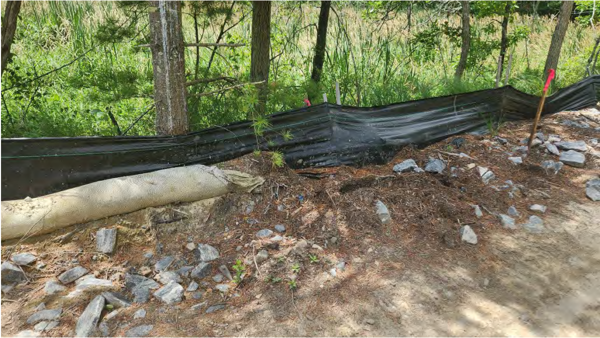
Photo 6: Filter tube is damaged and needs to be replaced in sections along segment 14. Photo taken on 7/1/24.
