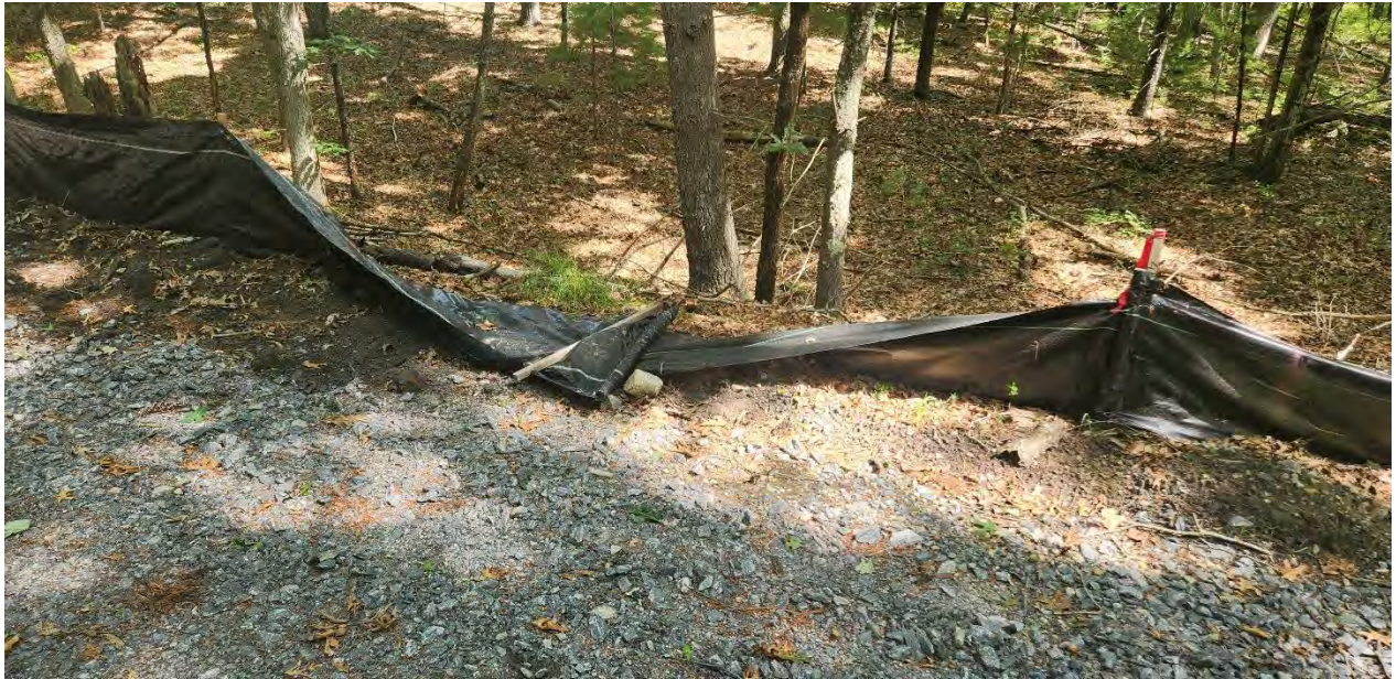
Photo 1: Broken stake in the silt fence along segment 8.
