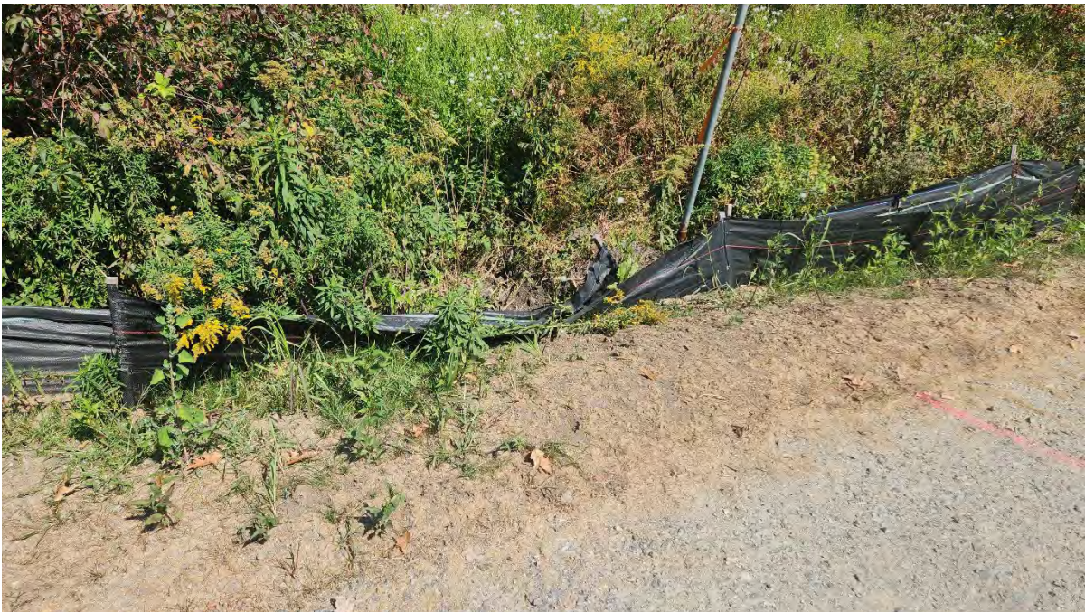
Photo 5: Silt fence ripped along segment 14. Photo taken on 9/16/24.
