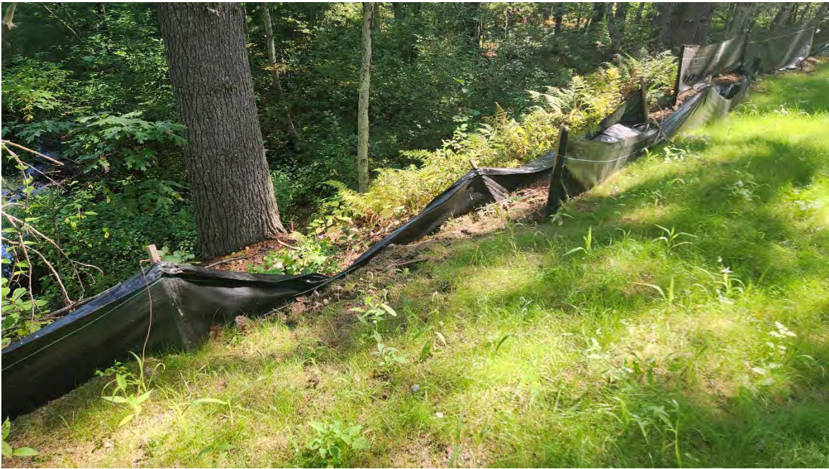
Photo 2: Broken stakes and sagging in the silt fence along segment 9. Photo taken on 9/16/24
