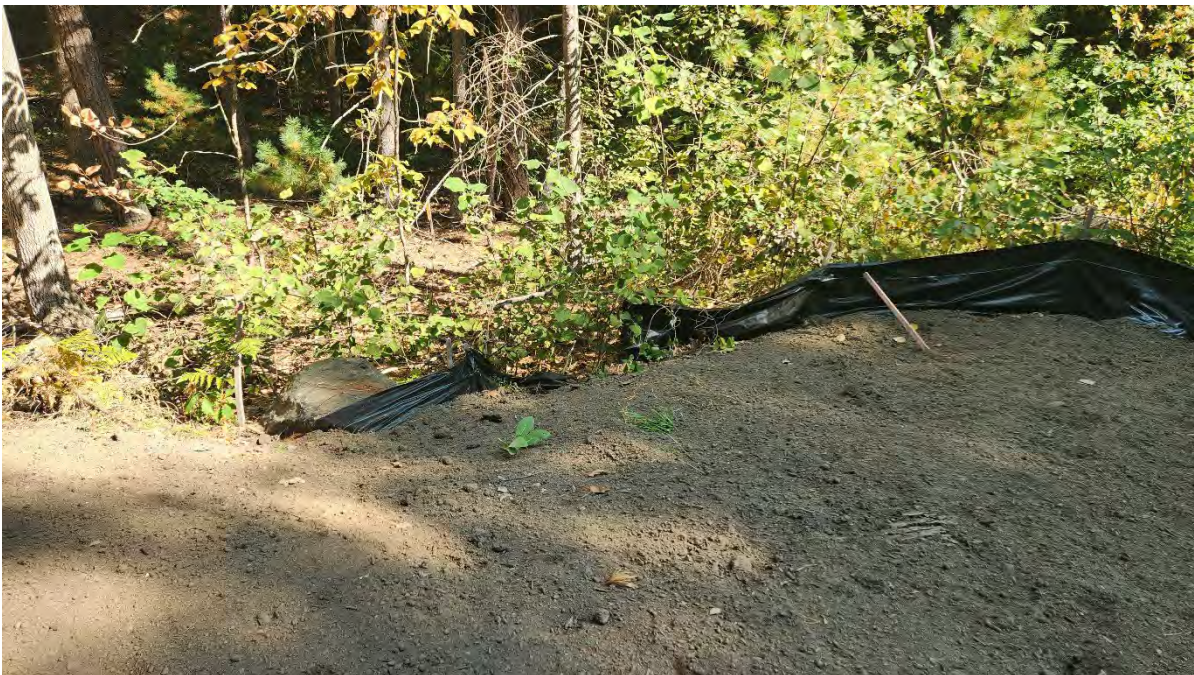
Photo 3: Broken stakes and ripping in the silt fence along segment 10. Photo taken on 9/16/24
