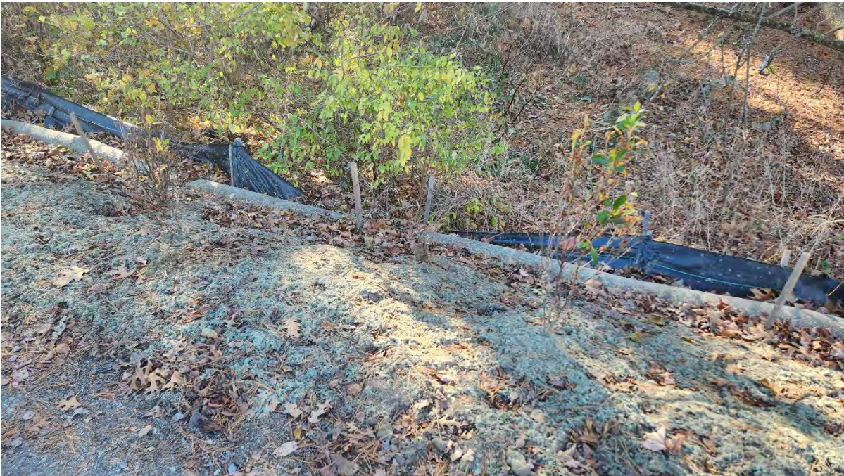
Photo 5: Rip in the silt fence along segment 13. Photo taken on 11/15/24.
