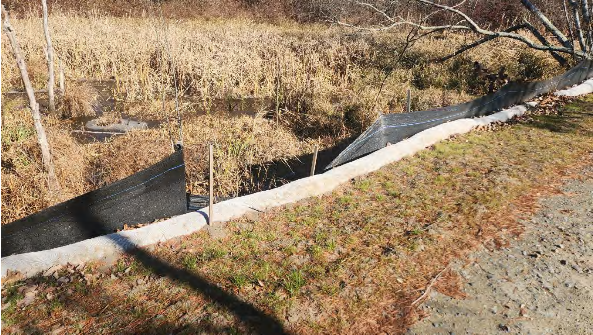
Photo 6: Rip in the silt fence along segment 14. Photo taken on 11/15/24.
