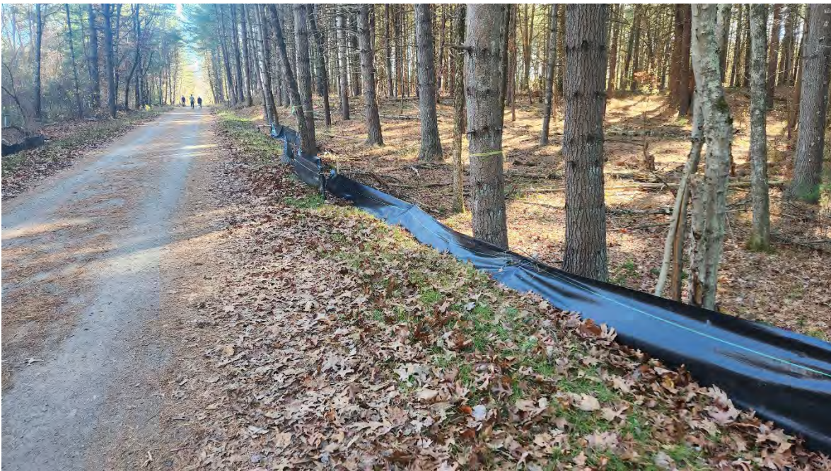
Photo 3: Broken stakes in the silt fence along segment 11. Photo taken on 11/15/24
