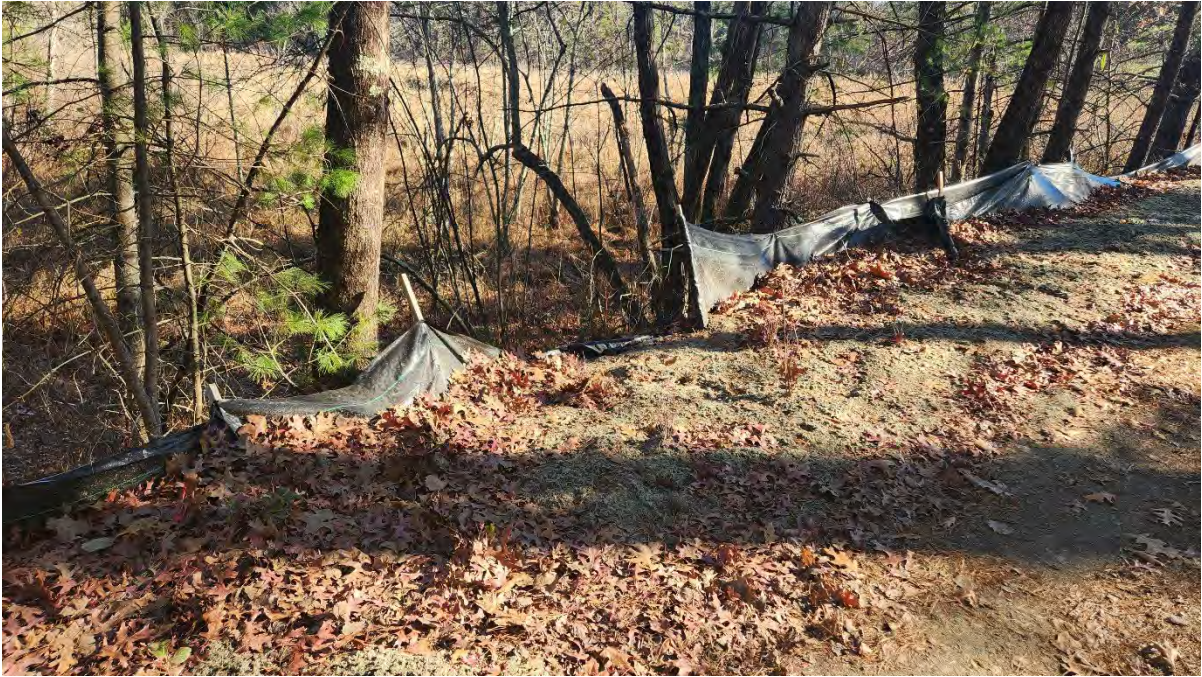
Photo 2: Rip in the silt fence along segment 7. Photo taken on 11/15/24
