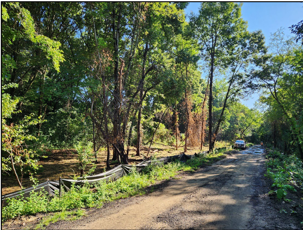
Photo 4. Mitigation area conditions at approximately STA 739+00 (Segment 14) facing northeast after invasive species management. Photos 3 and 4 show invasive management that was done using a mini excavator in 2023.
