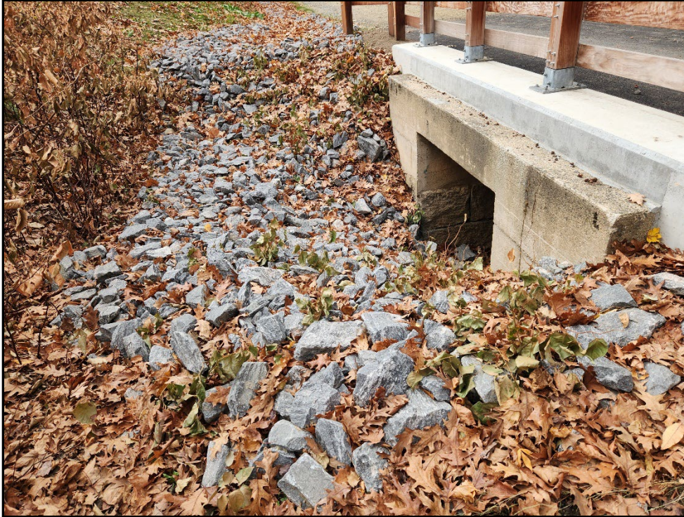
Photo 21. Japanese knotweed growing through rip rap near STA 119+50 in Segment 1. This photo was taken in fall of 2024.
