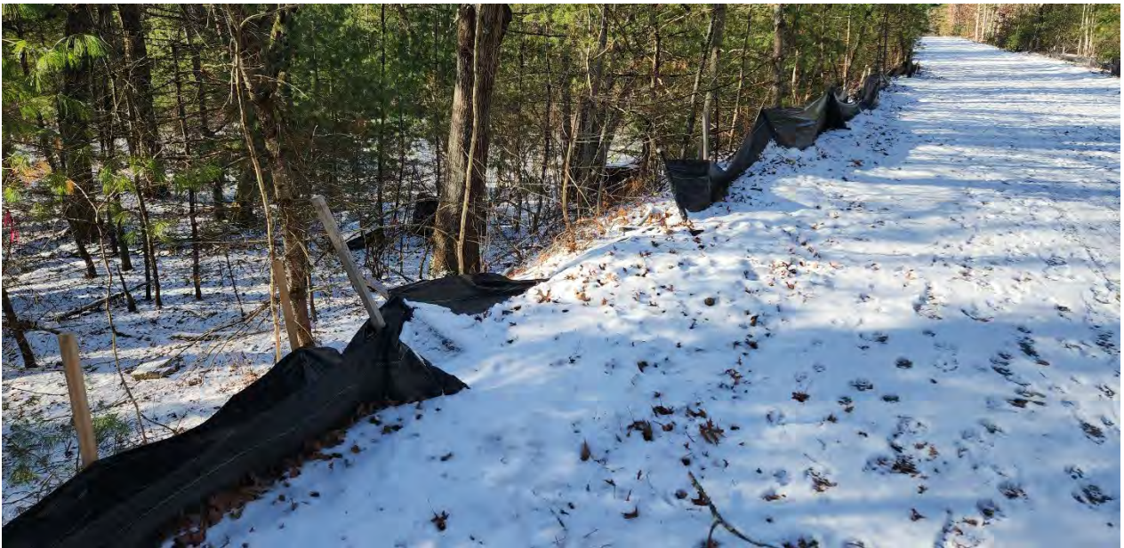
Photo 1: Broken stake in the silt fence along segment 7. Photo taken on 12/23/24
