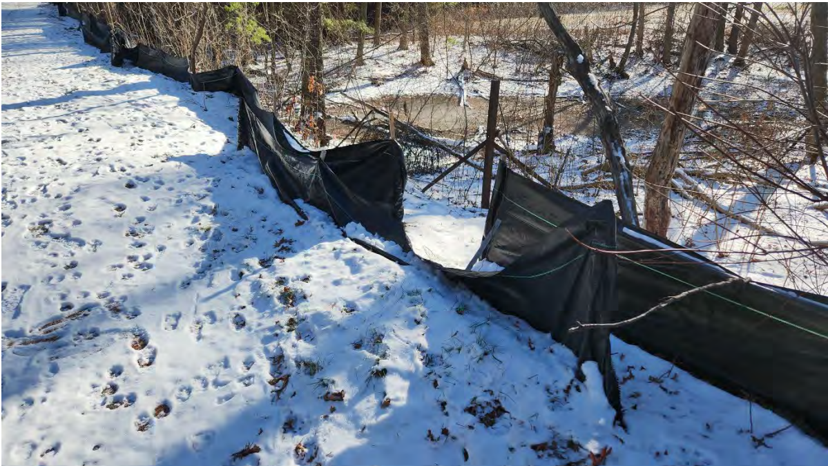
Photo 5: Rip in the silt fence along segment 11. Photo taken on 12/23/24.
