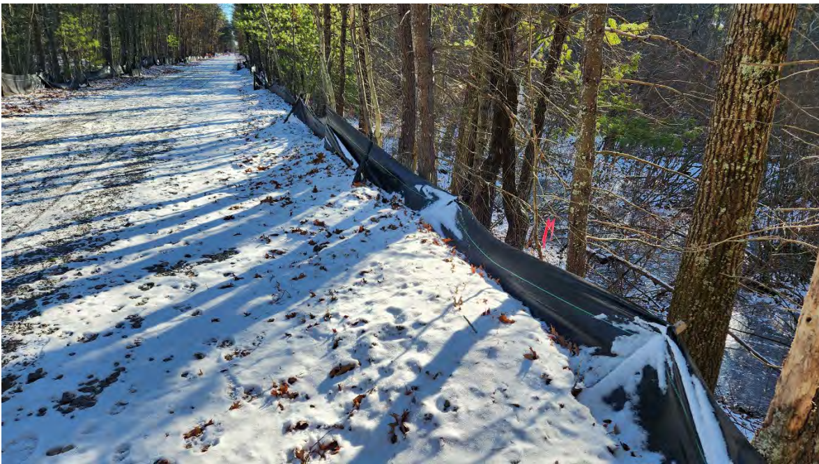
Photo 3: Broken stakes in the silt fence along segment 8. Photo taken on 12/23/24
