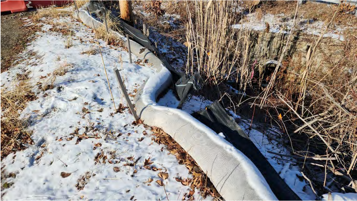
Photo 6: Rip in the silt fence along segment 12. Photo taken on 12/23/24.
