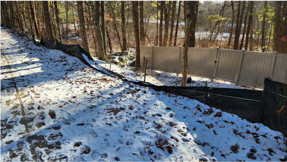
Photo 4: Rip in the silt fence along segment 10. Photo taken on 12/23/24
