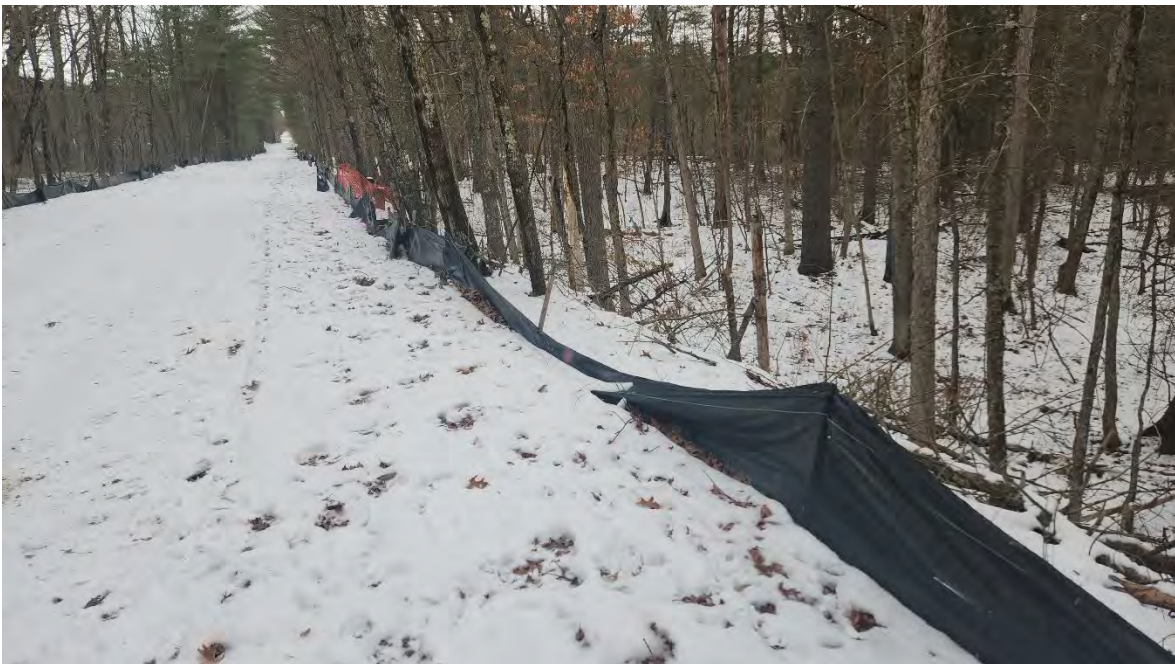
Photo 3: Silt fence is ripped from stake along segment 8. Photo taken on 1/28/25
