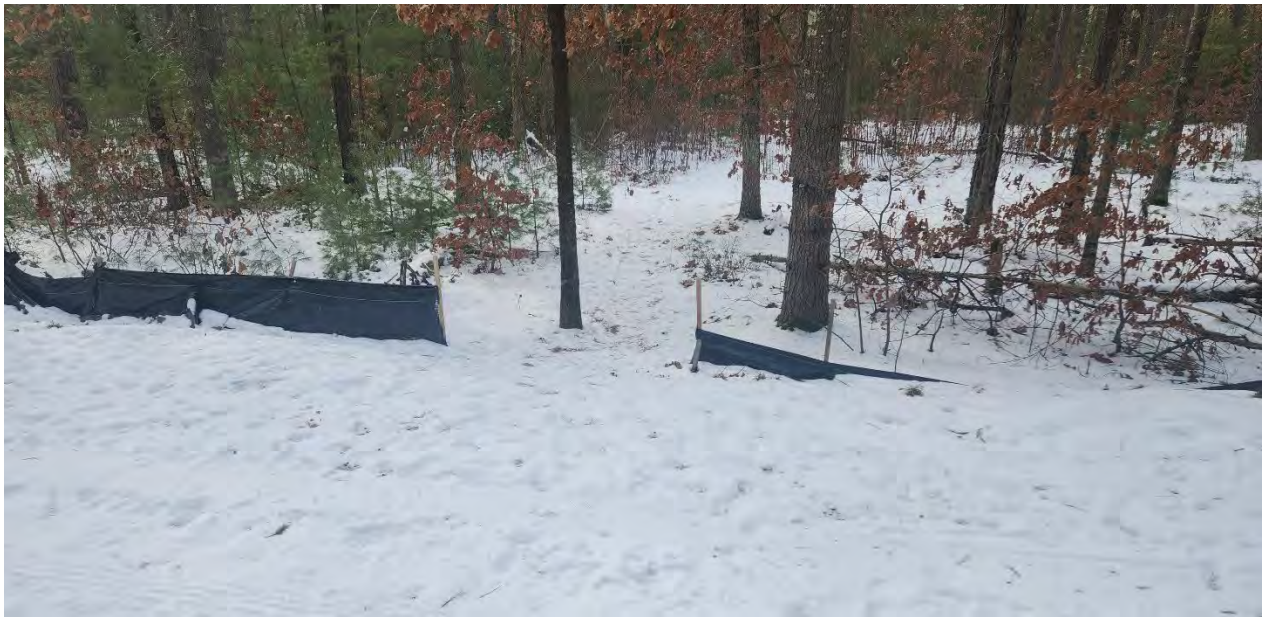
Photo 1: Rip in the silt fence at a trail connection along segment 7. Photo taken on 1/28/25
