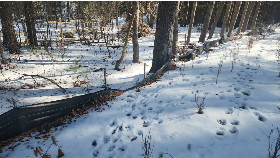
Photo 4: Silt fence is ripped from stake along segment 9. Photo taken on 1/28/25
