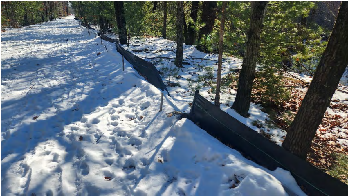
Photo 5: Rip in the silt fence along segment 11. Photo taken on 1/28/25.
