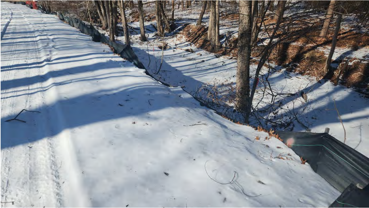
Photo 6: Broken Stake in the silt fence along segment 14. Photo taken on 1/28/25.
