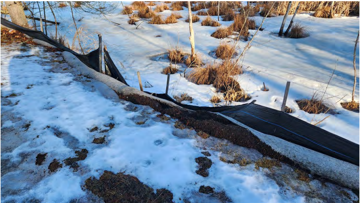
Photo 7: Broken stakes in the silt fence and damaged filter tube along segment 14. Photo taken on 2/28/25.
