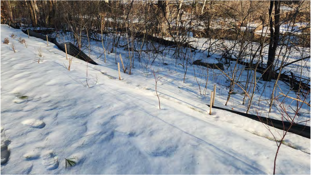
Photo 6: Rip in the silt fence along segment 13. Photo taken on 2/28/25.
