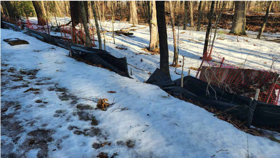
Photo 4: Rip in the silt fence along segment 11. Photo taken on 2/28/25
