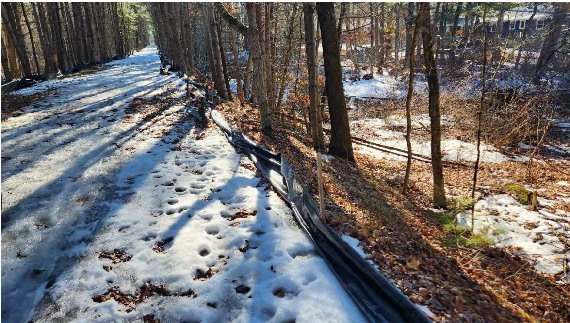
Photo 3: Significant ripping in the silt fence along segment 10. Photo taken on 2/28/25
