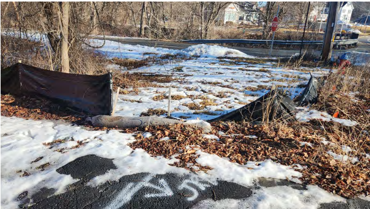
Photo 5: Rip in the silt fence along segment 12. Photo taken on 2/28/25.
