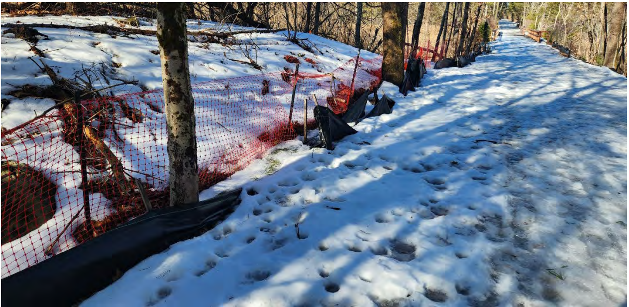
Photo 1: Ripping and broken stakes in the silt fence along segment 8. Photo taken on 2/28/25
