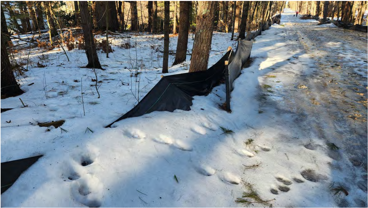
Photo 2: Broken stake in the silt fence along segment 9. Photo taken on 2/28/25
