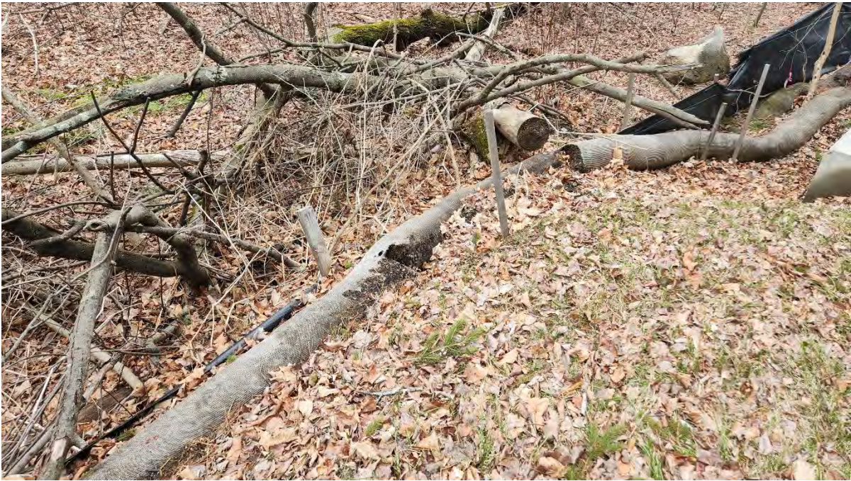
Photo 6: Rip in the silt fence and damaged filter tube along segment 13. Photo taken on 3/31/25.
