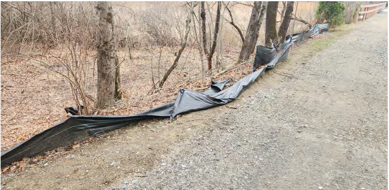
Photo 1: Ripping and broken stakes in the silt fence along segment 8. Photo taken on 3/31/25
