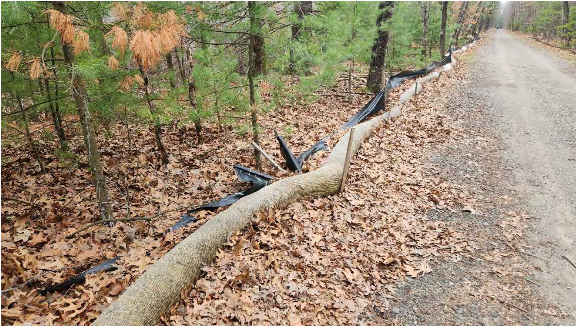
Photo 4: Rip in the silt fence along segment 11. Photo taken on 3/31/25
