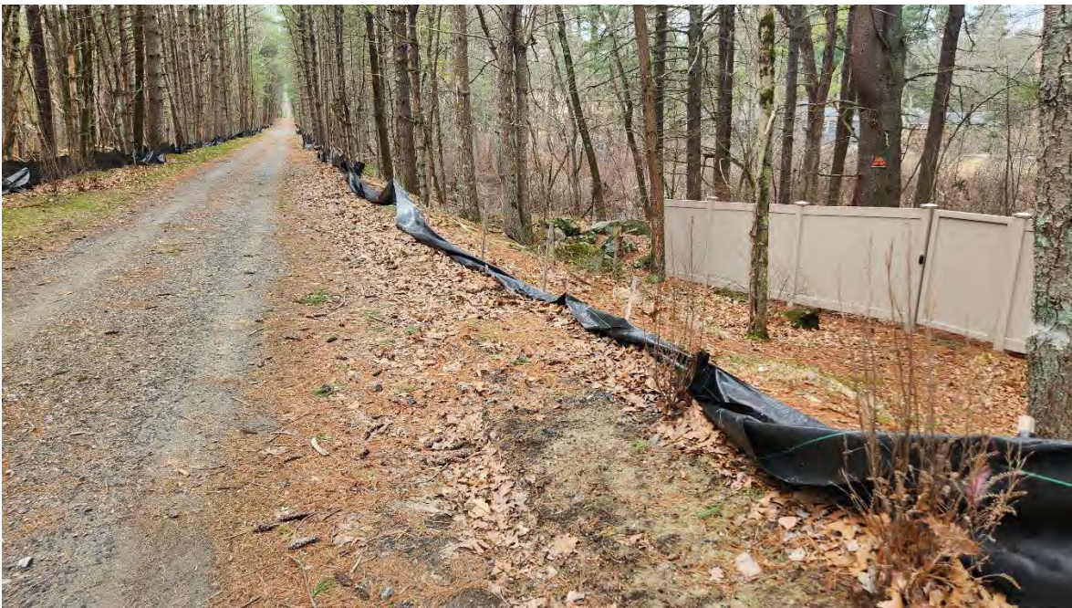
Photo 3: Significant ripping in the silt fence along segment 10. Photo taken on 3/31/25
