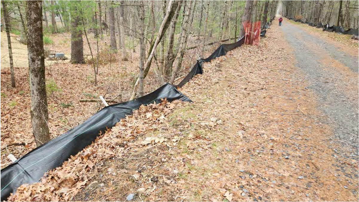
Photo 2: Broken stakes in the silt fence along segment 9. Photo taken on 3/31/25
