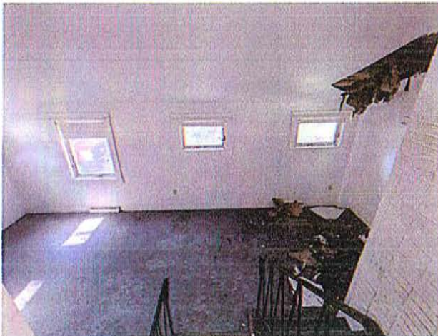
21 Great Lakes in currently inhabitable due to ceiling damage.
