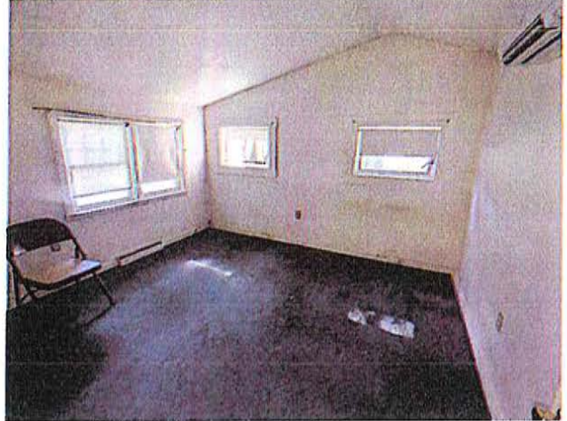
The carpet and interiors need replacement.
