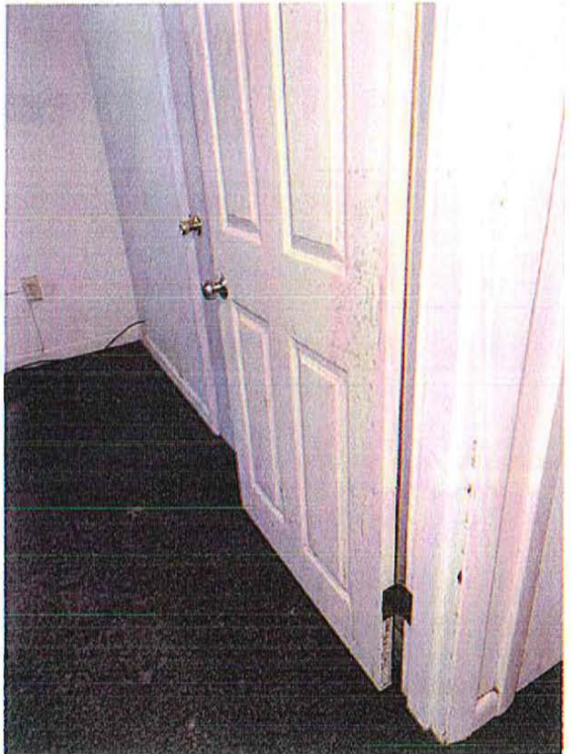
A bedroom door needs replacement.
