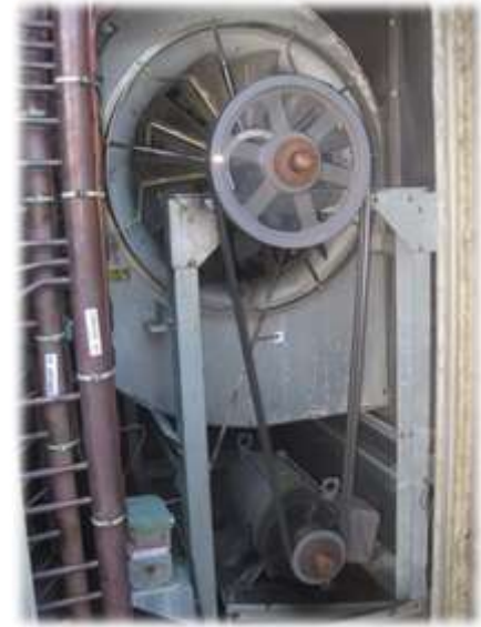
Figure 7.1: Existing belt driven fan with inlet guide vanes inside RTU-1.
