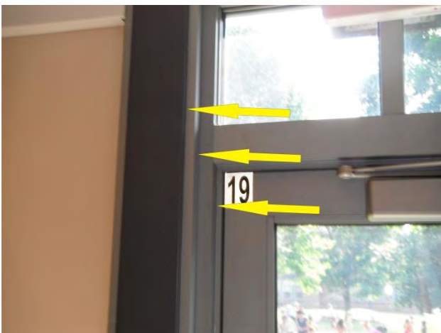
Doors – arrows point to locations of missing sealant and air leakage pathways at the perimeter casing of the door system.
