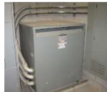
Figure 29.1: Existing standard efficiency transformers like the one pictured above at the Curtis Middle School will be replaced in this measure.
