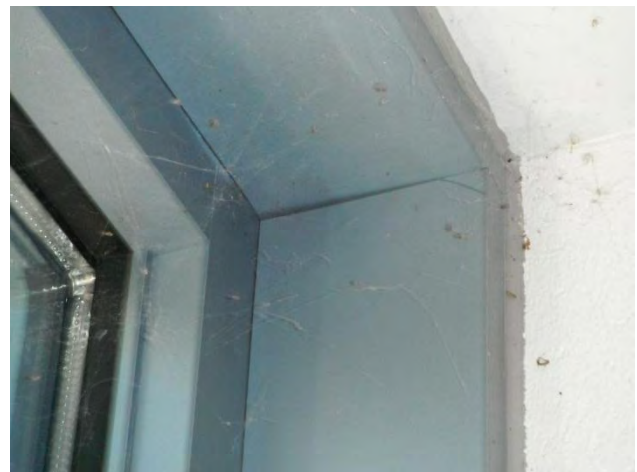
Doors – gaps at the perimeter casing where sealant was not installed. Accumulation of cob webs is an indicator of excessive air leakage.
