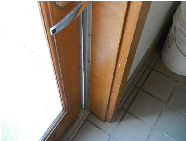
Doors – daylight shining through the separation between the existing weather stripping and the door identifies an air leakage pathway.
