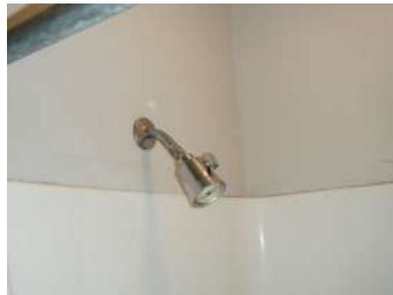
Figure 25.1: Standard flow showerhead fixtures like the one shown above at the Fire Department Headquarters will be replaced with low consumption models in this measure.
