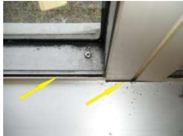
Figure 11.1: By reducing building infiltration through leaky windows, energy savings will be achieved through reduced heating and cooling loads. Shown above is a single pane window at the Fairbank Community Center.
