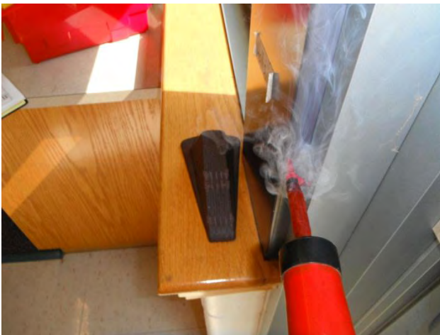
Doors – air leakage shown by smoke tracer testing at the perimeter casing of the door system.
