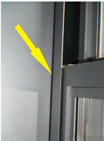
Windows – sealant missing at gap between the window frame and the stop.
