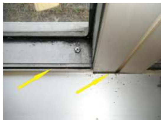
Figure 11.1: By reducing infiltration through leaky windows at the Fairbank Community Center, energy savings will be achieved through reduced heating and cooling loads.
