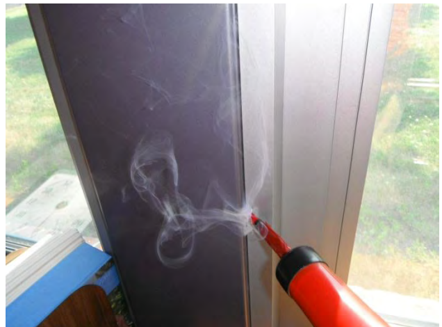
Windows – air leakage shown by smoke tracer testing at window casing-wall joint.
