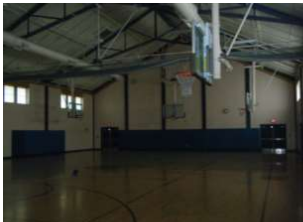
Figure 6.1: Existing constant air volume system serving the gymnasium at the Haynes Elementary School.
