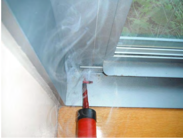
Windows – air leakage shown by smoke tracer testing at window stop-frame joint.
