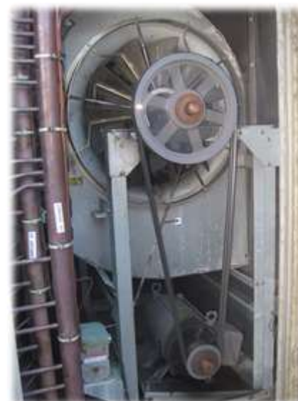
Figure 7.1: Existing belt driven fan with inlet guide vanes inside RTU-1.
