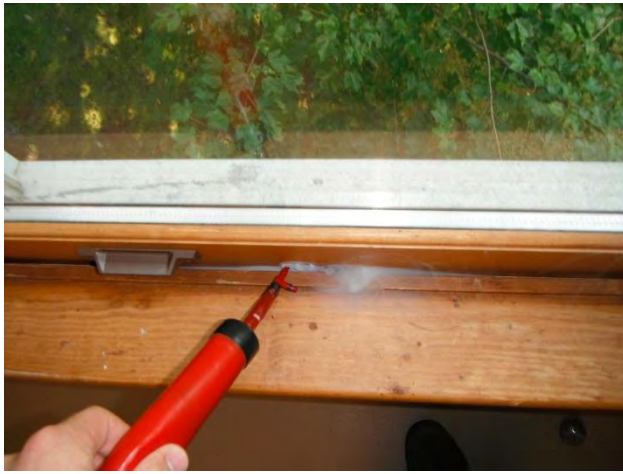
Windows – air leakage shown by smoke tracer testing at the bottom of the lower sash of the double hung window.
