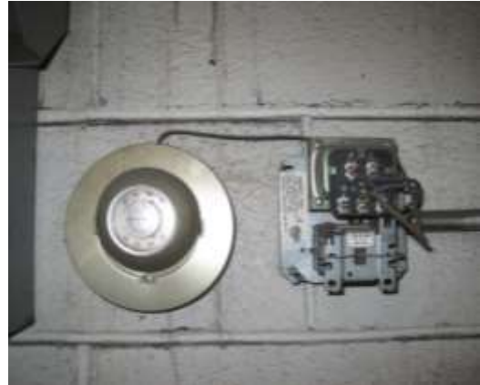
Figure 4.1: Ameresco proposes to replace the existing T87 thermostats at the DPW Highway Building with new programmable thermostats.
