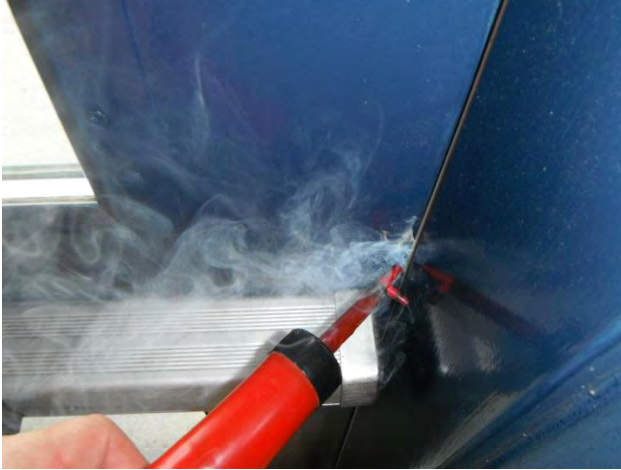
Doors – air leakage shown by smoke tracer testing at double door system.
