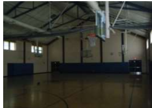
Figure 6.1: Existing constant air volume system serving the gymnasium at the Haynes Elementary School.
