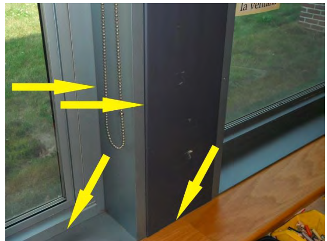
Doors – arrows point to locations of missing sealant and air leakage pathways at the perimeter casing of the window system.
