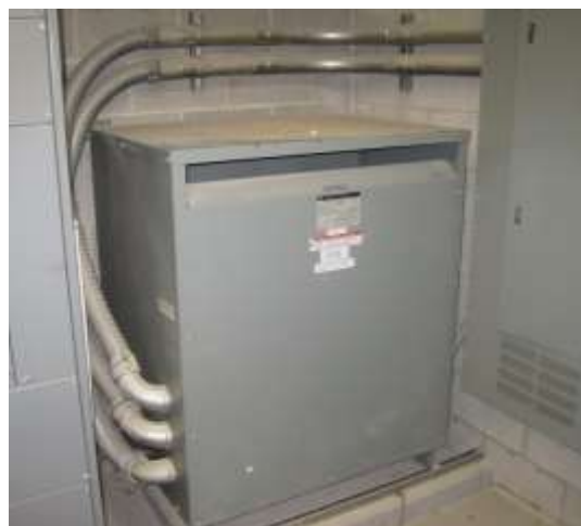
Figure 29.1: Existing standard efficiency transformers like the one pictured above at the Curtis Middle School will be replaced in this measure.
