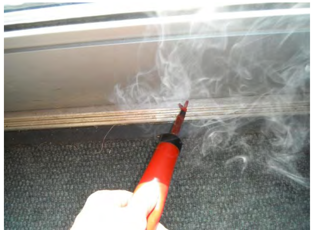
Doors – air leakage shown at single door system at the base of the door.
