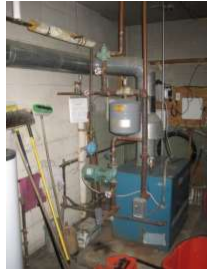
Figure 22.1: Existing bare pipe at Fire Station North and Fire Station South will be insulated.
