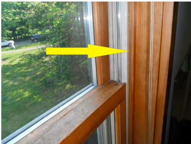
Windows – arrow points to the vertical joint between the compression jamb and the window stop where sealant was never installed.
