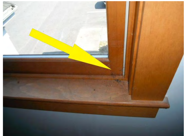
Windows – cob webs and dust accumulation at the bottom of the lower sash is an indicator of unwanted air leakage.
