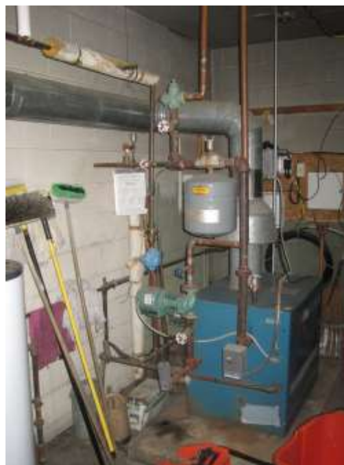
Figure 22.1: Existing bare pipe at Fire Station North and Fire Station South will be insulated. Pictured above is the boiler at Fire Station North.
