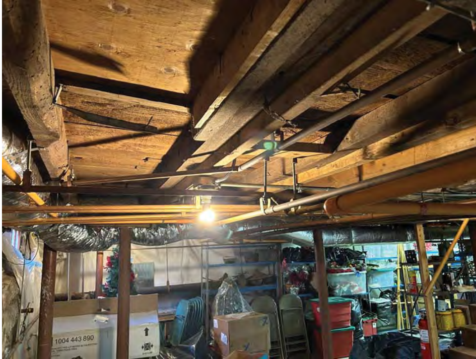
Figure 8.2-5 Sistered framing in central bay.
