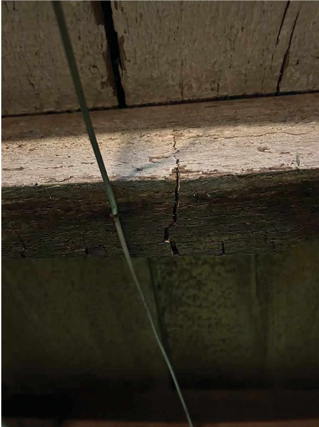
Figure 8.3-13 Cracked joist below parlor.
