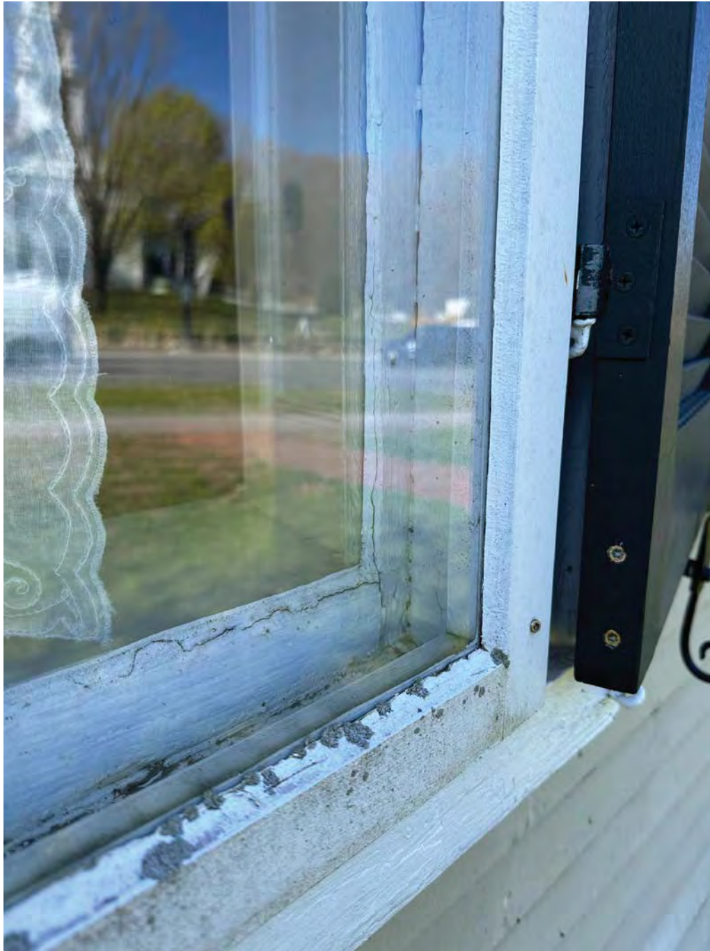
Figure 4.4-12 The perimeter sealant and glazing putty around the windows appear deteriorated, with cracks and gaps in some locations, leading to poor performance.
