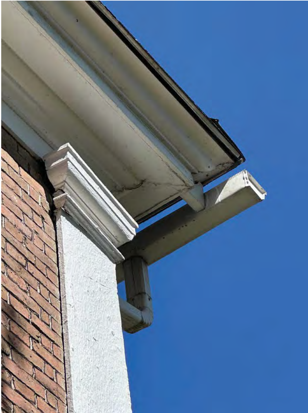
Figure 4.7-3 Along the north elevation, a gutter was installed along the roofline, supported by wood blocking.
