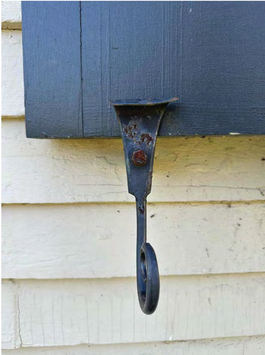
Figure 4.5-5 Less typical conditions found were that the shutters have been loosely anchored to the building, and many of the tiebacks are loosely installed and are rusting.
