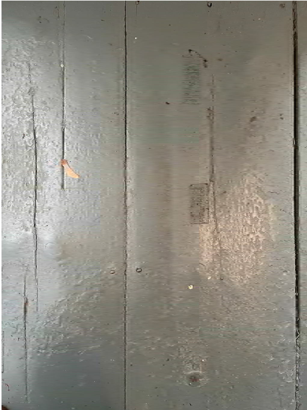
Figure 4.11-2 Floorboards vary in width, and are painted a dusty blue. Signs of cracking and paint loss were observed.
