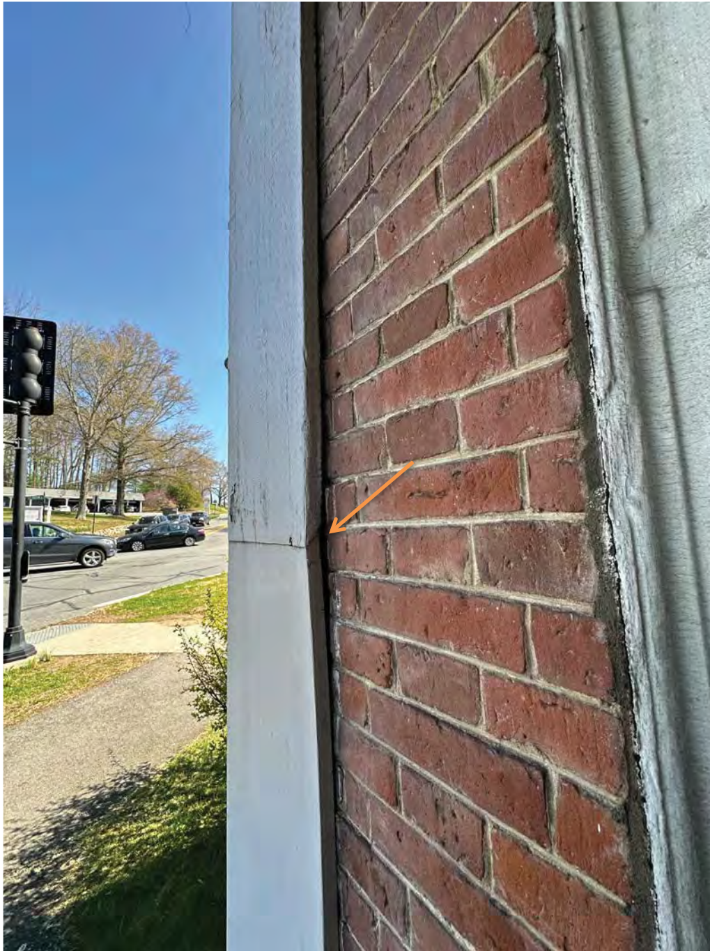
Figure 4.1-14 The pilasters are separating from the brick walls causing gaps between the materials.
