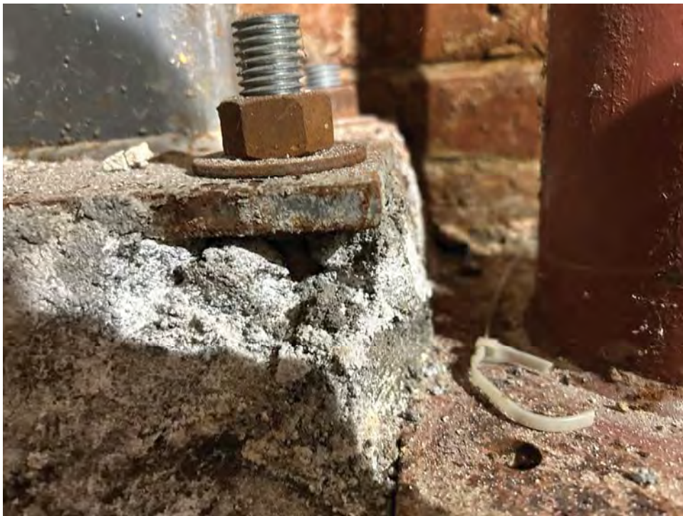
Figure 8.3-2 Spalled grout at HSS post anchorage.
