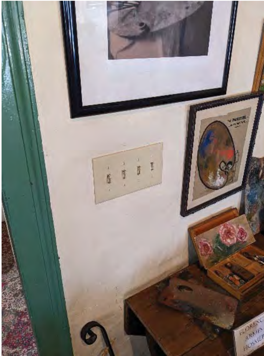
Figure 9.8-2 Outdated lighting controls.
