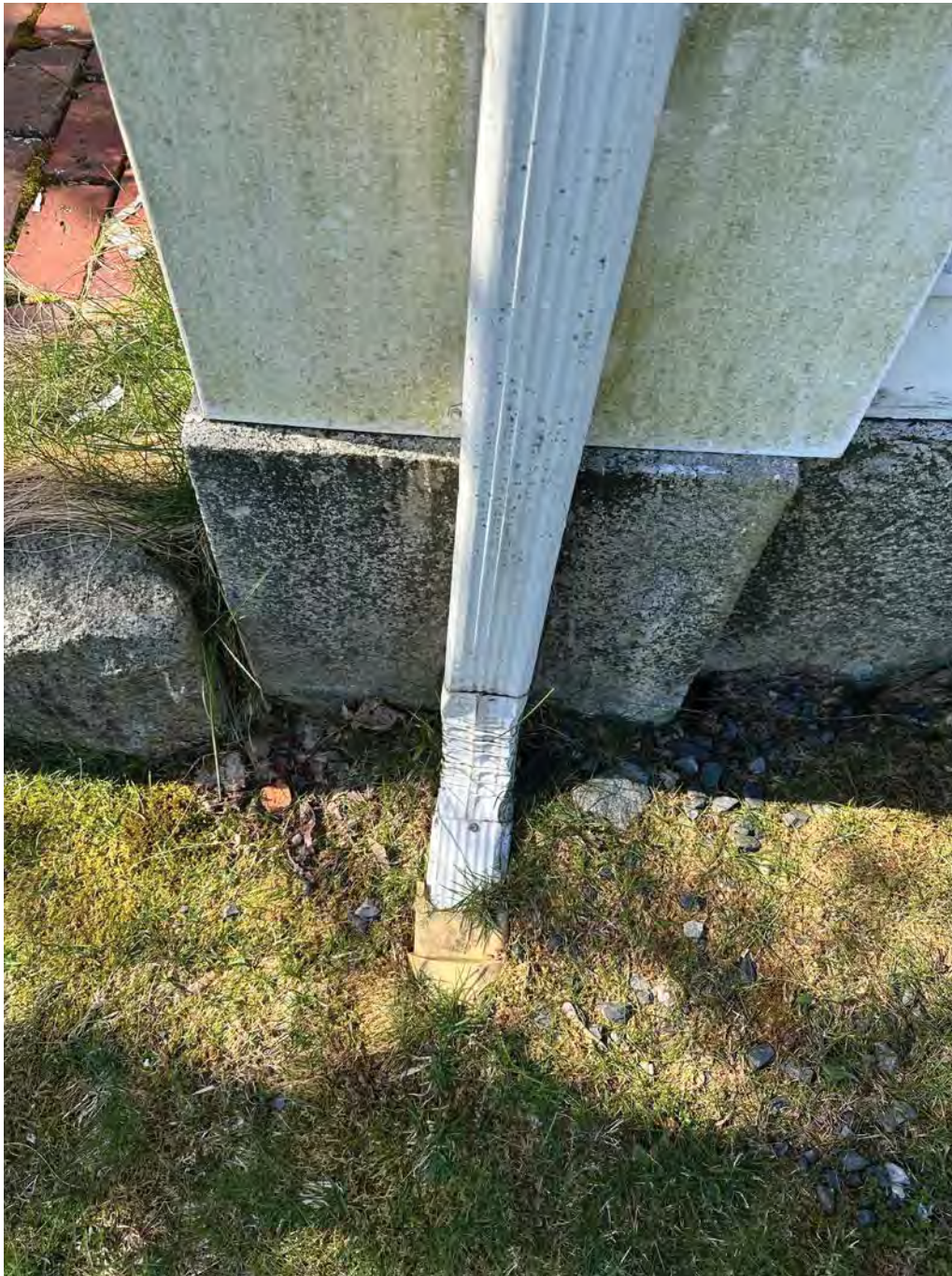
Figure 4.3-5 There is no evident base flashing between the wood pilaster and the granite foundation.
