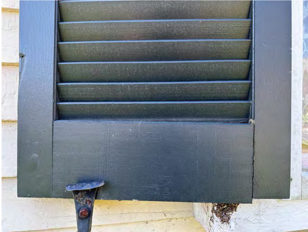
Figure 4.5-1 Loose bottom rail of a shutter. Typical conditions seen throughout.
