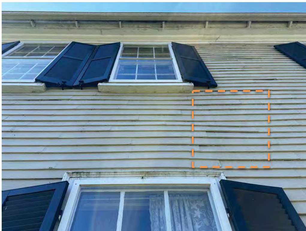
Figure 4.1-5 Depression in the clapboard, approximately 4 square feet in size.
