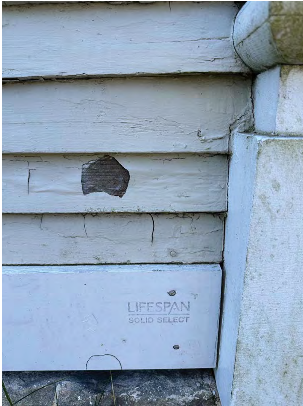
Figure 4.1-6 Blistering paint on butt-beveled clapboard.
