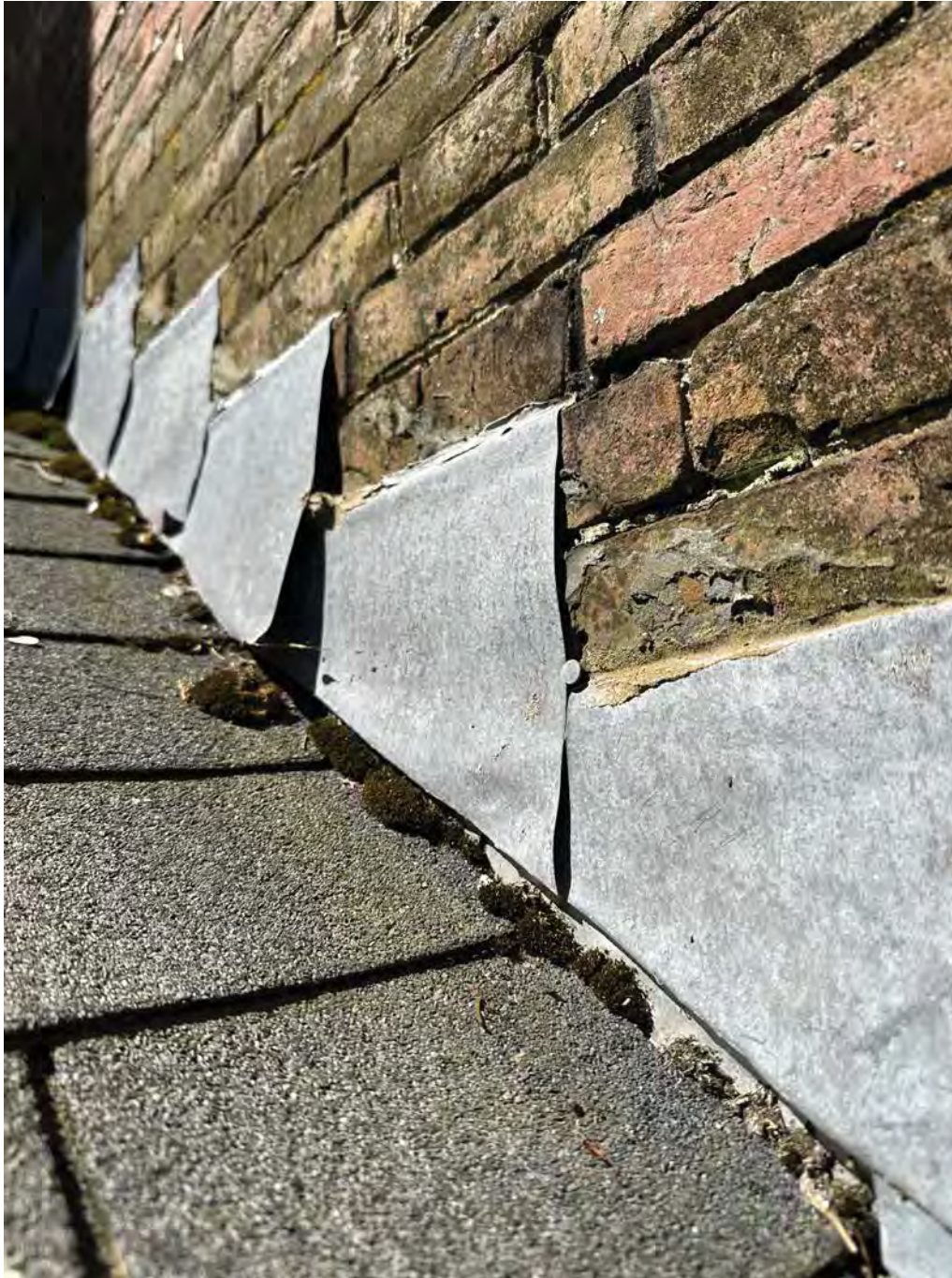
Figure 4.6-12 The step-flashing at the building joint of the north-facing slope along the east elevation of the house is in need of replacement. Portions have become unattached from the brick wall and roof, and are deflected in many places.
