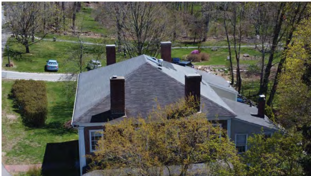
Figure 4.6-7 Along the west slope, there are signs of water damage seen in the form of discoloration, evident near the chimneys.
