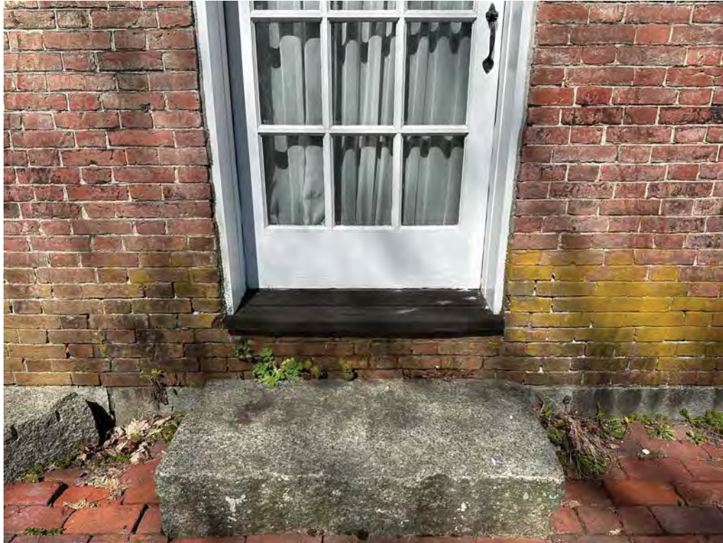
Figure 4.4-9 Door and sill on D-12 and D-06 were found to be damaged, cupped, and pitched backward.
