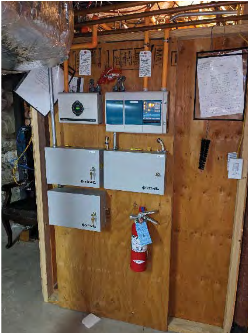
Figure 9.9-2 VESDA early warning smoke detection system.
