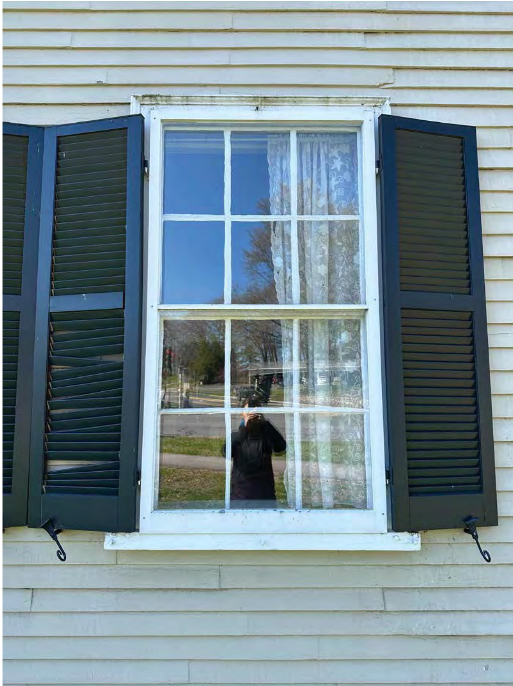
Figure 4.4-10 The storm windows are non-operable and are screwed to the wood casing. One storm window on the north façade (W-05) was installed upside down.
