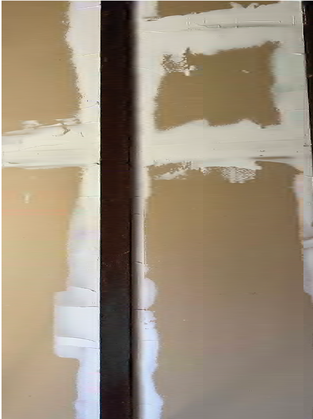
Figure 4.10-22 Southern and western walls of S-05. Drywall and timber framing with no finish material or paint.
