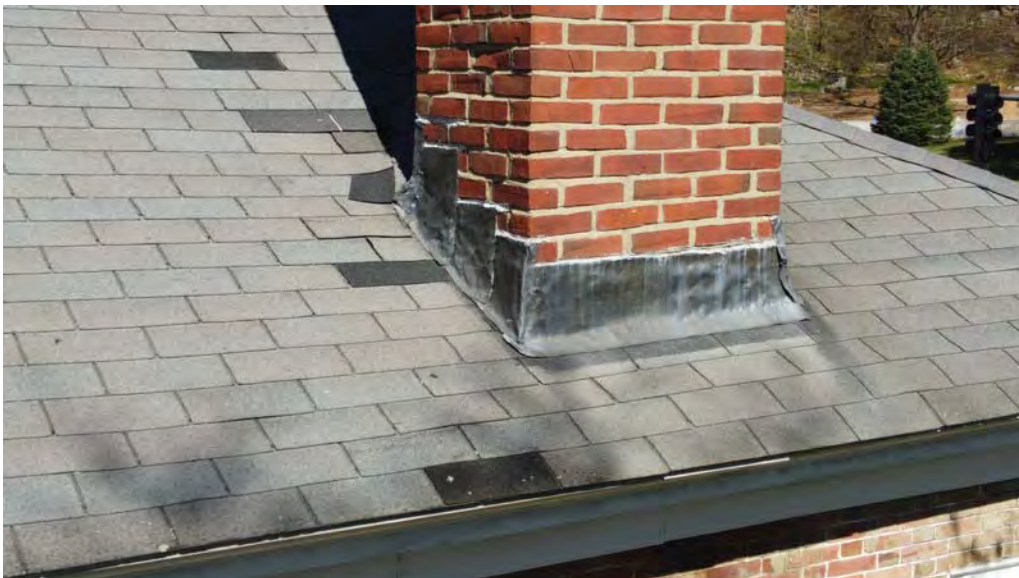
Figure 4.6-3 The step-flashing around the chimneystacks and crickets are in poor condition due to general end-of-life degradation as sections of the flashing are upturned and have become detached from the finished roof surface, or itself.
