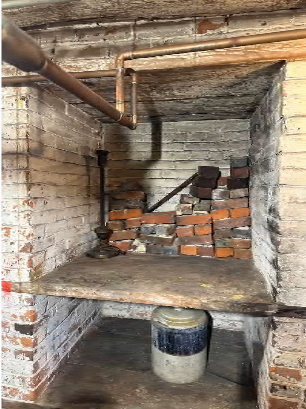
Figure 4.12-2 Fireplaces FP-05 and FP-09, and FP-06 and FP-10 each share a chimneystack with two flutes, with foundations and footings visible in the basement. Visible are cracked bricks, and loss of masonry coating.
