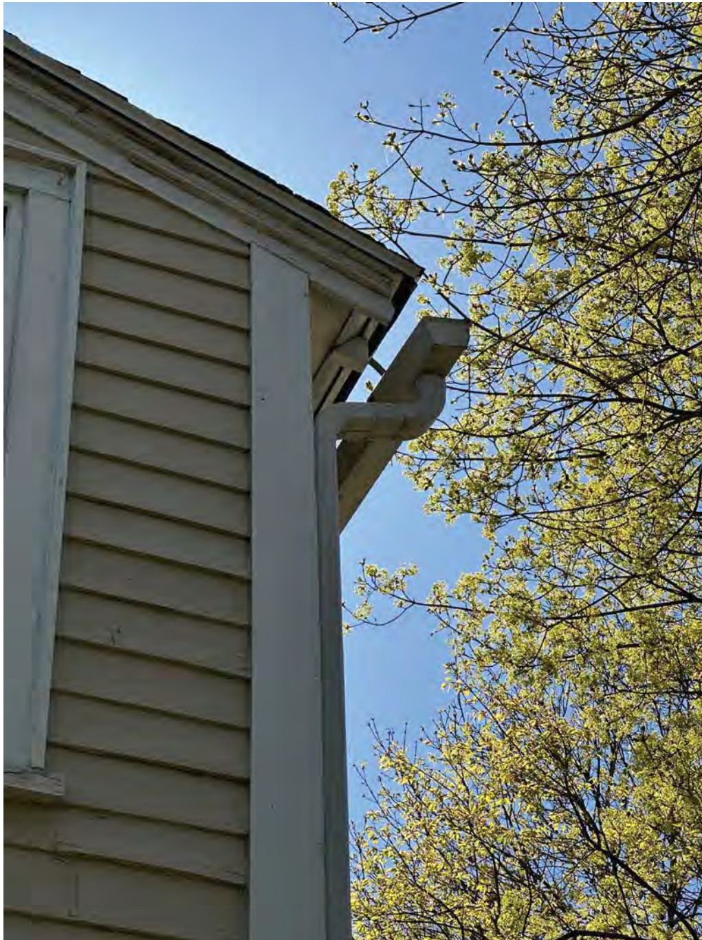
Figure 4.7-7 This gutter is fastened to the roof rafter at the southeast corner with a spike-and-ferrule, while the remaining length of gutter is fastened using strap hangers, which were installed atop the roof membrane, rather than below.
