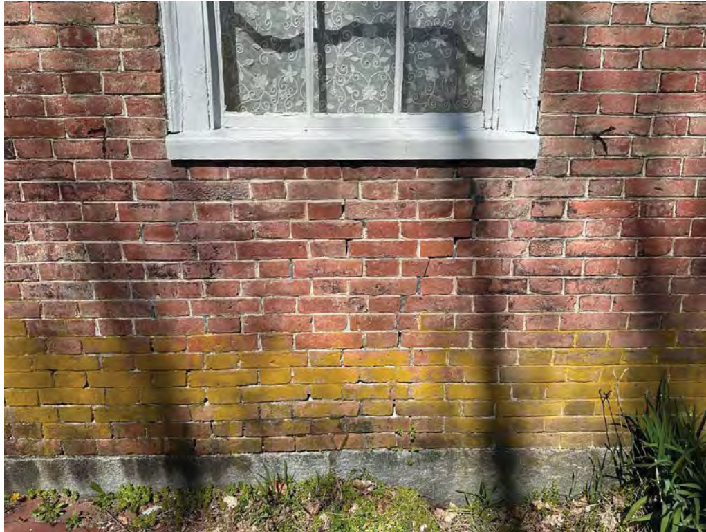
Figure 4.2-5 Crack on the east elevation below W-07. Previously improperly patched.
