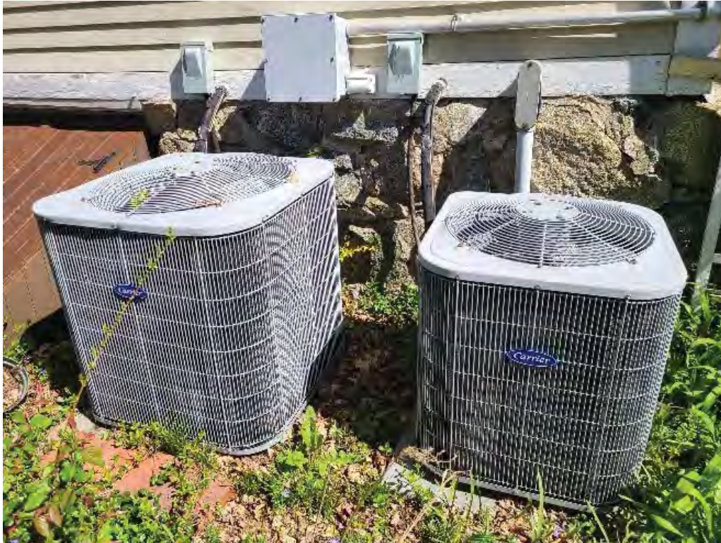
Figure 9.2-1 First Floor (Right) and Second Floor (Left) Outdoor Condensing Units.
