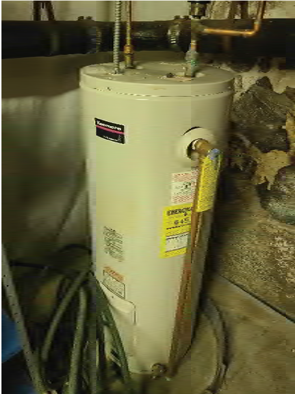
Figure 9.3-2 Electric Domestic Hot Water Heater.
