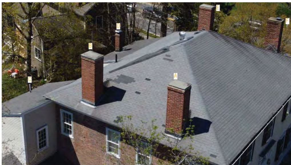
Figure 4.12-1 Chimney A services: FP-01 & FP-07
