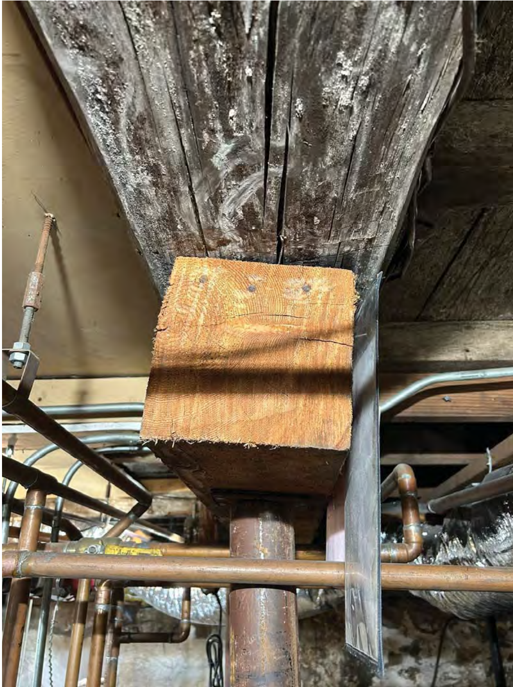
Figure 8.3-9 Rotated low support beam with torsional cracking.
