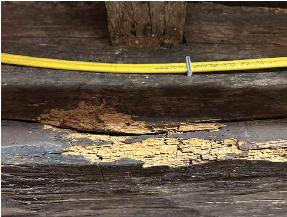
Figure 8.3-12 Deteriorated original timber beam.
