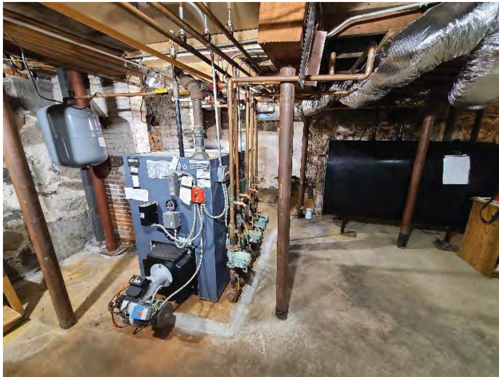
Figure 9.1-2 Boiler System and Fuel Oil Storage Tank Located within Basement B-01.
