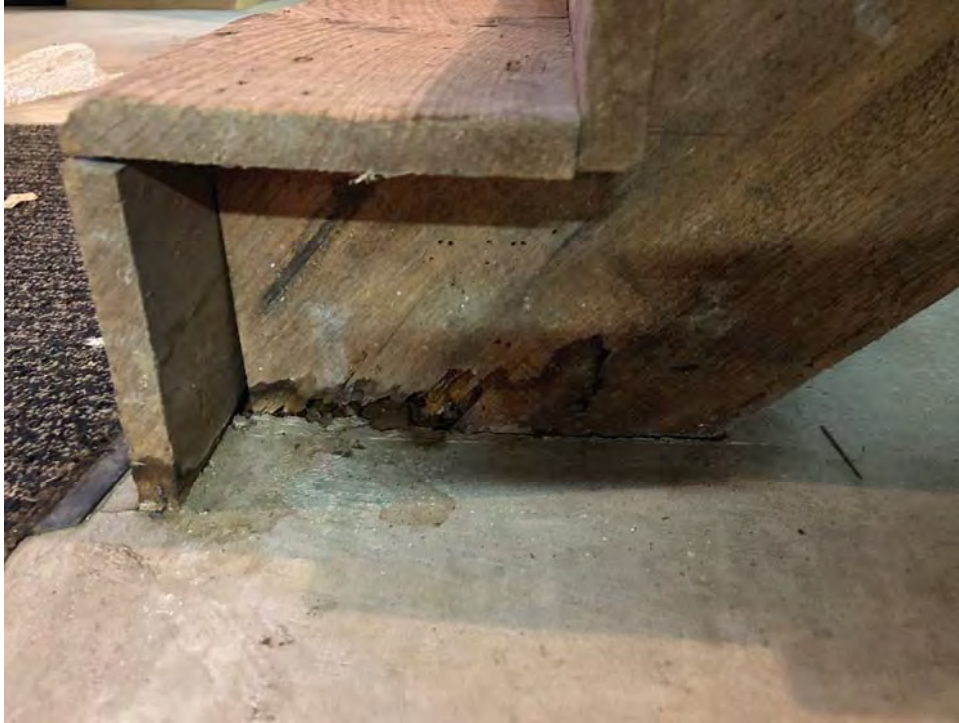
Figure 8.3-3 Deteriorated stringer bearing.
