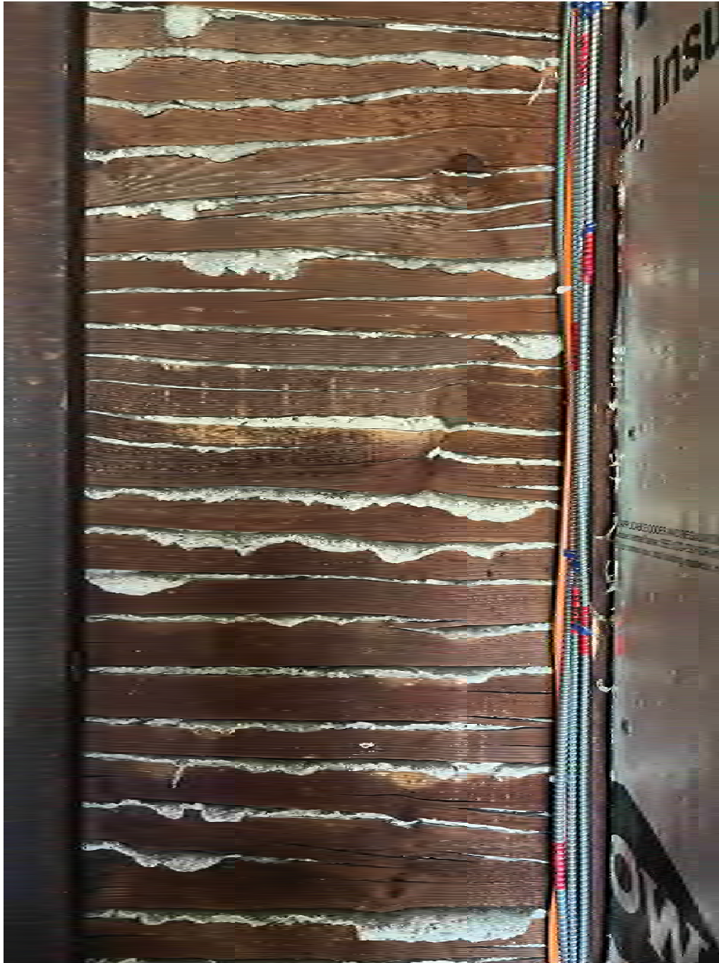
Figure 4.10-21 Bare lathe wall in S-05.
