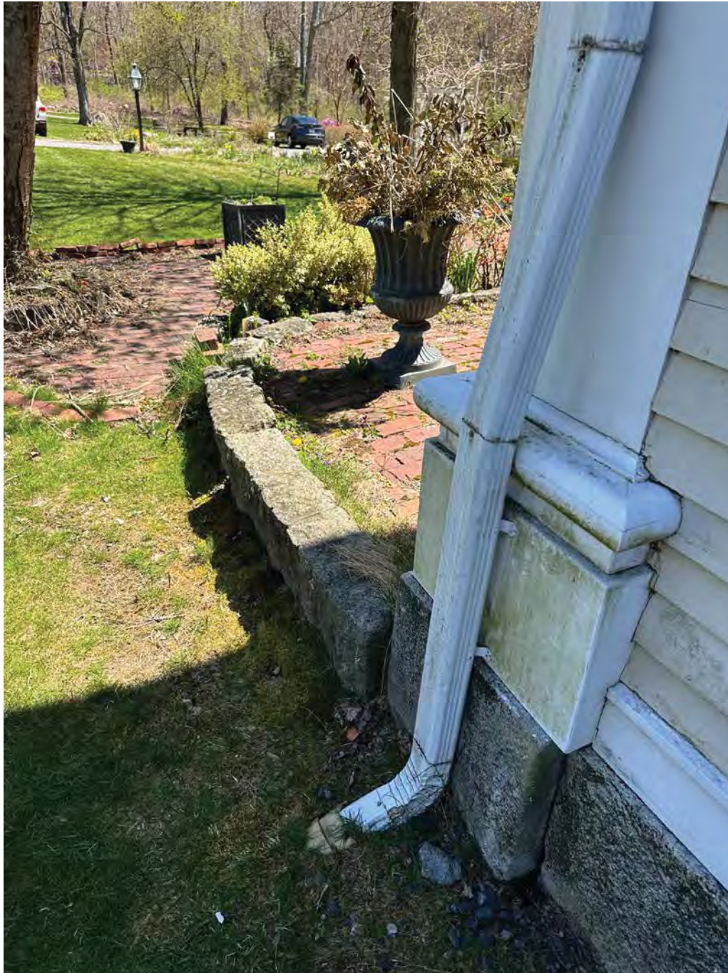
Figure 4.7-1 Located at the northeast corner of the house is a downspout missing an elbow to help expel water away from the immediate perimeter of the house, below grade.
