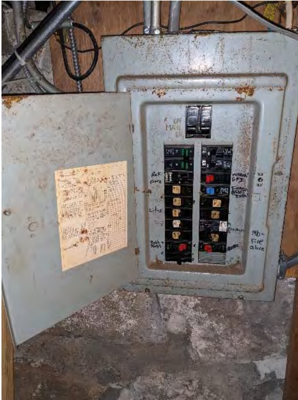
Figure 9.7-1 100A, 120/240V, single phase panel with rust damage.
