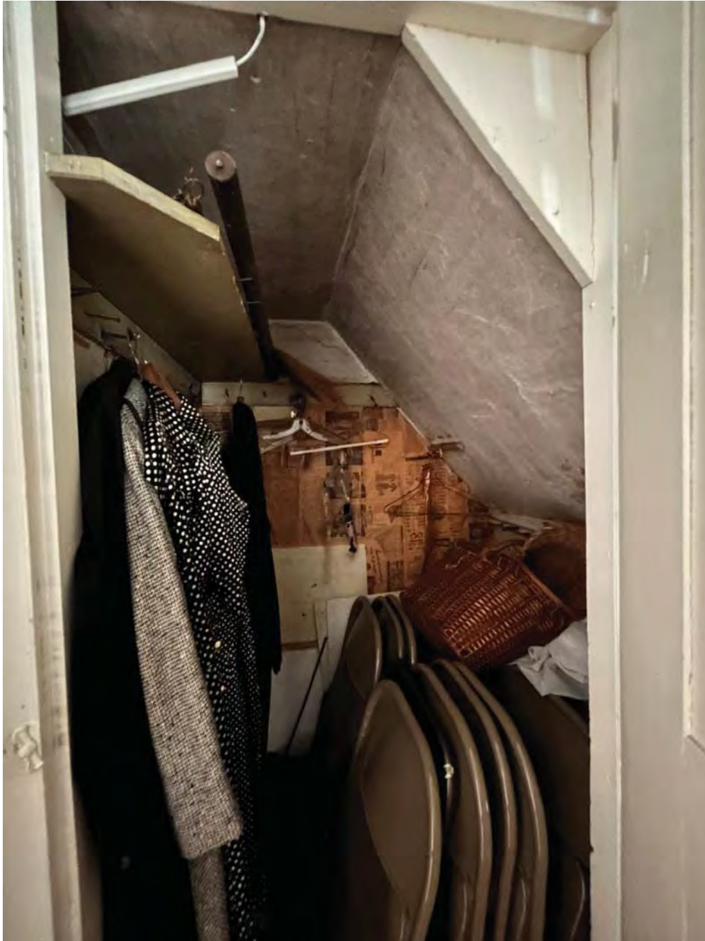
Figure 8.3-19 Cracking in ceiling under stair to attic.
