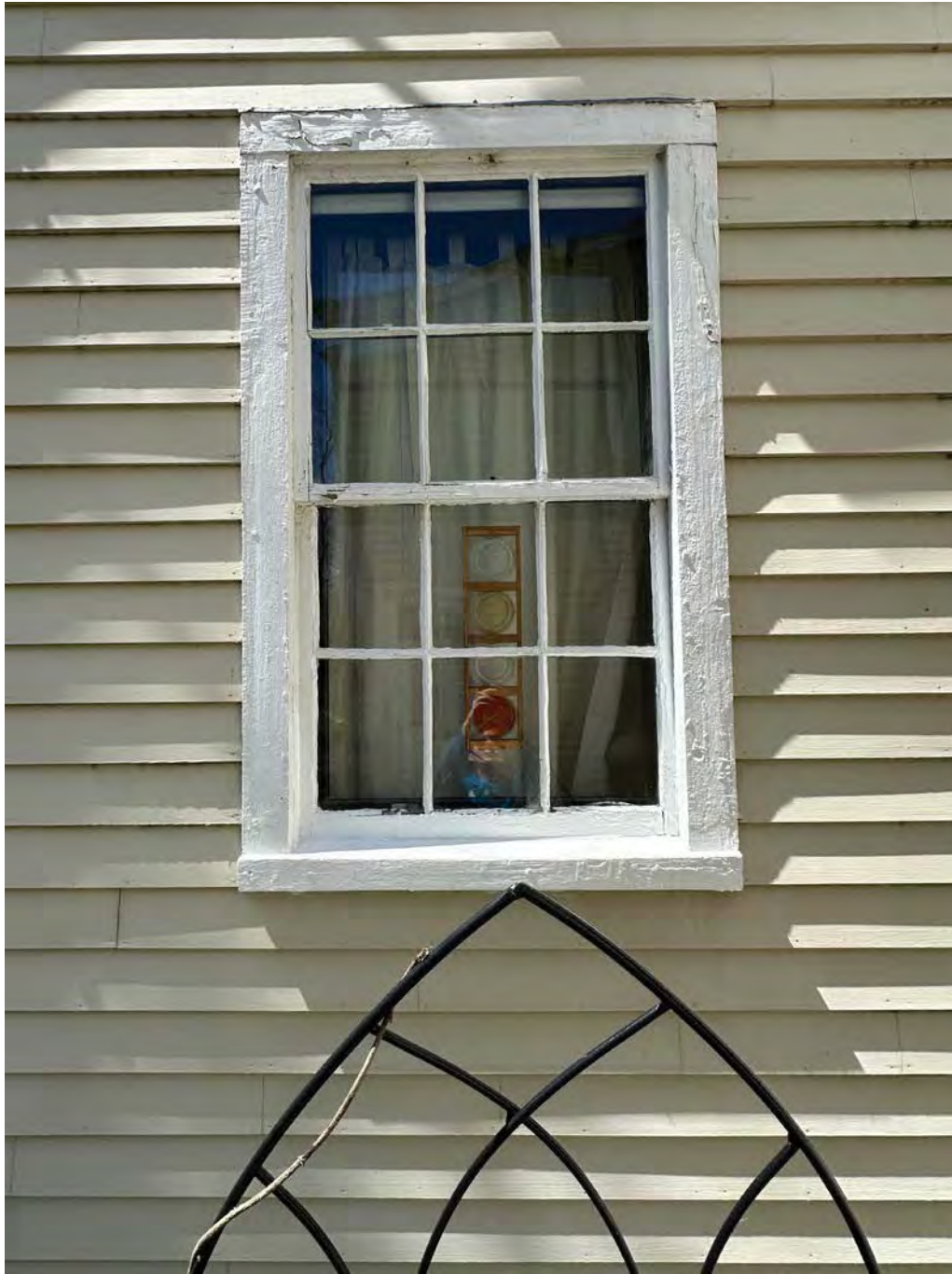
Figure 4.4-6 Minor wood damage and peeling paint found typically over all elevations.
