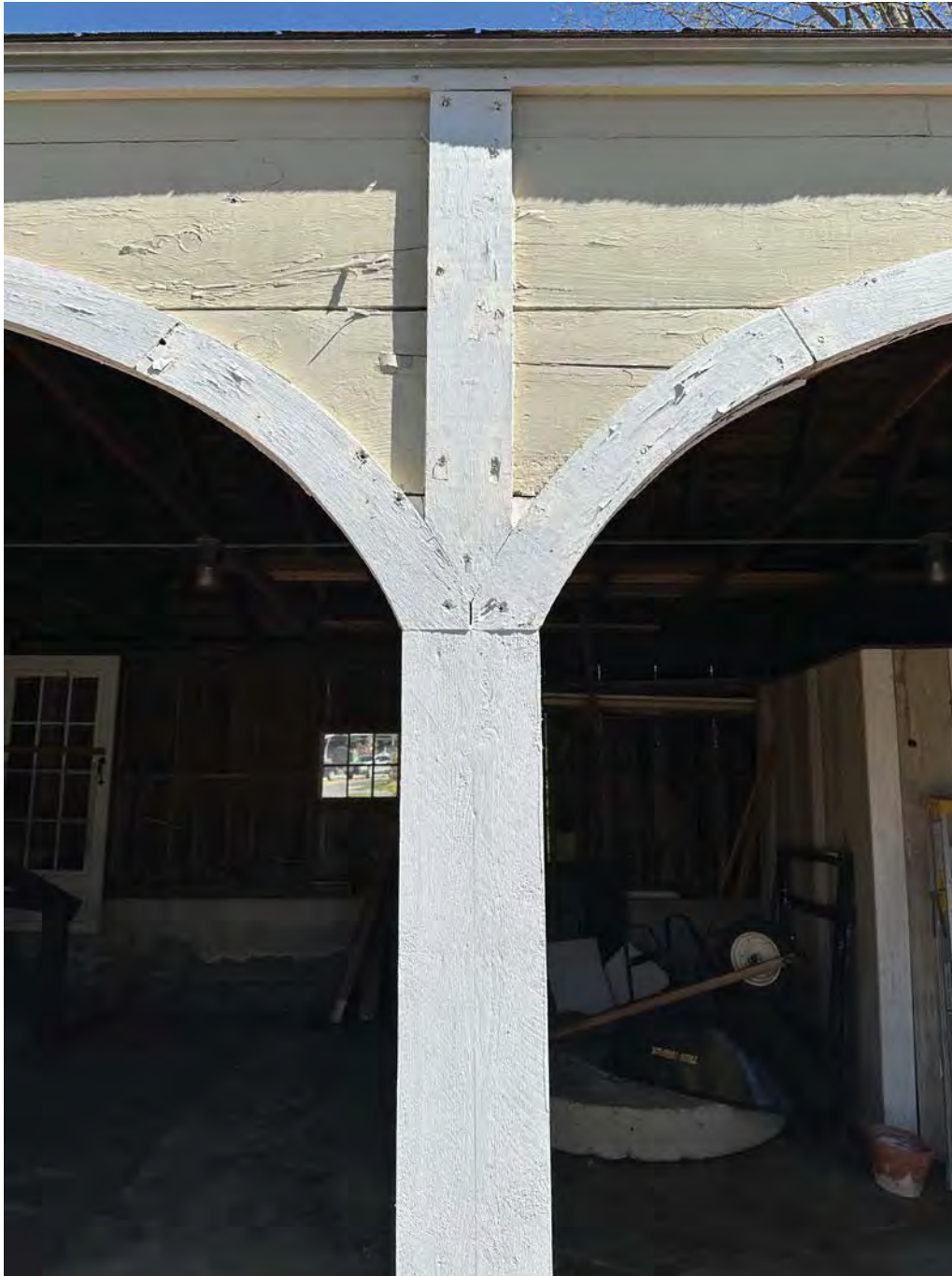
Figure 4.1-9 Peeling paint at carriage house columns and arches.
