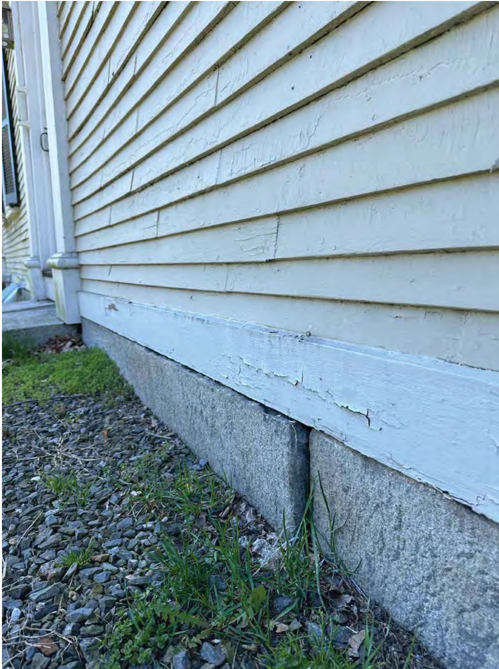
Figure 4.1-7 Splits in the wood ranging from 1 linear foot to 2 linear feet.
