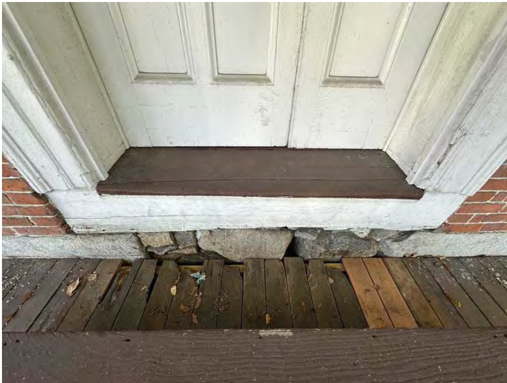
Figure 4.9-3 The decking planks directly below the door threshold are rotted, and are exhibit the most severe deterioration of the deck.
