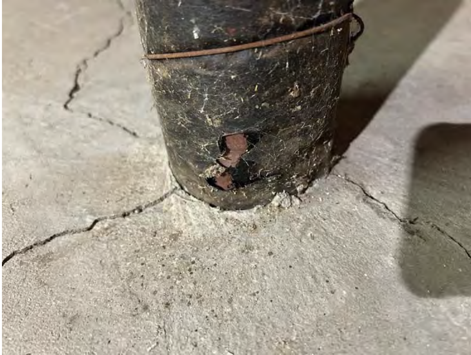
Figure 8.3-1 Failed post waterproofing.
