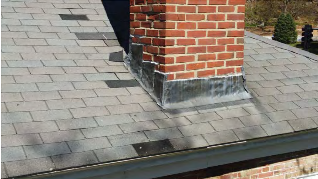
Figure 4.8-3 The step-flashing around the chimneystacks and crickets is in poor condition due to general end-of-life degradation as edges of the flashing are upturned and portions of the step-flashing are separating.
