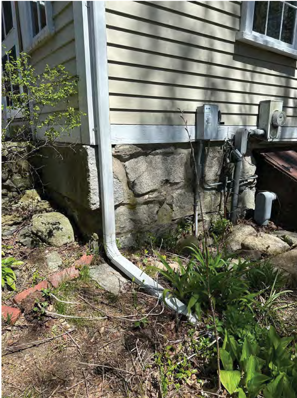
Figure 4.7-8 This downspout terminates an appropriate distance from the house's foundation, and expels water above grade, however is visibly clogged at its termination.
