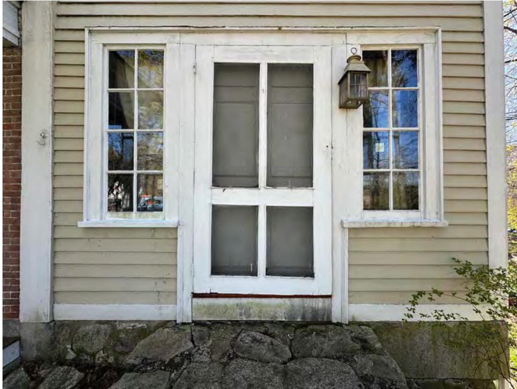
Figure 4.4-2 Two vertical fixed wood windows flanking the office entrance door (D- 21). The screen door was found to be damaged and inappropriate in design.
