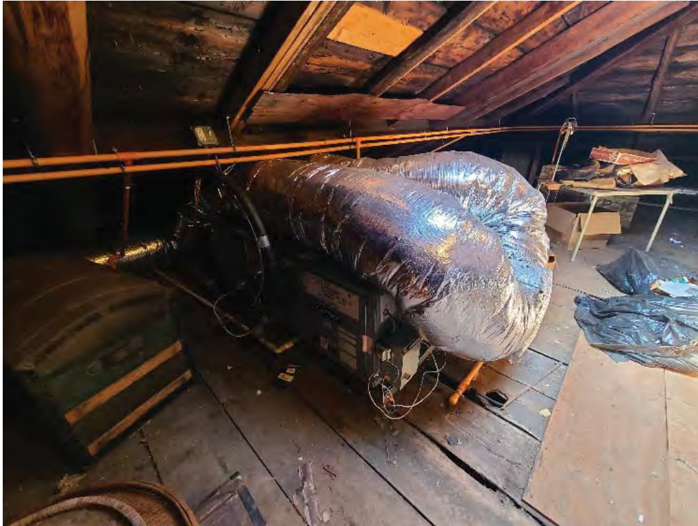
Figure 9.2-3 Second Floor Ducted Fan Coil Unit Located within the Attic (A-01).
