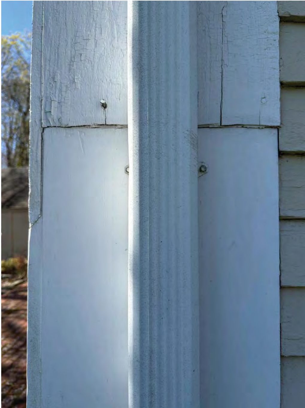
Figure 4.1-13 At the joint of the repaired pilasters, there are several splits in the wood ranging from 8 inches to 2 feet in length.
