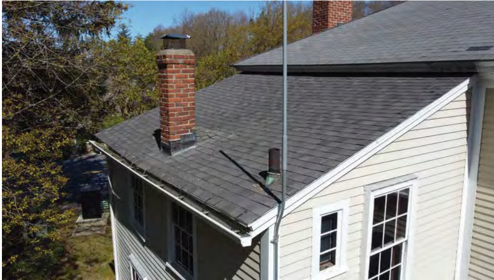
Figure 4.7-6 Visible along the sloped edge of the roof are gutter straps, which are puncturing the roof membrane.
