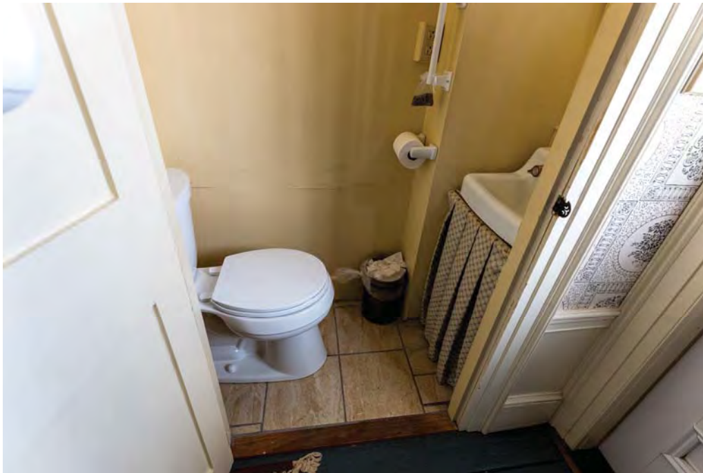
Figure 4.11-9 Modern tiling in room F-06 is in good condition, however it is not historically accurate to the house.
