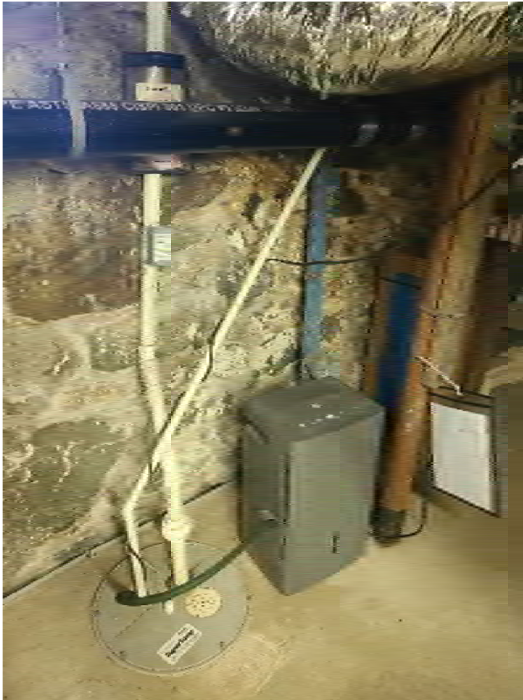
Figure 9.2-7 Basement (B-01) Dehumidifier tied to Sump Pump Pit.
