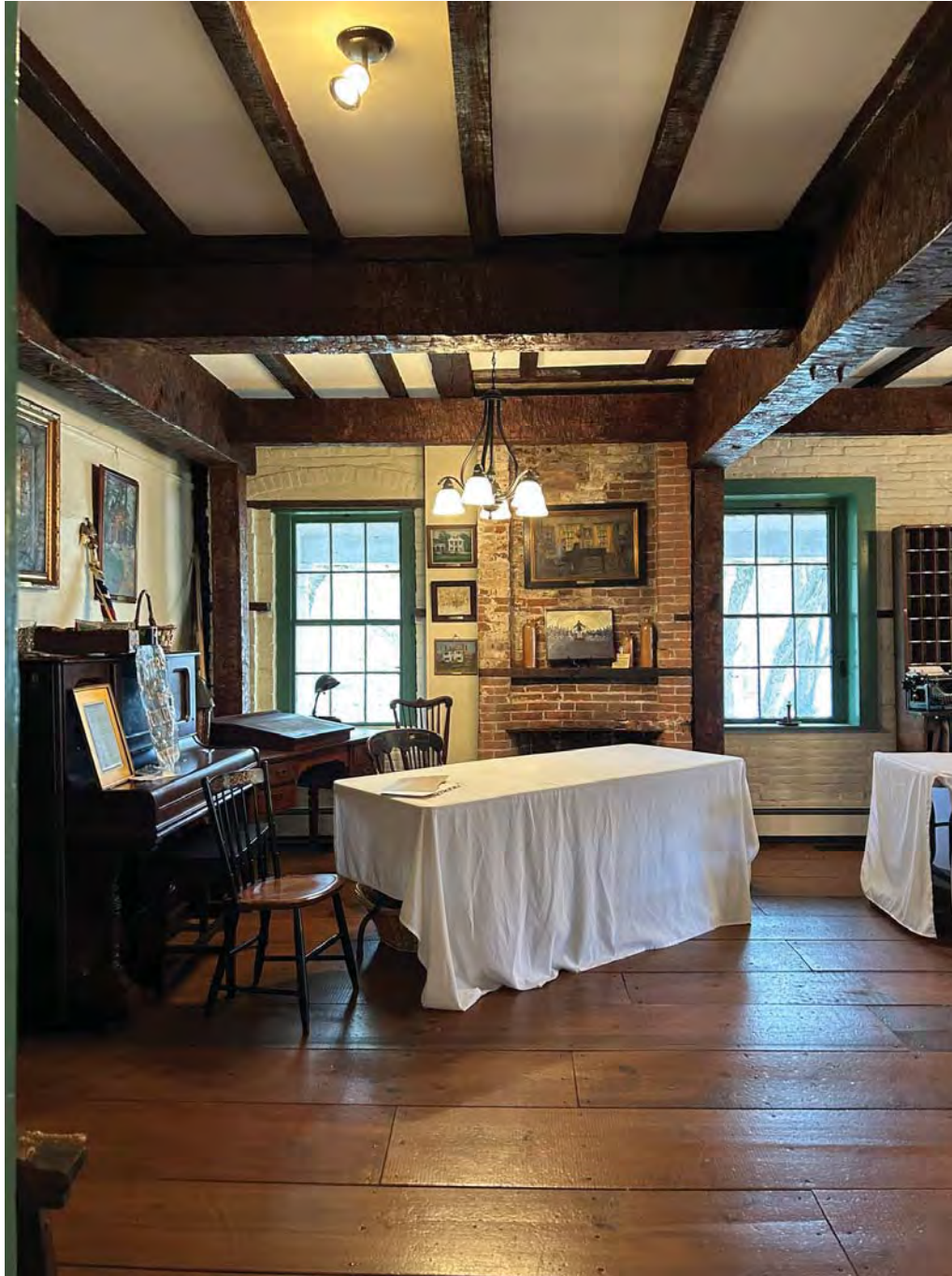
Figure 8.2-7 Dropped, wood clad steel beams at south end of storeroom.
