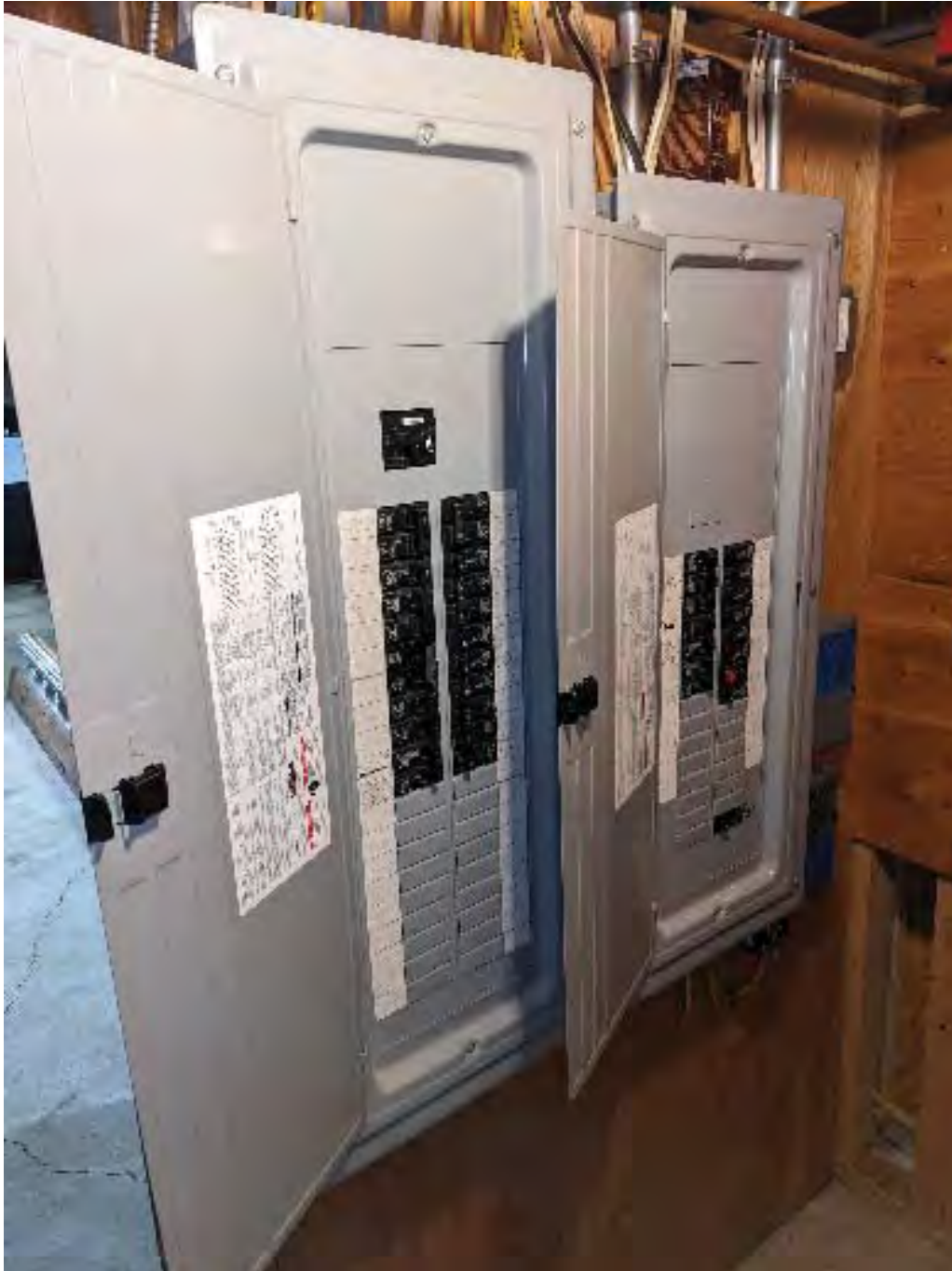
Figure 9.7-2 Newer 200A, 120/240V, single phase panels.
