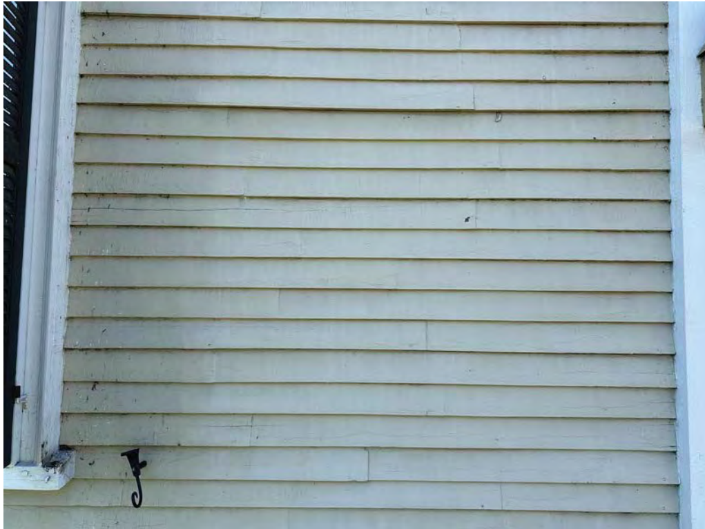
Figure 4.1-4 Large horizontal cracks visible across the north elevation.
