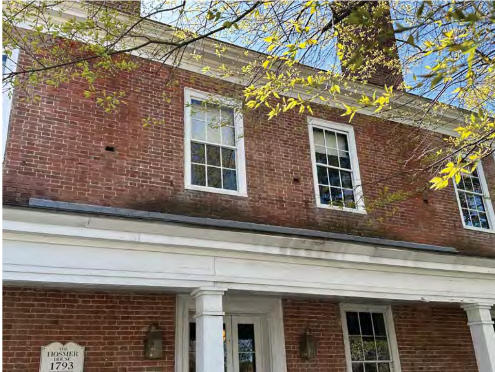
Figure 4.2-2 Discolored bricks due to water infiltration. And inadequate flashing.
