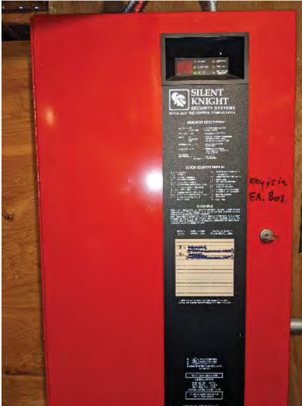
Figure 9.9-1 Silent Knight Fire Alarm Control Panel.
