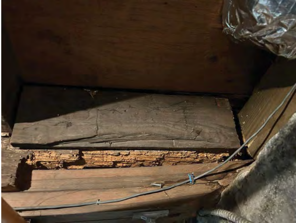
Figure 8.3-15 Previous splice at north bearing of west central beam.
