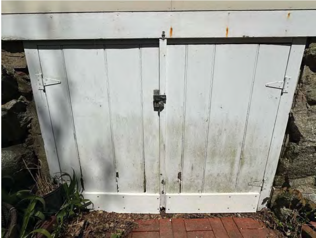
Figure 4.1-11 Fasteners used to secure the trim, corner boards and water tables have begun to corrode and stain the wood.
