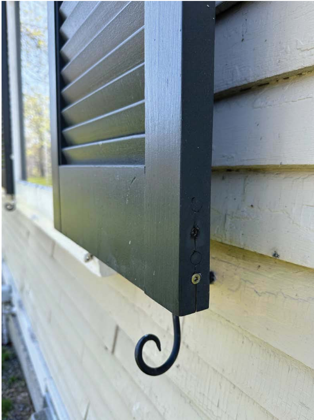
Figure 4.5-3 Instances where the bottom rail of the shutter has become loose. A repair had been made by inserting a screw into the side of the stiles, through to the bottom rail, however this seems to have failed as well, as the wood around the screw is now splitting.
