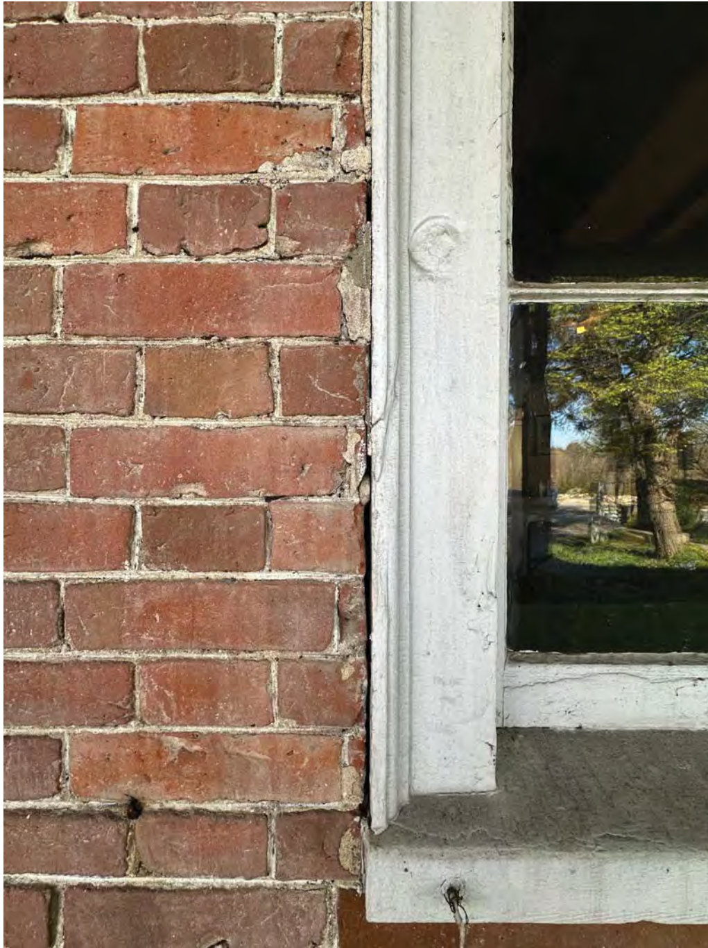
Figure 4.4-13 The perimeter sealant and glazing putty around the windows appear deteriorated, with cracks and gaps in some locations, leading to poor performance.
