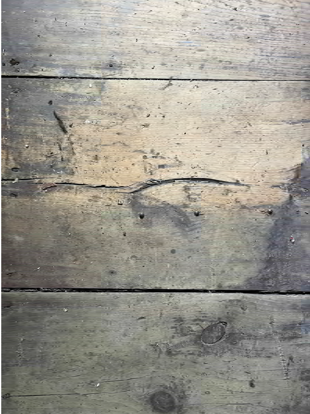
Figure 4.11-7 Splits in the wood were observed in room F-05, as well as evidence of past repairs, where wood has weakened due to water damage.
