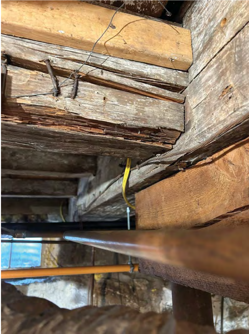
Figure 8.3-10 Deteriorated trimmer east end connection.
