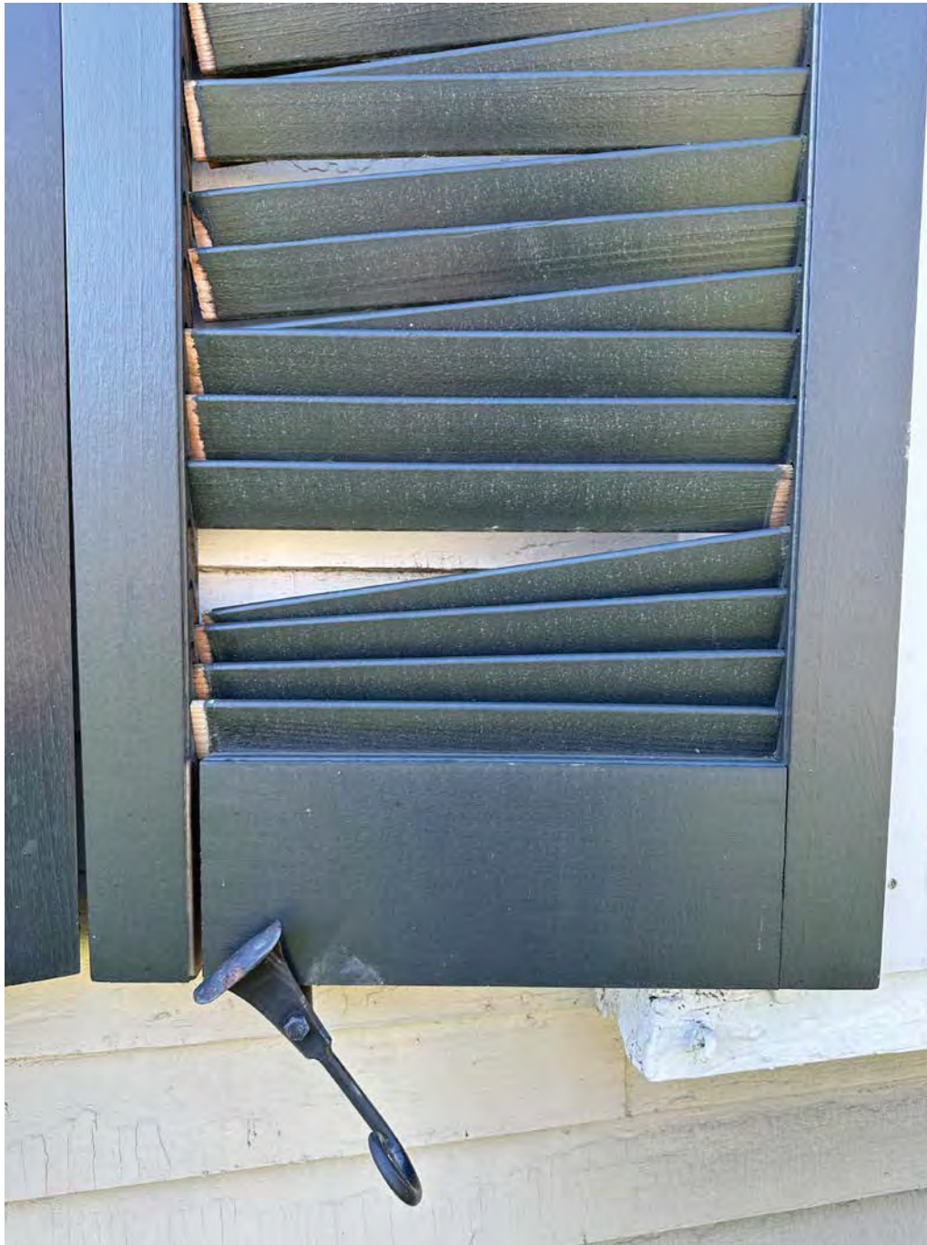
Figure 4.5-2 Louvers which have fallen out of place. Typical condition seen throughout.
