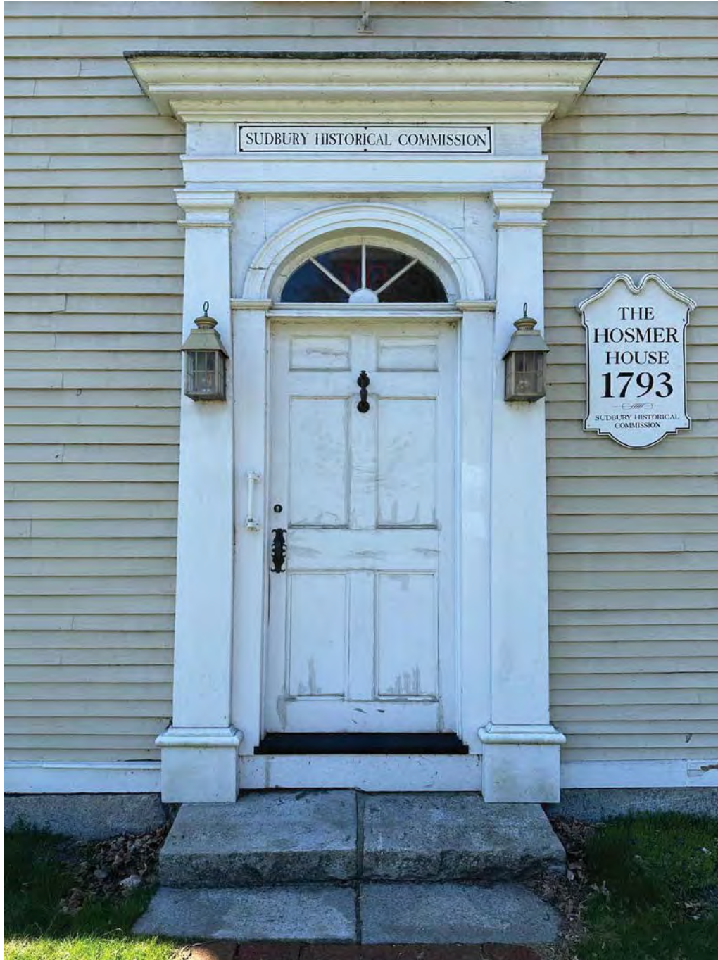
Figure 4.4-7 D-01 in poor-to-fair condition, showing signs of wood deterioration, cracks, and previous repairs.
