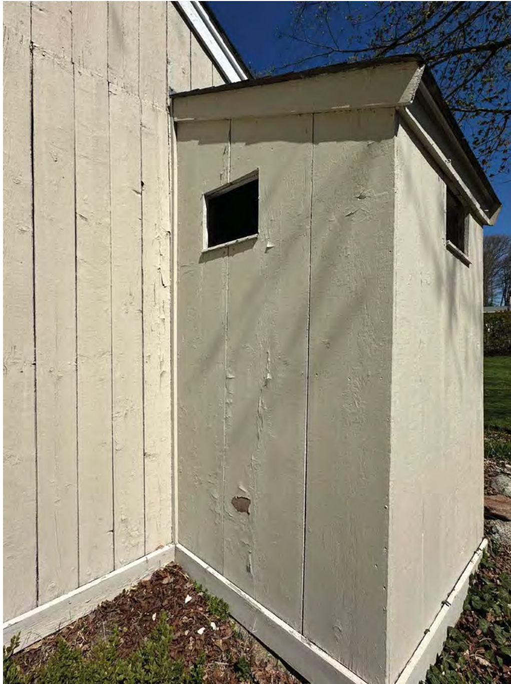
Figure 4.1-10 Vertical planks at outhouse are an average of 15" in width. Visible gaps varying approximately 1" to 2" in width, and peeling paint.
