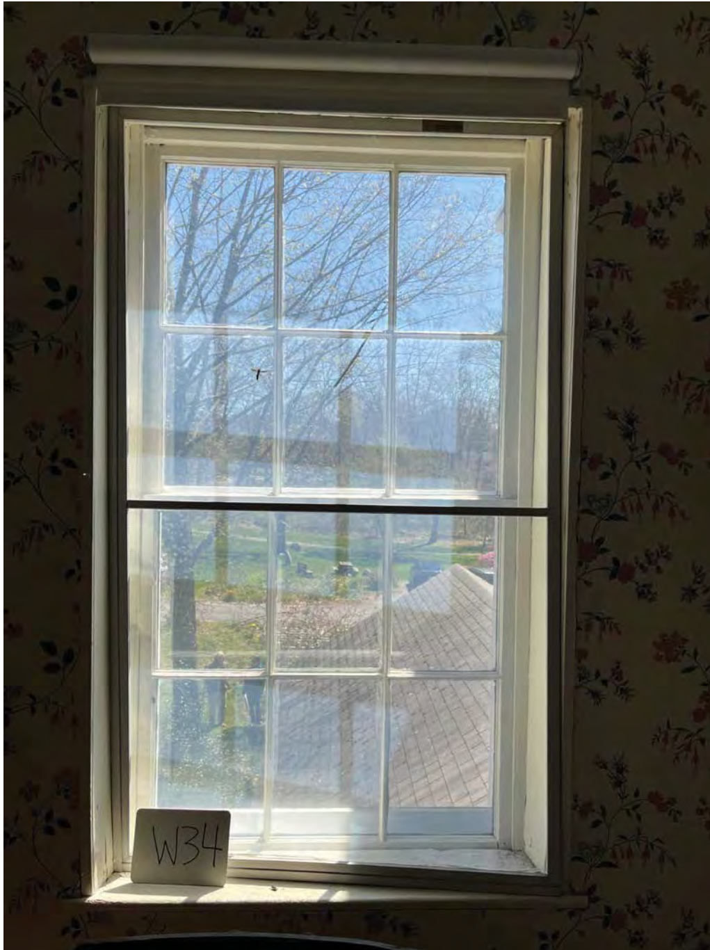
Figure 4.4-3 Window inserts painted white and installed at the interior of the windows.
