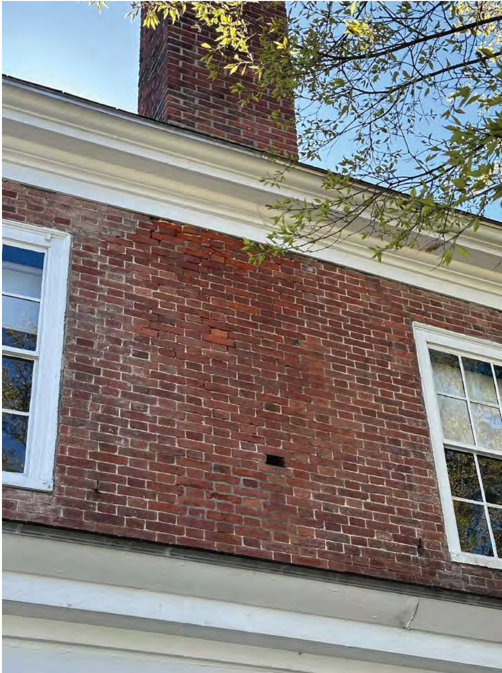
Figure 4.2-7 There are two areas on the west elevation of approximately 3' by 5' between windows W-46 and W-47, which show signs of deterioration. Bricks are missing their fire faces or cracked, and there is extensive mortar loss.
