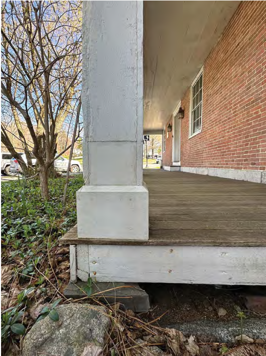
Figure 4.9-6 Between 12" to 14" of the shafts of the two columns at either end of the porch have been replaced along with all 4 column capitals and bases.
