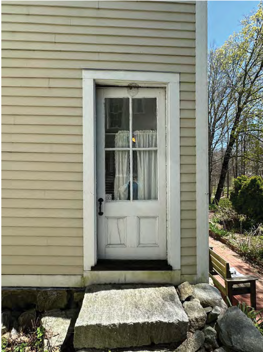
Figure 4.4-8 D-12 in poor-to-fair condition, showing signs of wood deterioration, cracks, and previous repairs.
