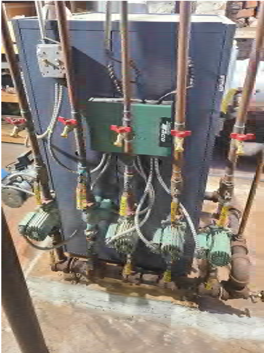
Figure 9.1-3 Hot Water Heating System Recirculation Pumps and Switching Relay.
