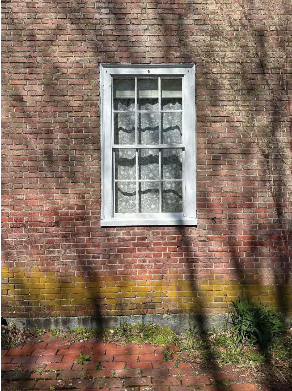
Figure 4.2-3 Extensive biological growth on the east elevation along the entire wall.
