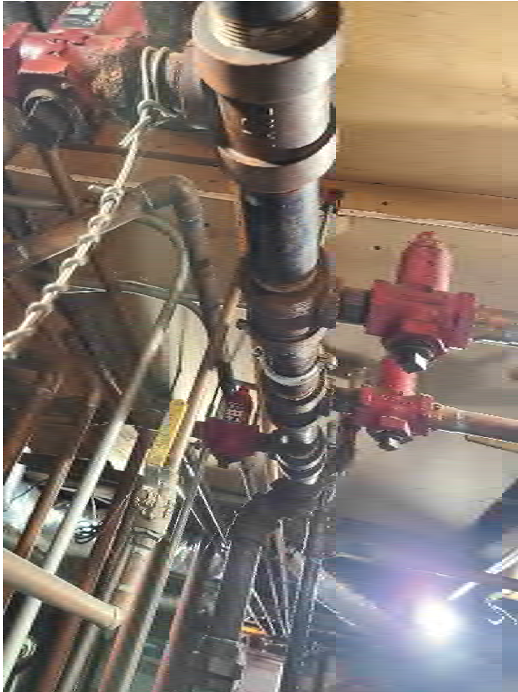
Figure 9.1-4 Hot Water Heating System Control Valves.
