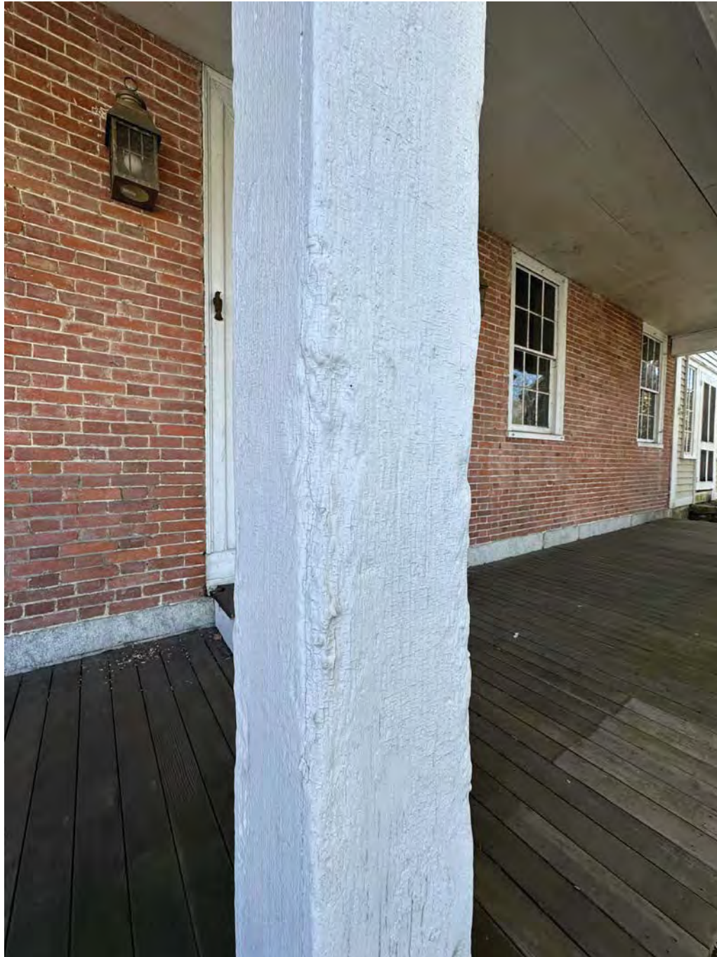
Figure 4.9-4 The 4 columns which support the porch roof are in poor-to-fair condition. The shaft of the columns have degraded over time, and have lost material mass at various locations.
