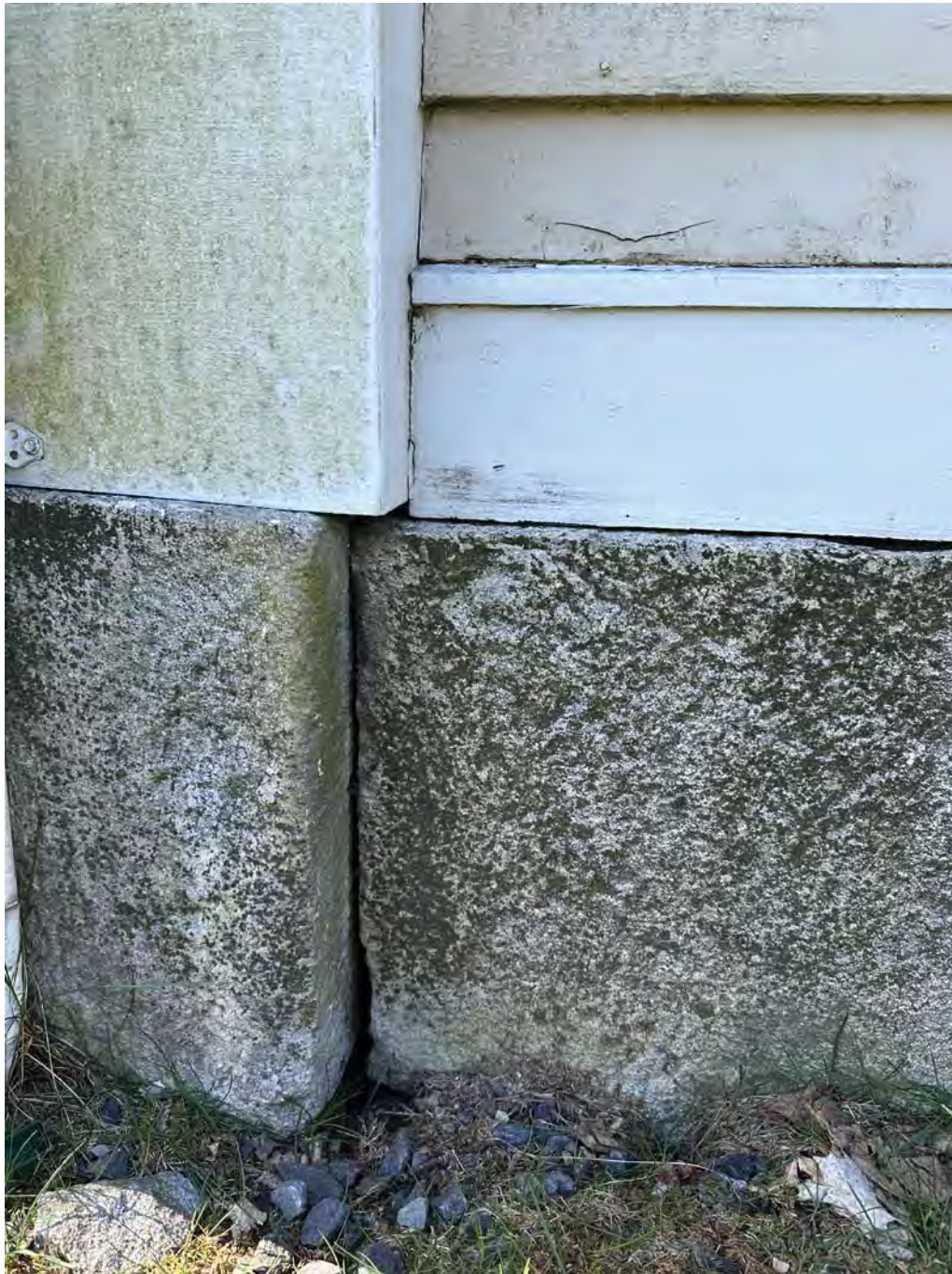
Figure 4.3-1 Along the north, east and west elevations, the base is constructed with a single rectilinear cut stone which sits directly below the exterior cladding system.
