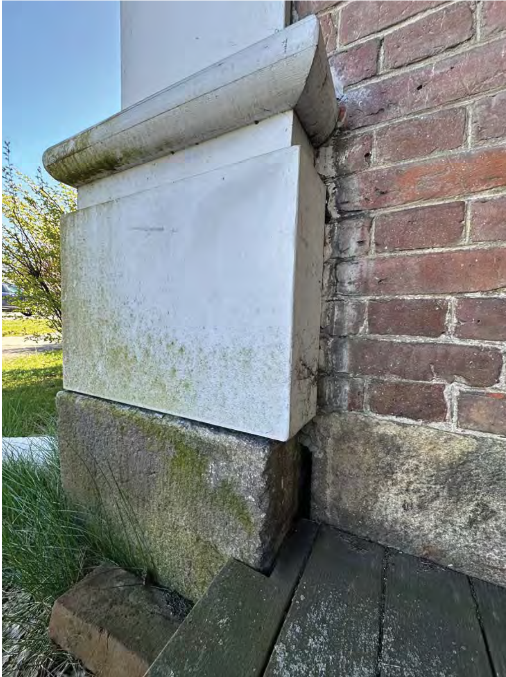
Figure 4.3-4 There is no evident base flashing between the wood pilaster and the granite foundation.
