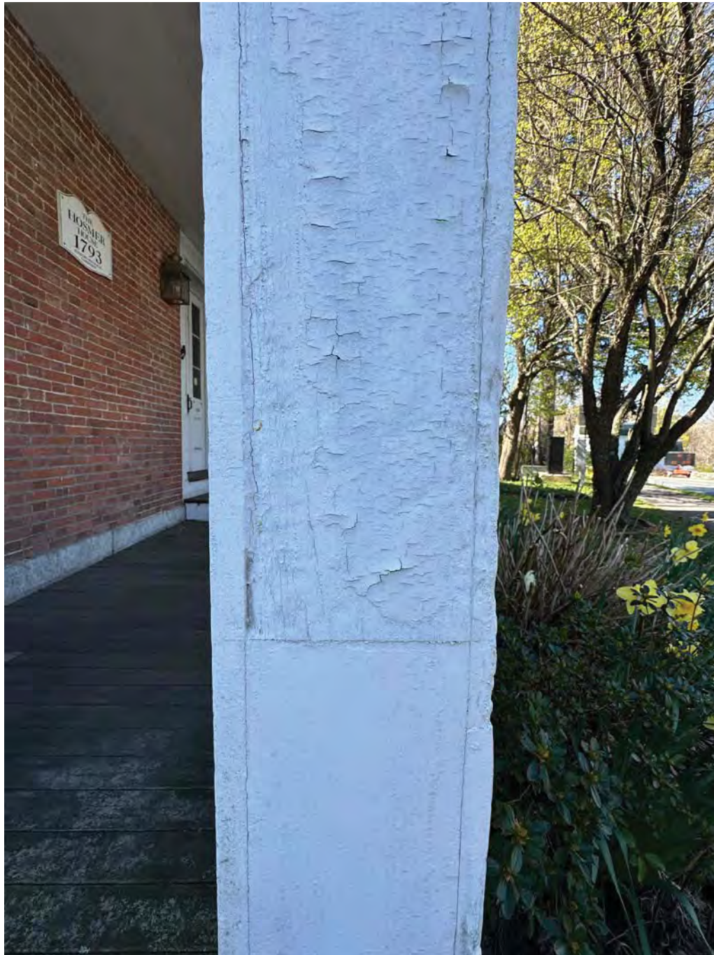
Figure 4.9-5 Between 12" to 14" of the shafts of the two columns at either end of the porch have been replaced along with all 4 column capitals and bases.
