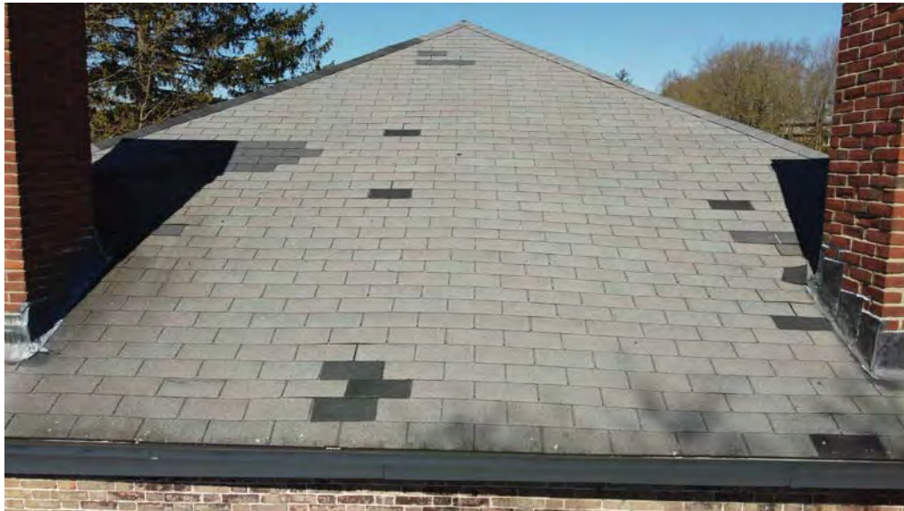
Figure 4.6-6 Selective shingle replacement is visible at several locations on the east slope of the main roof, and south slope near a vent pipe, as well as a portion of the ridge cap shingles along the southeast ridge. Also visible were some shingles which have become dislodged.
