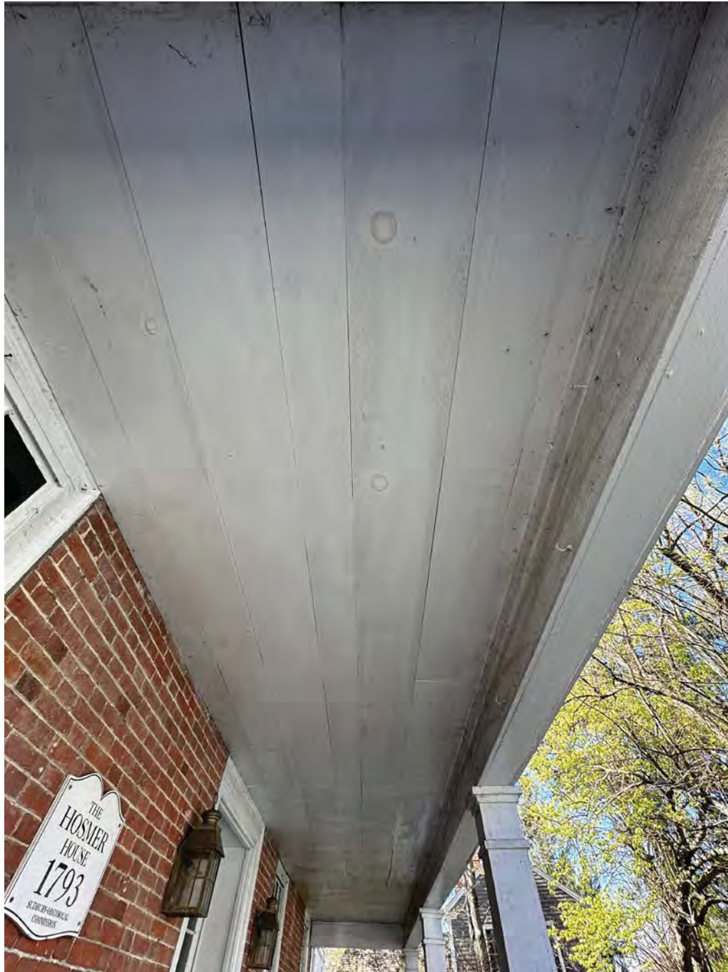
Figure 4.9-7 The porch ceiling is in good condition. The ceiling board at the underside of the roof is relatively new, however, oils are being drawn out from the knots in the wood, creating brown rings which telegraph through the white paint, typical throughout.
