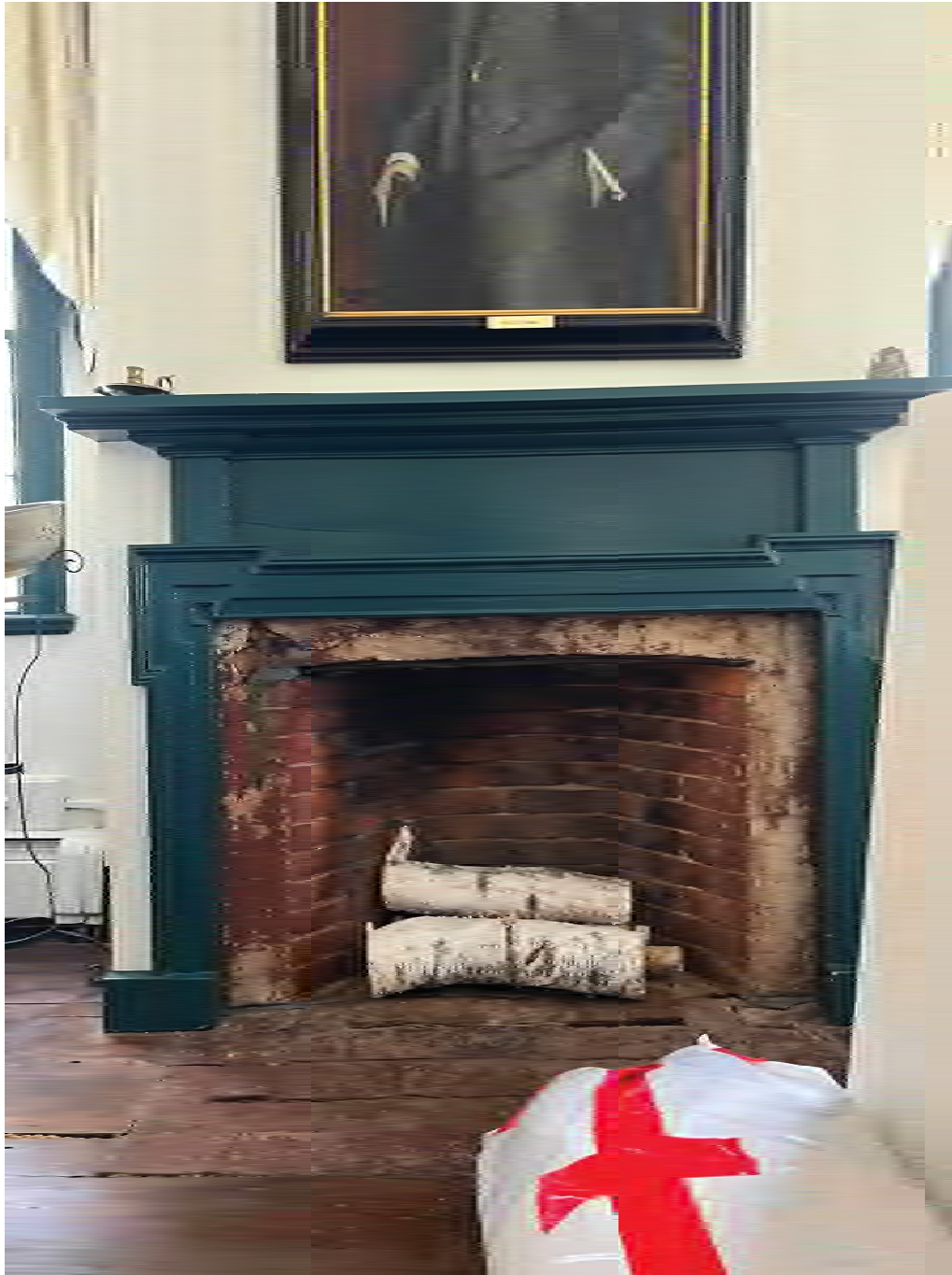
Figure 4.12-11 Painted decorative wooden mantel in room S-09. Lintel shows signs of corrosion.
