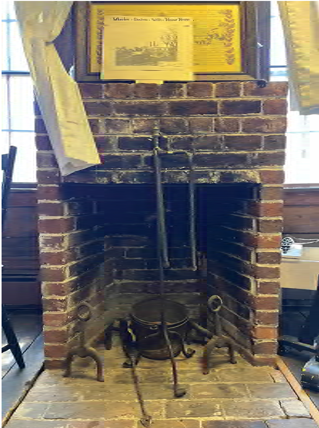
Figure 4.12-9 Corroded fireplace lintel in room F-07.
