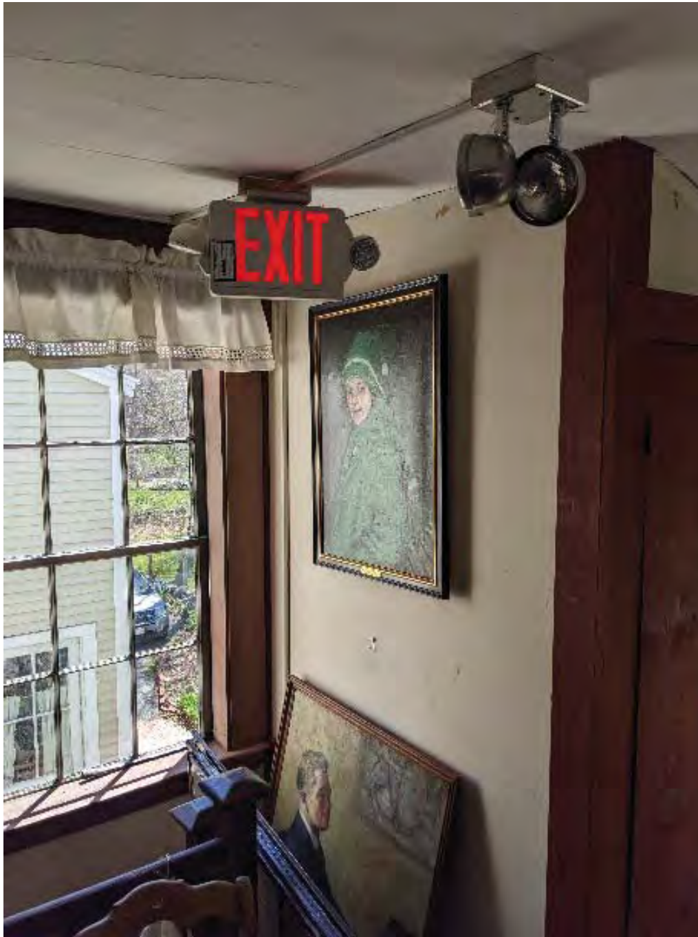
Figure 9.8-3 Existing exit signs and emergency lighting.
