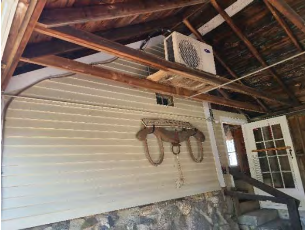
Figure 9.2-5 Disconnected 9,000 MBH Split System Condensing Unit Located within Carriage House.
