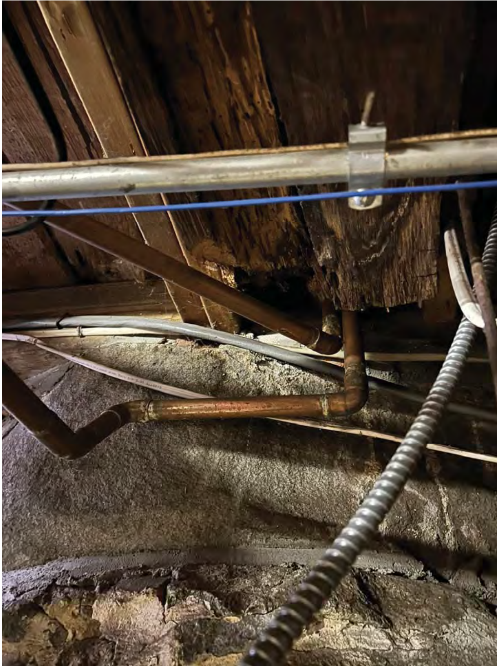
Figure 8.3-14 Void at previous beam bearing along south wall.
