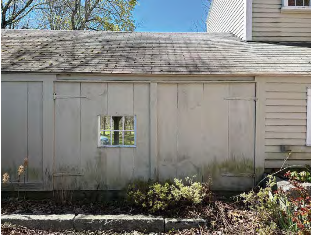
Figure 4.6-10 The carriage house roof is an open gable roof structure which slopes north and south on the site, and has no penetrations. Along the north-facing slope, there is extensive biological growth in the form of moss growing sporadically over the entire surface.
