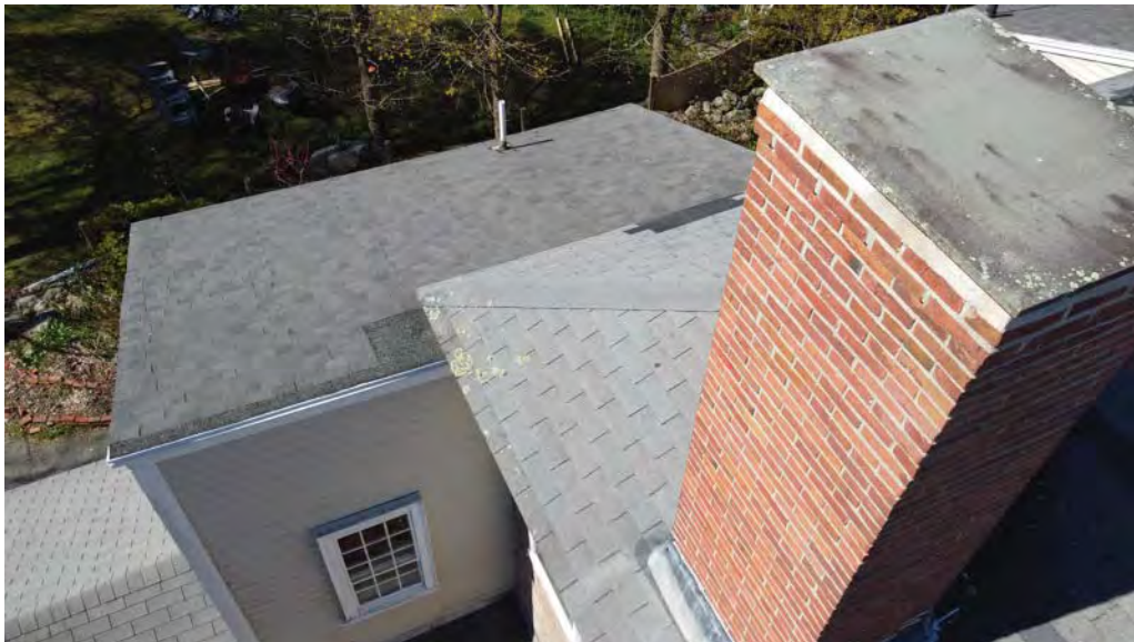
Figure 4.6-9 Both roofs of the additions are in the style of a shed roof, in fair condition.
