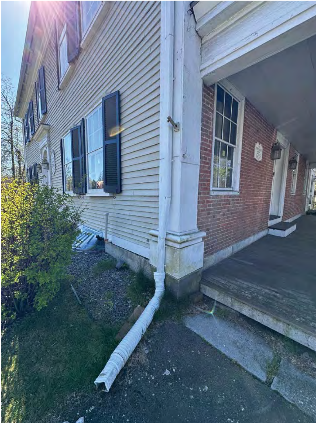
Figure 4.7-2 Located at the northwest corner of the house is a downspout that expels water through a downspout extension above grade, away from the house's foundation walls.
