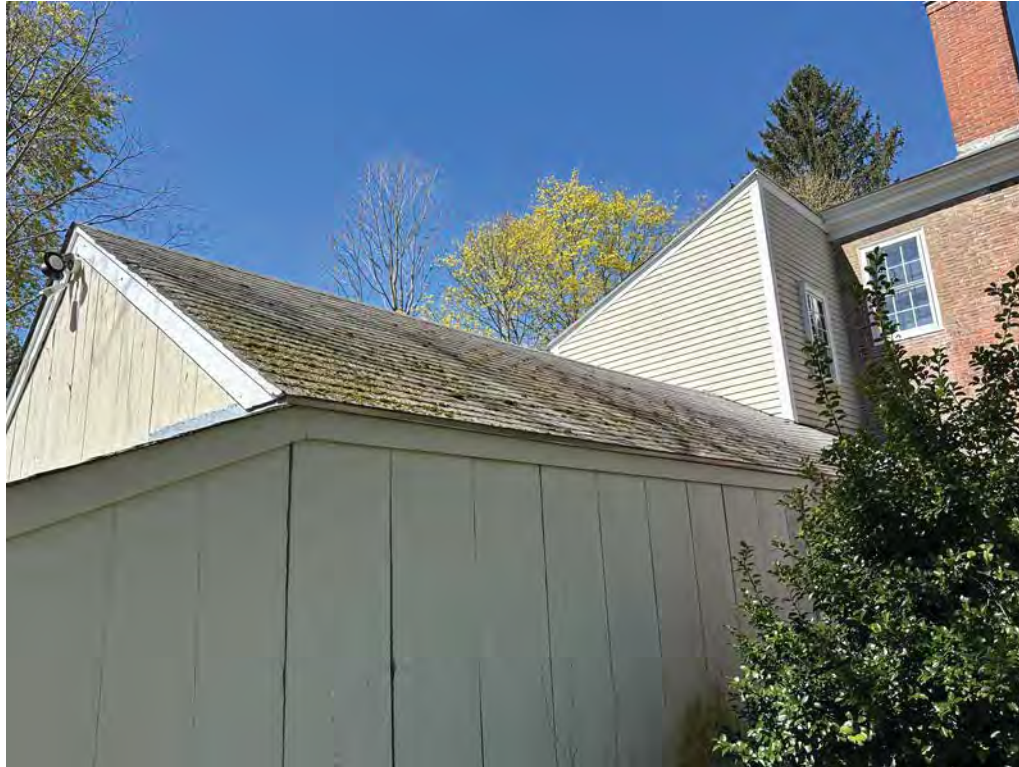
Figure 4.6-11 The carriage house roof is an open gable roof structure which slopes north and south on the site, and has no penetrations. Along the north-facing slope, there is extensive biological growth in the form of moss growing sporadically over the entire surface.
