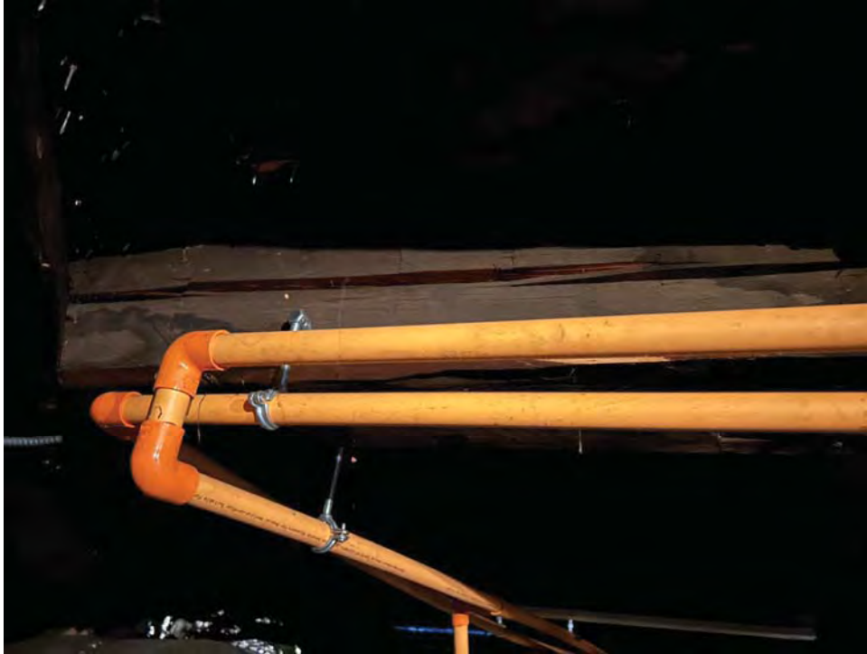
Figure 8.3-20 Large checks in roof purlin, southeast corner.
