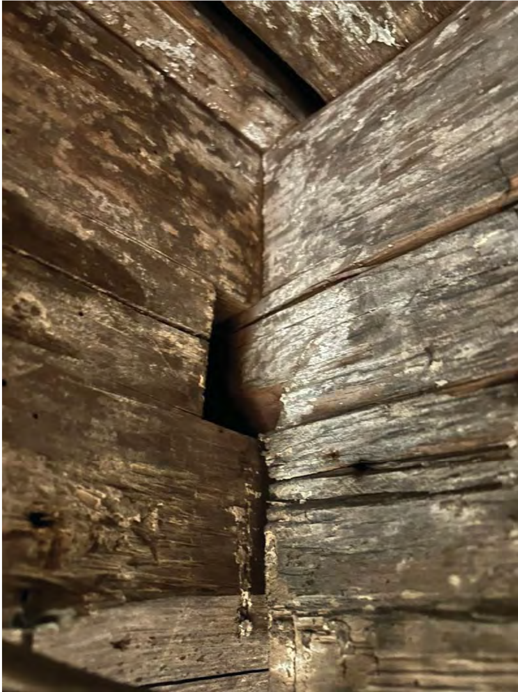
Figure 8.3-8 Wood deterioration at header to trimmer connection.
