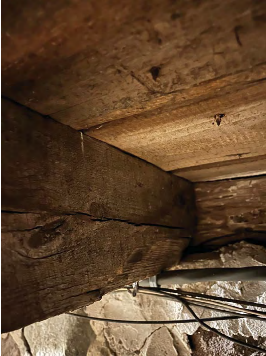
Figure 8.3-4 Fill length split in sister.
