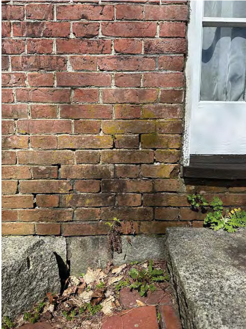
Figure 4.2-8 Several areas along the base of the building on the east elevation in which the mortar has deteriorated due to water infiltration, and in these gaps, small plants have taken root.
