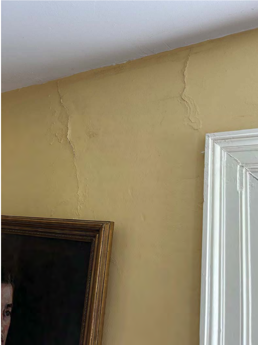
Figure 8.3-17 Cracking in north wall of parlor.
