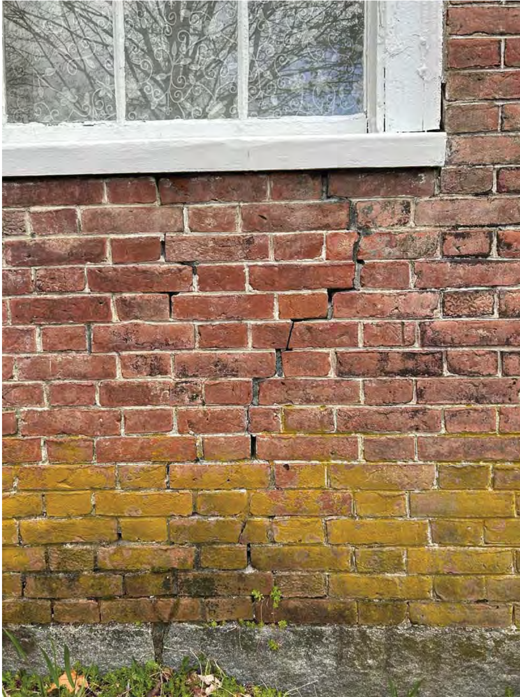
Figure 8.3-22 Masonry cracking in east wall.
