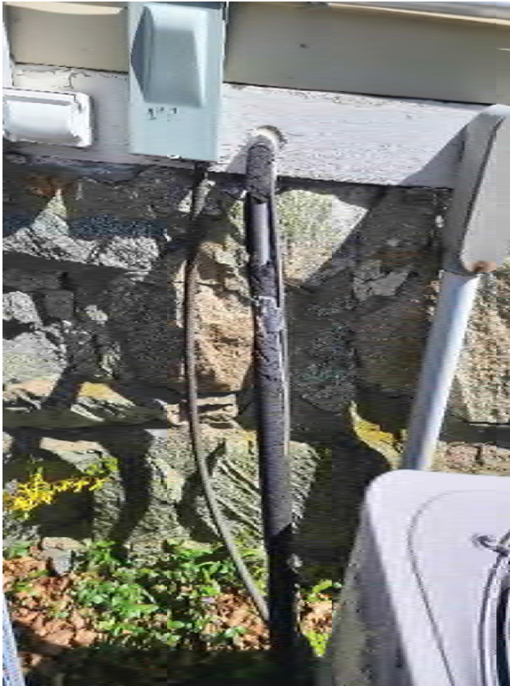
Figure 9.2-4 Insulated Refrigerant Suction Line (Left) and Uninsulated Refrigerant Liquid Line (Right).
