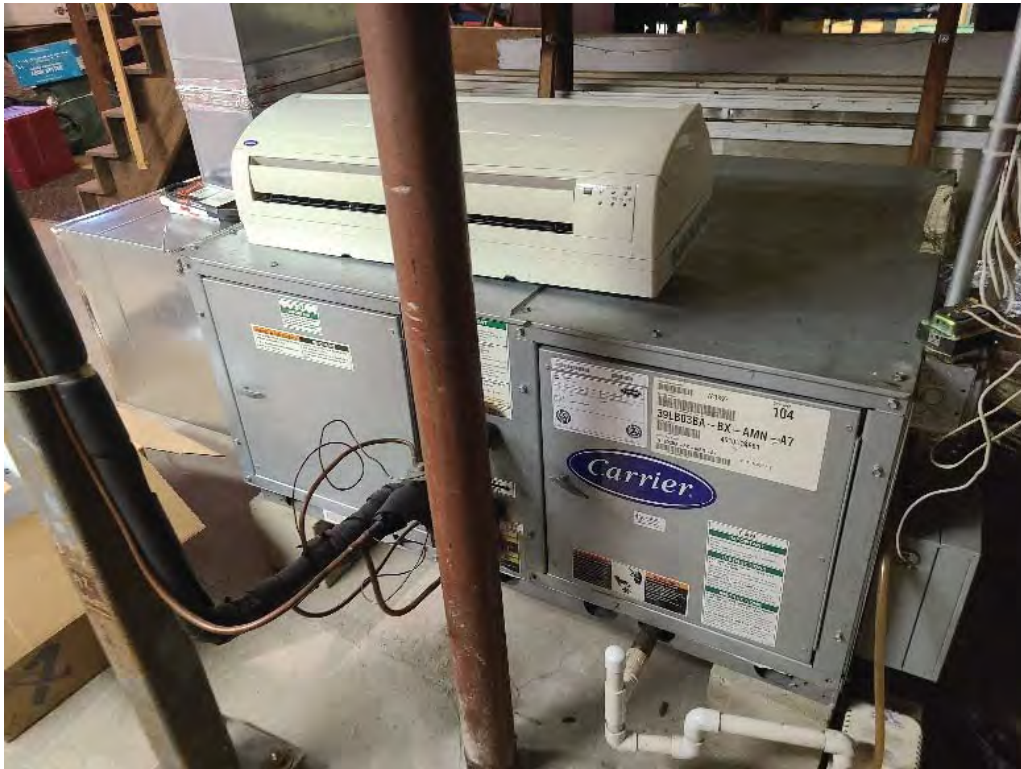
Figure 9.2-2 First Floor Ducted Fan Coil Unit Located within Basement (B-01).
