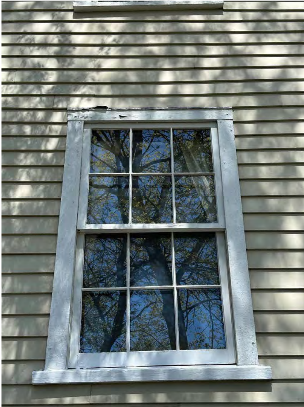
Figure 4.4-14 Metal window head flashing was noted at most windows but appears bent or poorly installed in some areas.
