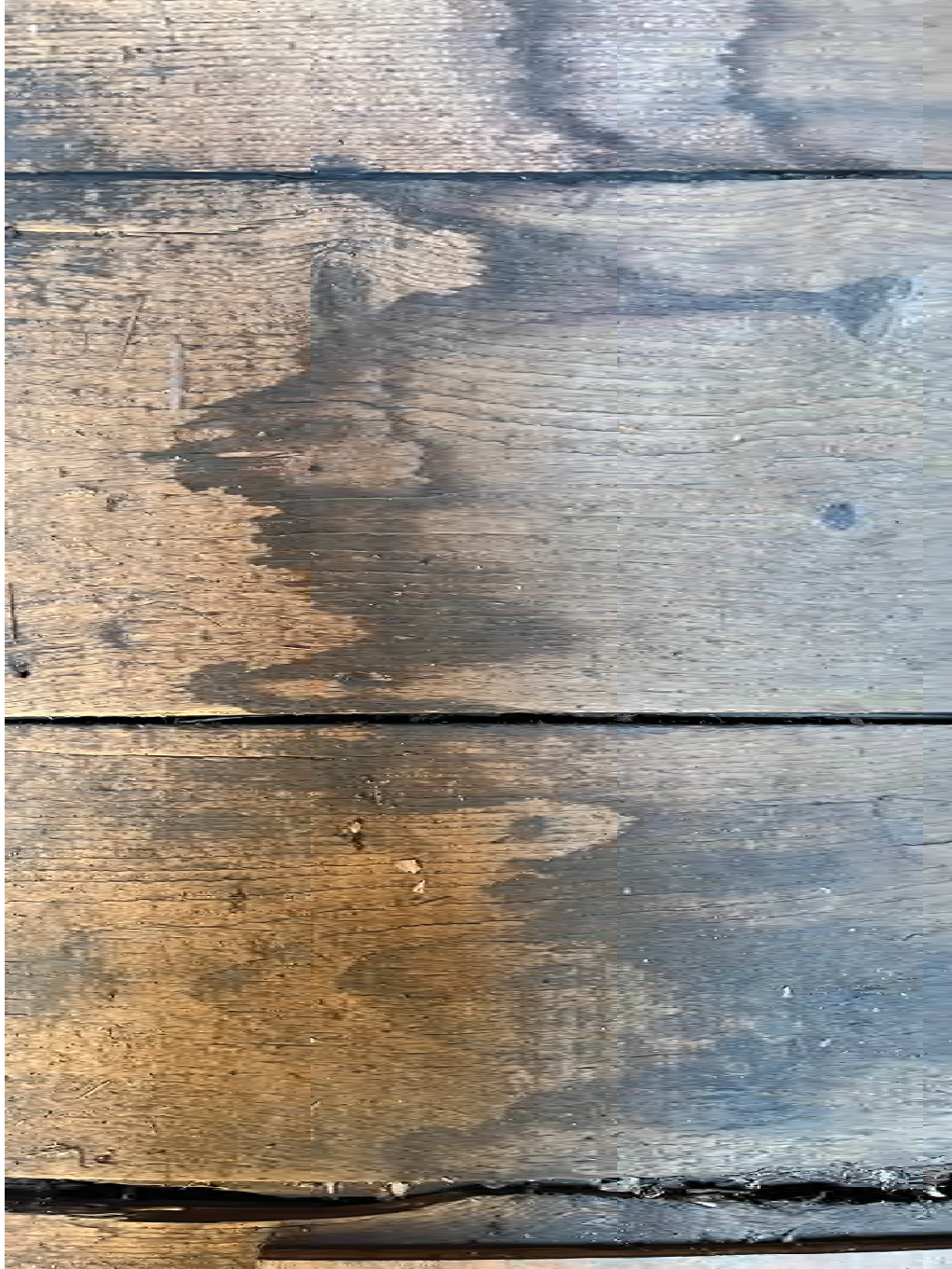
Figure 4.11-8 Splits in the wood were observed in room A-01, as well as evidence of past repairs, where wood has weakened due to water damage.
