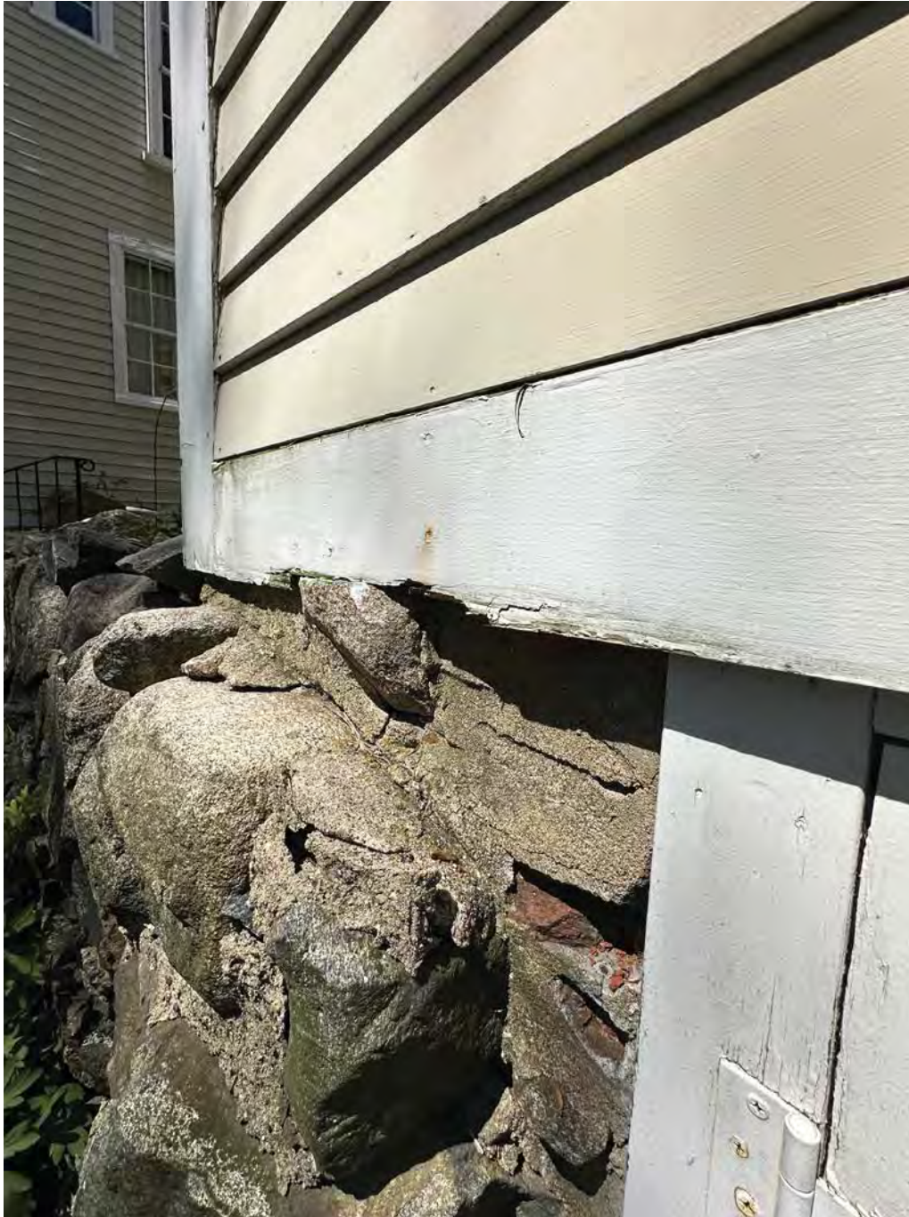
Figure 4.3-6 There is no evident base flashing between the cladding system and the ashlar stone foundation wall.
