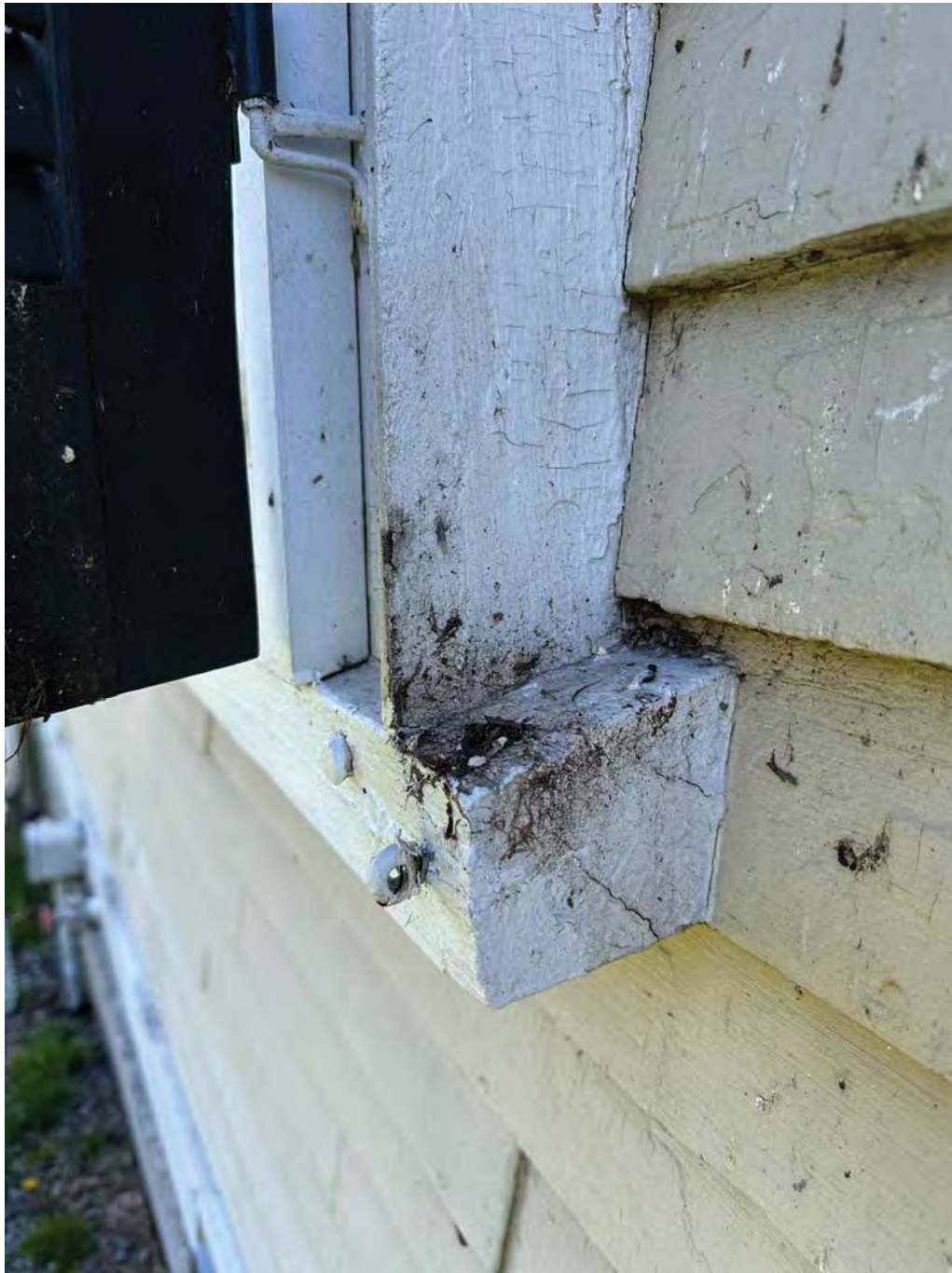
Figure 4.5-4 Evidence of soiling such as dust, dirt and debris piling up. Typical condition seen throughout.
