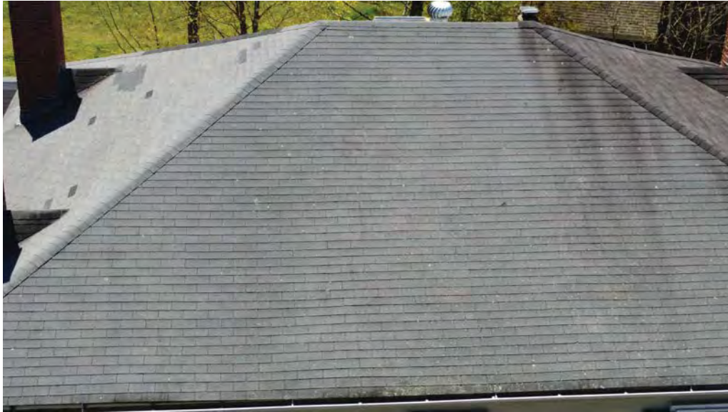
Figure 4.6-4 There are signs of biological growth typical across the entire north slope of the main roof, and edge of the south roof.
