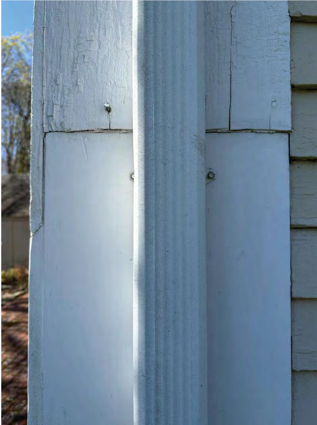
Figure 4.7-5 Downspouts fastened directly to the wooden pilasters with downspout straps installed without spacers at the northwest and northeast corners.
