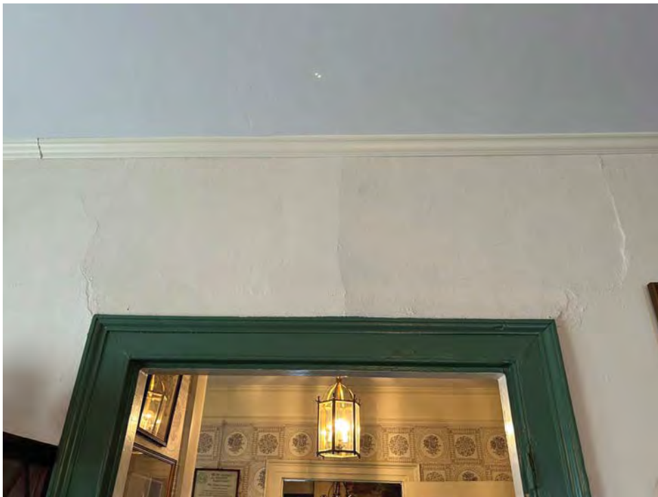
Figure 8.3-16 Diagonal cracking above opening to dining room.
