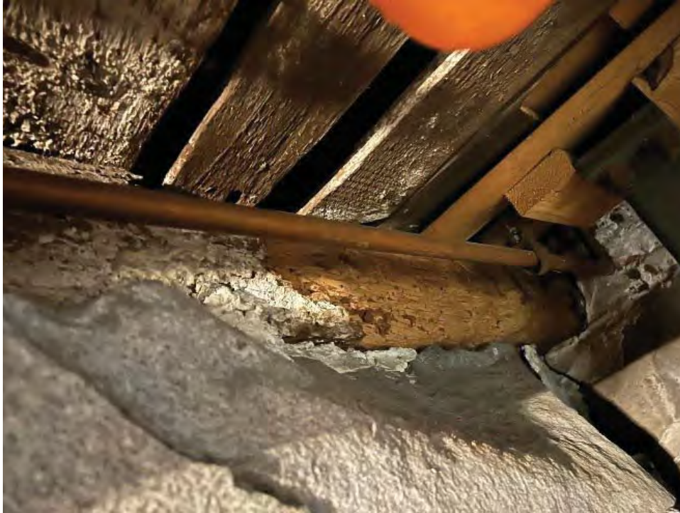
Figure 8.3-5 Deterioration at sill southwest corner.
