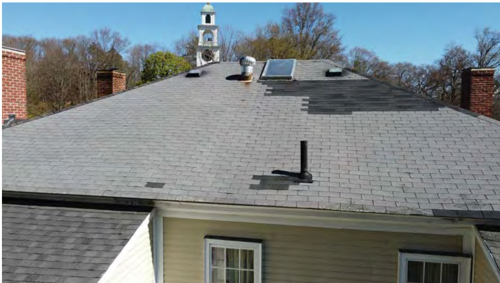
Figure 4.6-5 Selective repairs have been done on a portion of the roof on the south slope, where a large hole was patched.
