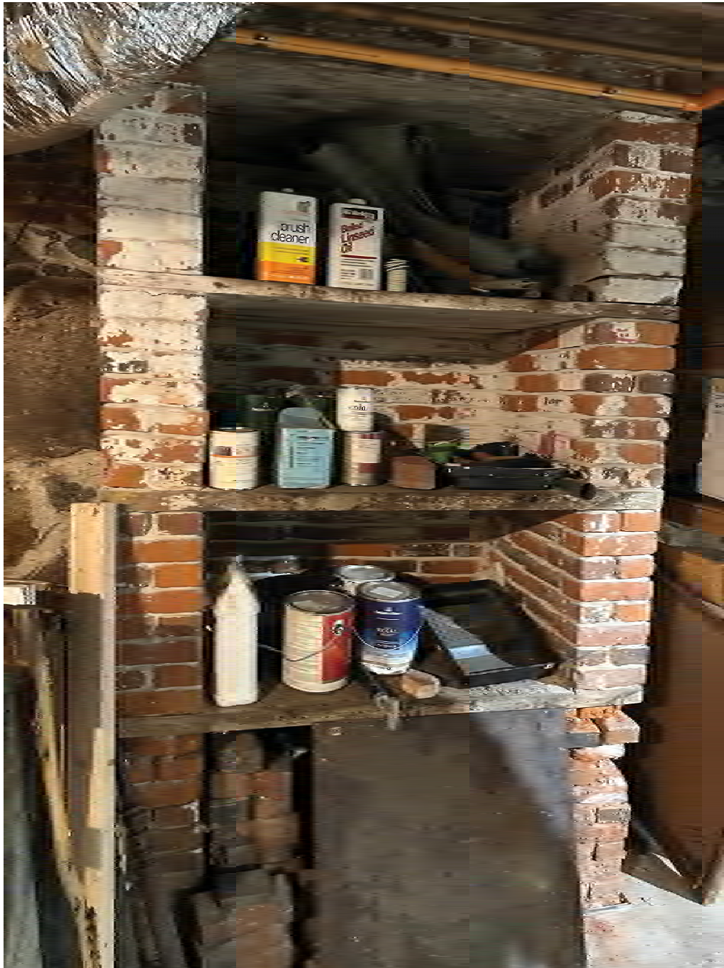
Figure 4.12-3 Fireplaces FP-05 and FP-09, and FP-06 and FP-10 each share a chimneystack with two flutes, with foundations and footings visible in the basement. Visible are cracked bricks, loss of masonry coating and loss of mortar.
