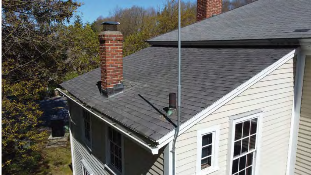
Figure 4.6-8 Both roofs of the additions are in the style of a shed roof, in fair condition.
