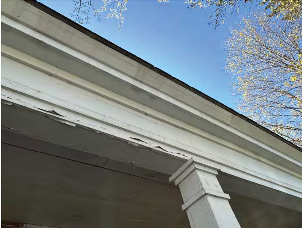
Figure 4.9-8 The frieze board and fascia of the porch roof have as well been replaced.
