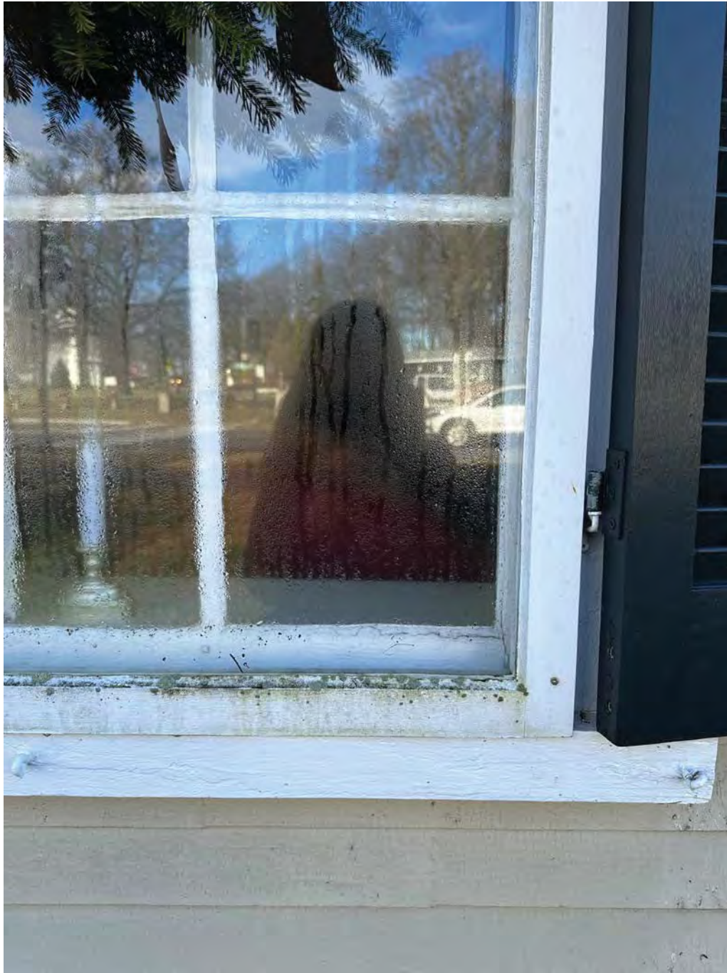
Figure 4.4-11 During the Request for Proposal process in December 2023, condensation was observed between the window and storm window.
