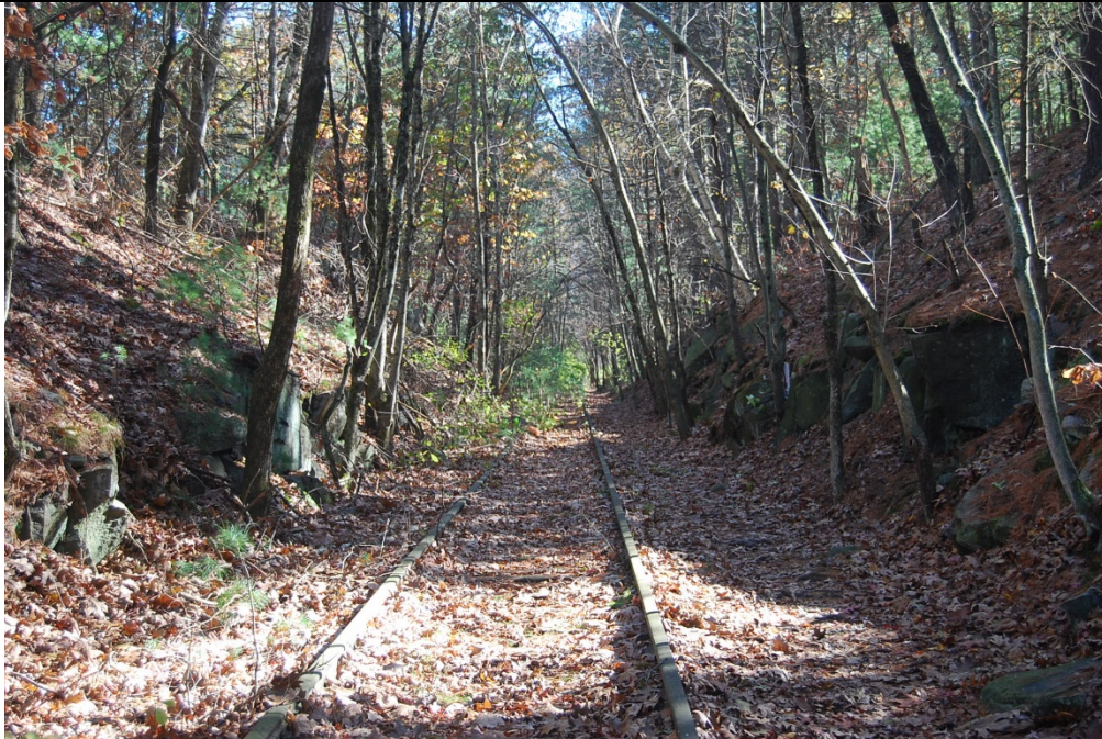
Railbed in stone cut at E side of intersection with Dutton Road. View looking E.
