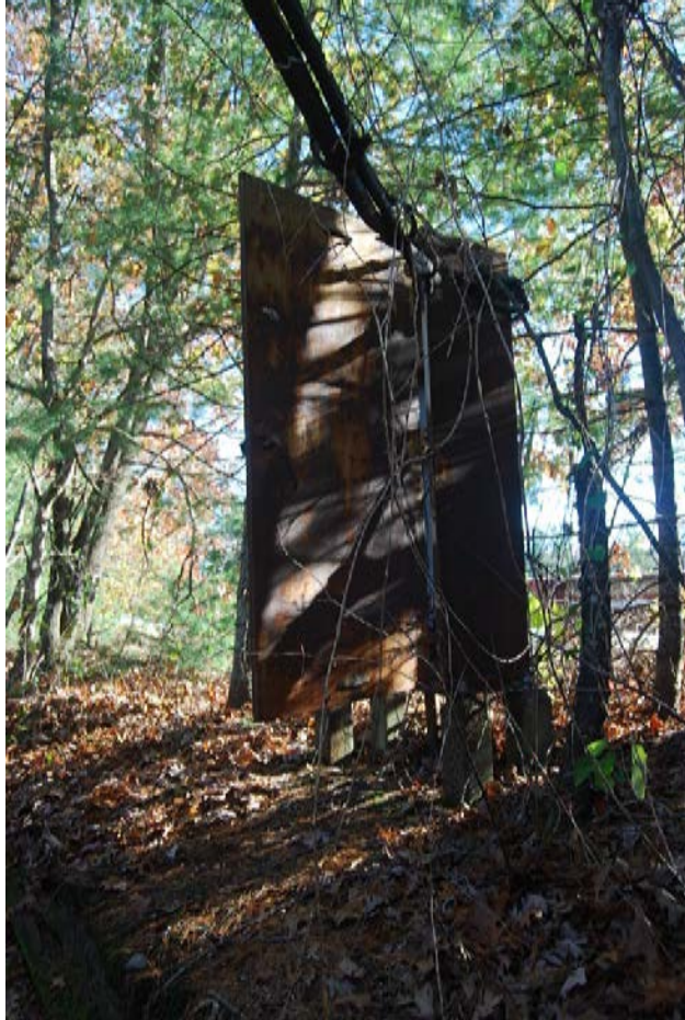
Relay Box at MP 20.59. South side of tracks. View looking SE. Box rests on four cast concrete piers.
