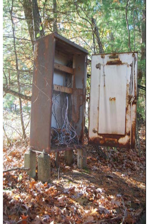
Relay Box at MP 20.59. South side of tracks. View looking SW. Box rests on four cast concrete piers.
