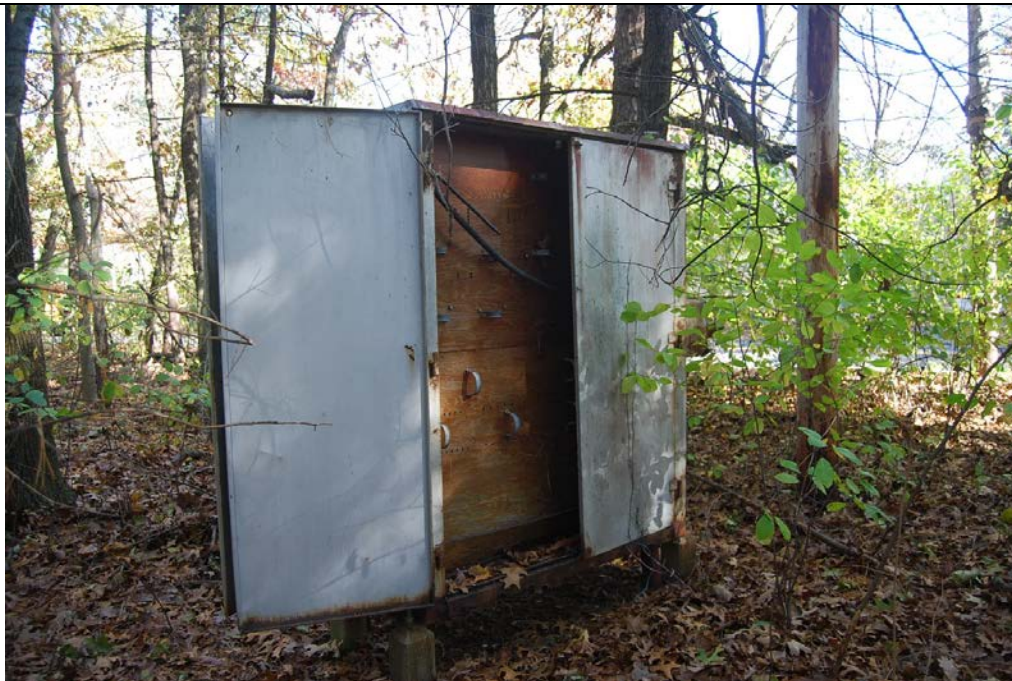
Relay Box at MP 20.79. Horse Pond Road visible through foliage. North side of tracks. View looking northeast. Box rests on four cast concrete piers.
