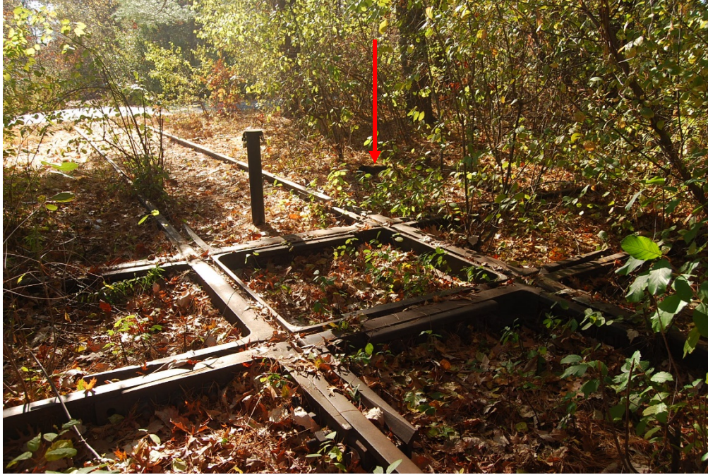
Diamond intersection. View looking SW. Fallen wood post at red arrow.
