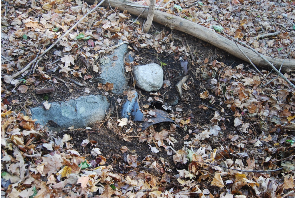
Culvert 127A. South elevation. View looking N. Although culvert has begun to fill in, stone box and cast iron pipe still visible.
