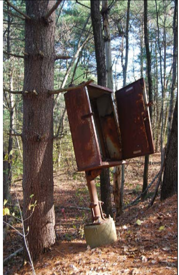
Relay Box at MP 21.16. North side of tracks. View looking northeast. "Candlestick" type.
