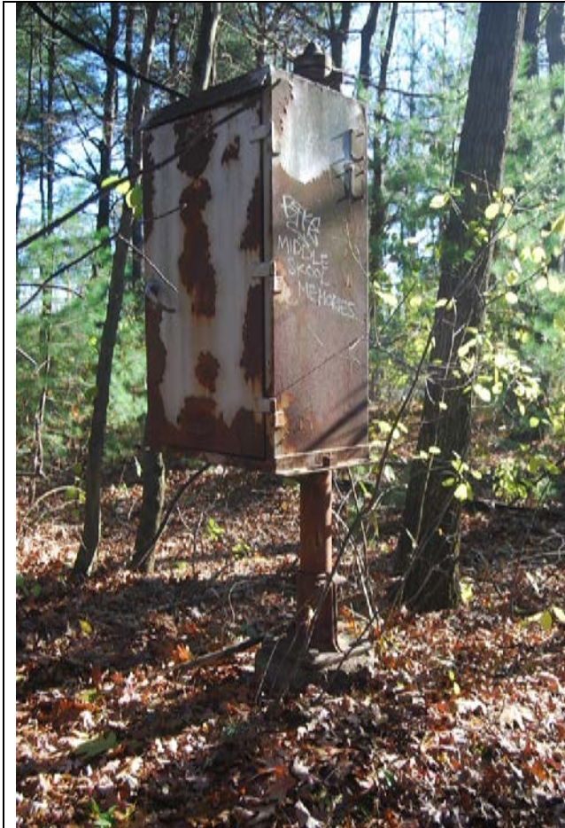
Relay Box at MP 20.07. North side of tracks. View looking NW. "Candlestick" type.
