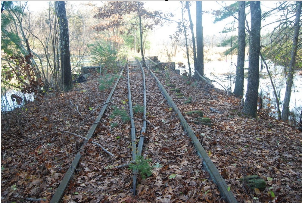
Raised railbed at approach to Bridge 127 at MP 19.47. View looking E.
