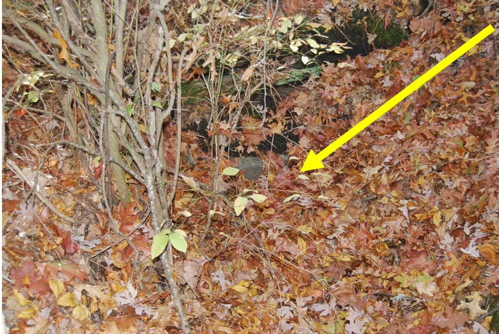
Culvert 127C. South elevation. View looking NW. Stone blocks visible at center photo.
