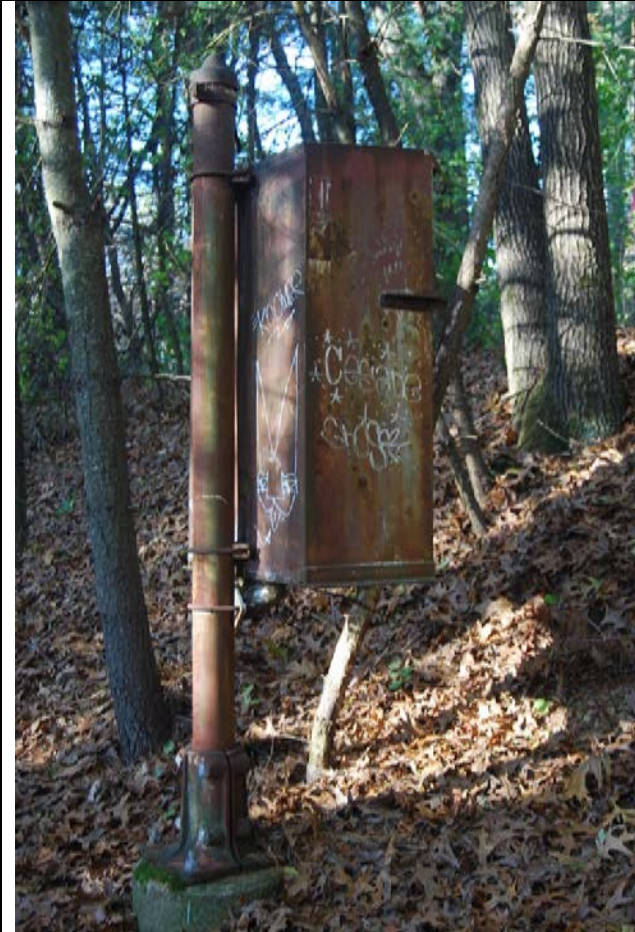
Relay Box at MP 20.59. North side of tracks. View looking northwest. "Candlestick" type.
