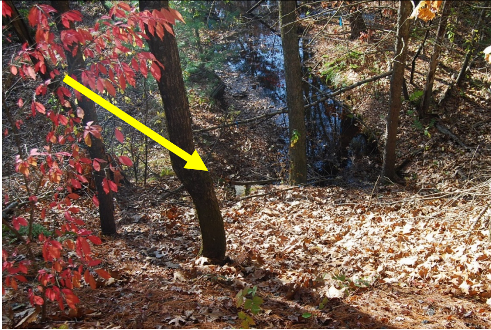
Culvert 127H. North elevation as seen from rail bed. View looking N.
