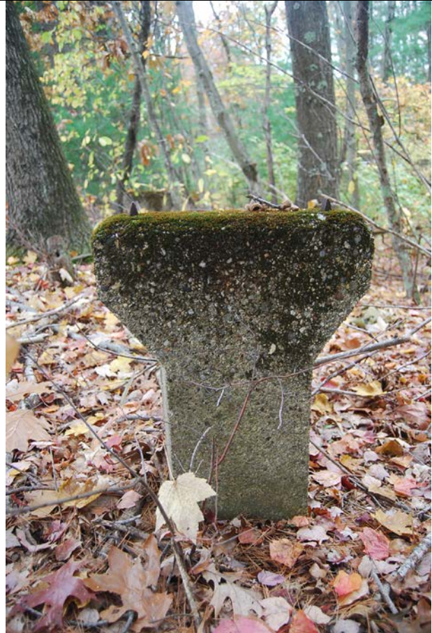
Rail Rest at MP 20.09. Detail, East post. Note inverted spikes at top used to contain rails.
