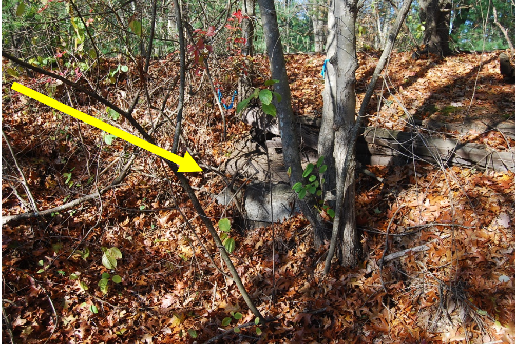
Culvert 127C. North elevation. View looking SE. Stone blocks visible at center photo.
