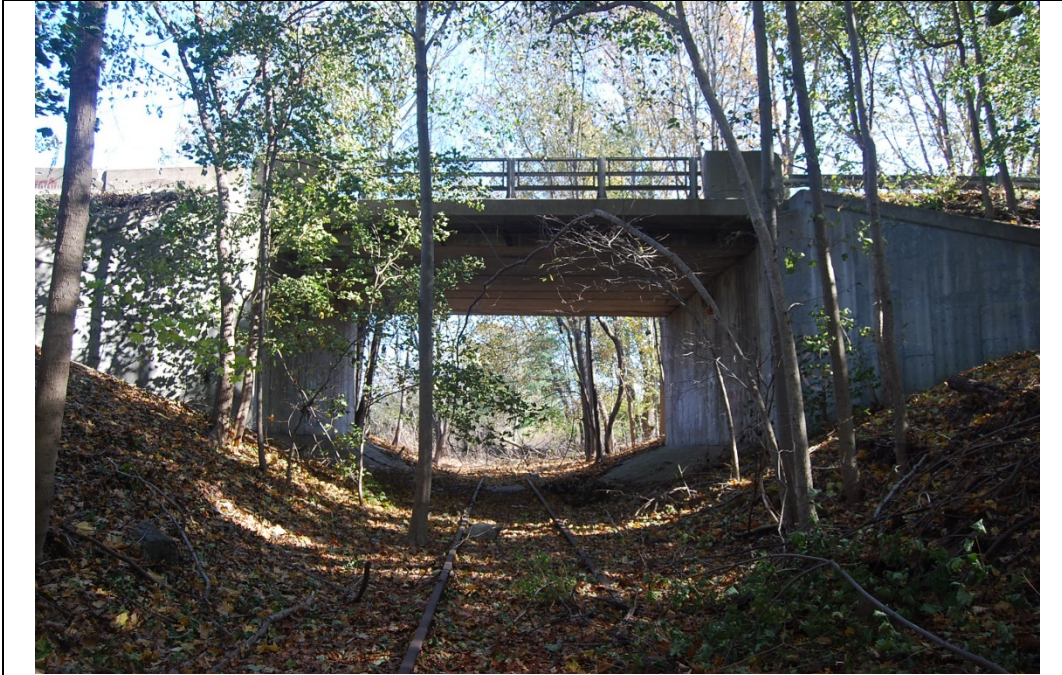
Rail bed in earthen cut near MP 18.86. View looking E toward Landham Road Bridge. Note intact trackage and bed.
