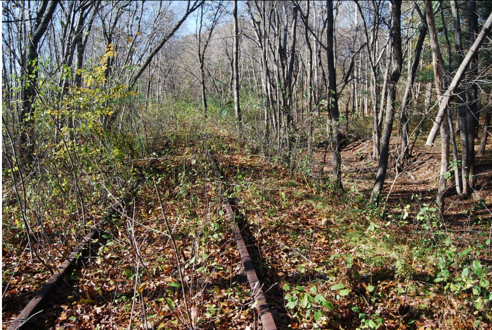
Railbed near MP 19.06, showing raised bed (approx. 15' high) typical to this area. View looking W.
