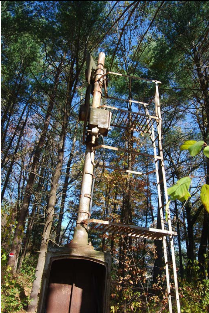
Signal M208 at MP 20.8. View looking N. Ladder detail.
