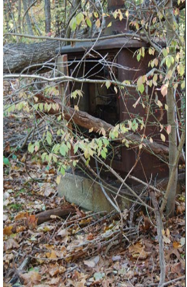
Cabinet detail. Auto Highway Flasher/ Signal Relay Box at MP 21.35 at NE corner of intersection of Peakham Road and ROW. View looking SE.
