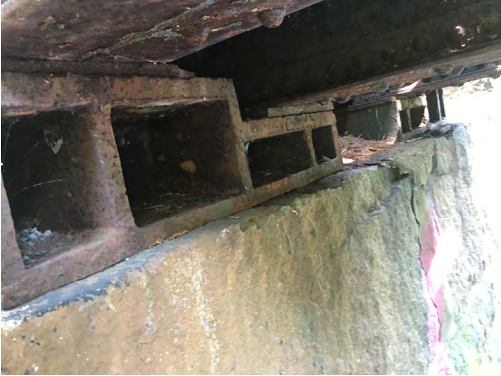
Photo 11: Typical Bearing Assemblies
