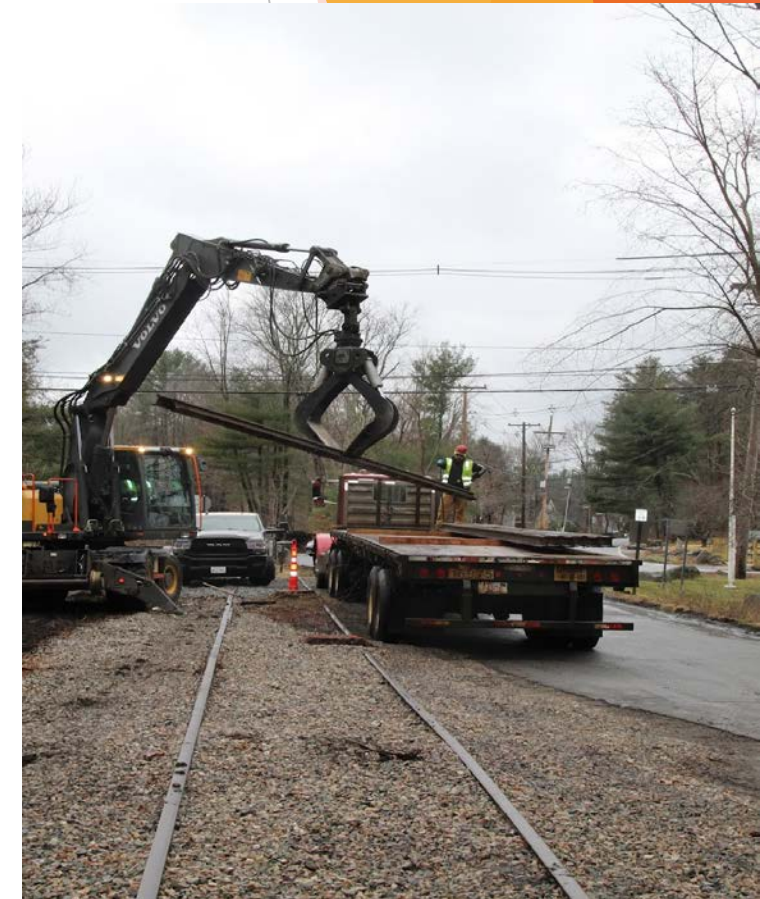
Cutting and stacking rails for the Bruce Freeman Rail Trail at Hudson Road & Peakham Road
