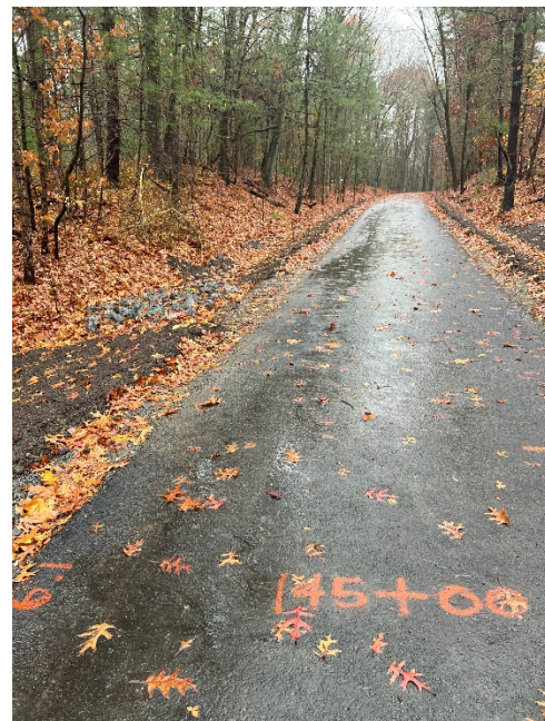
Photo 4: Sta. 145+00 looking north at the swales along both sides of the trail.
