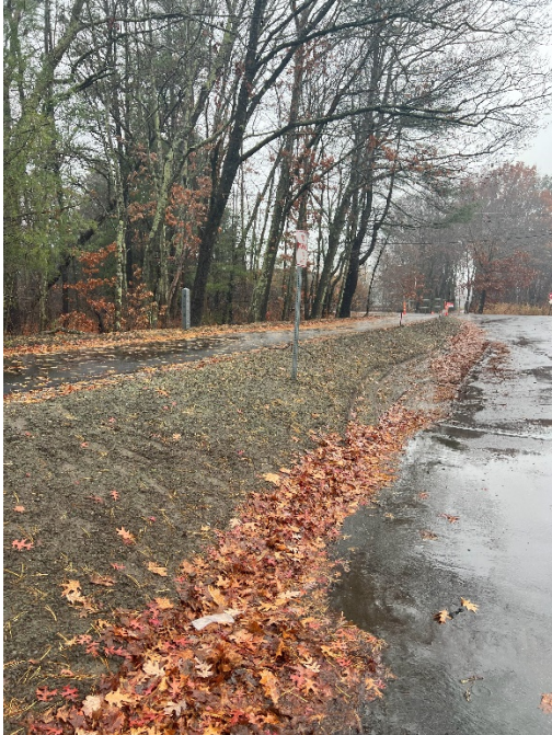
Photo 1: Sta. 107+00 looking north at the formed side slope with loam and seed
