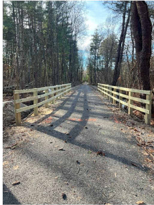
Photo 2: Sta. 167+50 looking south at the timber fencing across the 48" culvert.
