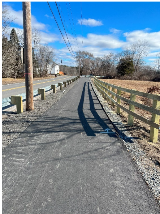
Photo 3: Sta. 1102+00 looking east at the timber fencing along the Davis Field spur path.
