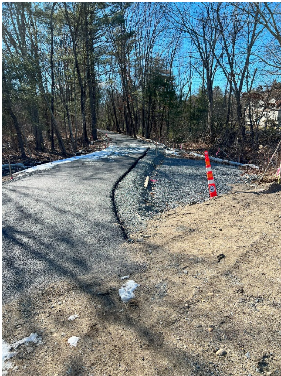
Photo 11: Sta. 307+50 standing at North Road looking south at the trail and proposed rest area.
