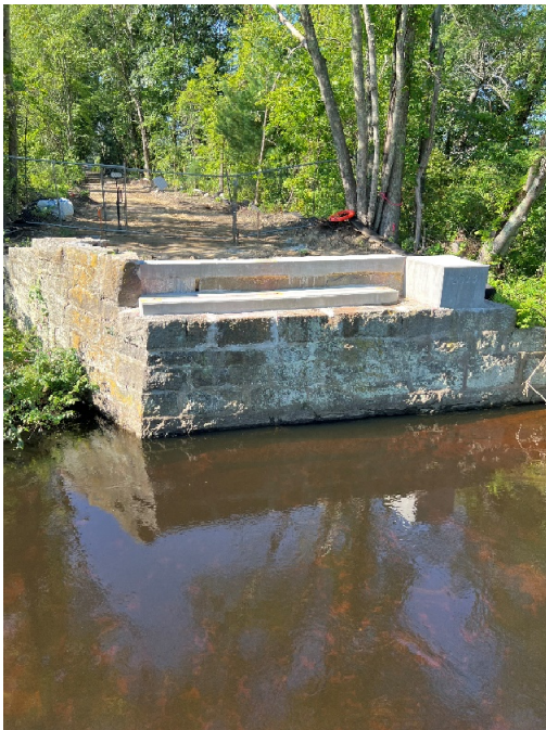
Photo 3: Sta. 126+50 looking south at the southern bridge abutment and backwall cap of the Hop Brook bridge
