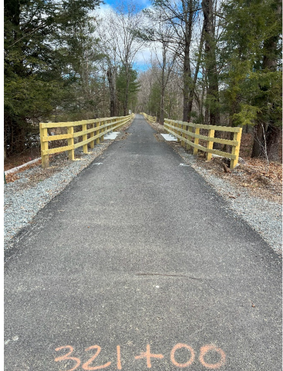
Photo 10: Sta. 321+00 looking north at the fencing across the cattle crossing.
