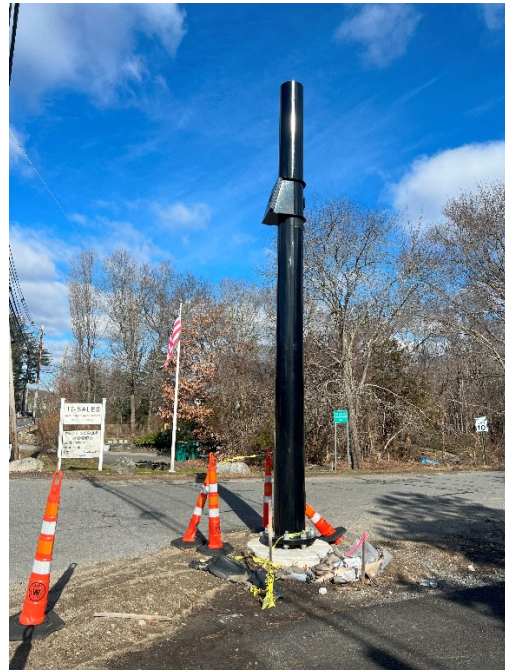
Photo 4: Sta. 175+50 looking at the newly installed mast for the Hudson Rd/Peakham Rd intersection.
