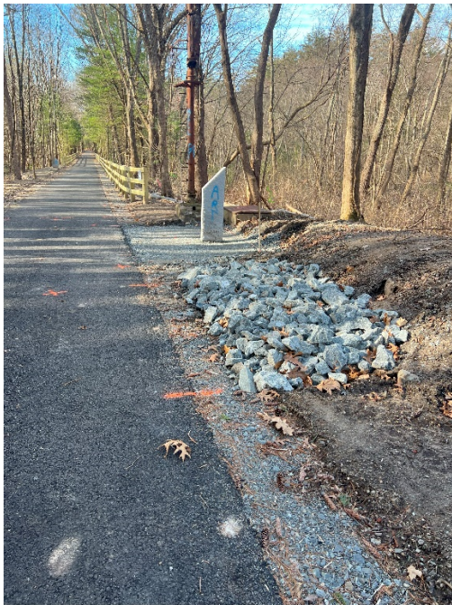
Photo 3: Sta. 163+50 looking south at the proposed rest area and modified rock for swale end.
