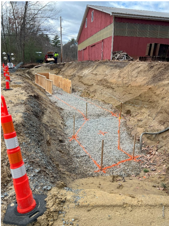
Photo 7: Sta. 217+50 looking south at the retaining wall forms for the Morse Rd rest area.
