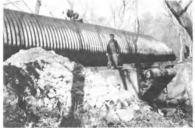
PEAKHAM ROAD bridge was made safer by the installation of a new culvert in November.
